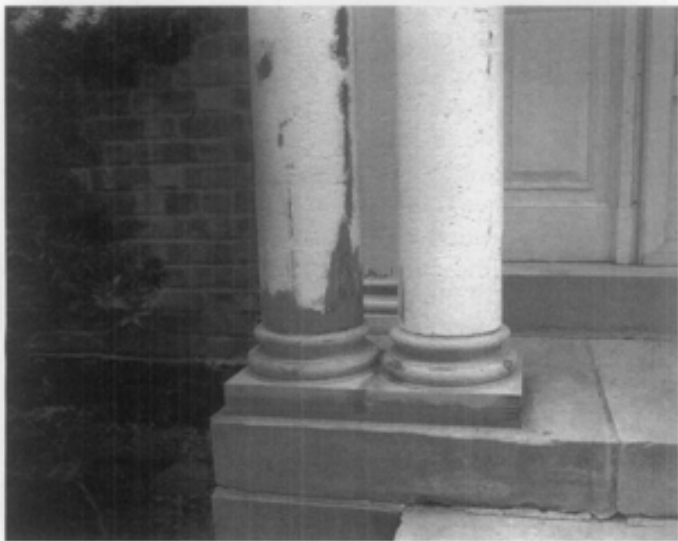
Figure 11. The lower shaft of the porch columns had decayed as water wicked up through the end grain (top). The column shafts were repaired in place by cutting out the deteriorated wood and making repairs using epoxy consolidants and fillers. (bottom). The column bases were replaced. Photos: Paul Marlowe, Marlowe Restorations.
