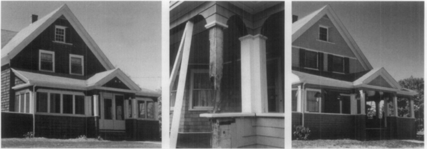
Figure 14. The enclosure of a prominent porch can dramatically change the historic character of a building. The L-shaped porch on this 1896 Shingle-style New England residence was later enclosed with aluminum windows and screens. Recent owners elected to reopen the historic porch. Among the other work, it was necessary to correct structural damage, as with this post, where beneath the wood casing carpenter ants had done serious damage. In reopening the porch, the historic character of the residence has been brought back and the traditional use of the porch is once again enjoyed. Photos: Mark Landry, Landmark Services.
