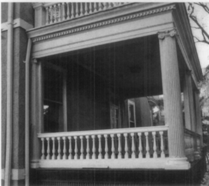
Figure 17. The porch's structural system must be capable of supporting today's loads. In this case moisture led to the deterioration of the wood girder at the corner, creating a major structural deficiency (top). A new solid timber was installed to replace the girder (middle); alternatively a built-up girder could have been used since a fascia board would conceal it. The column base was repaired and portions replaced and the balustrade and column reset and secured (bottom). Photos: Paul Marlowe, Marlowe Restorations.
