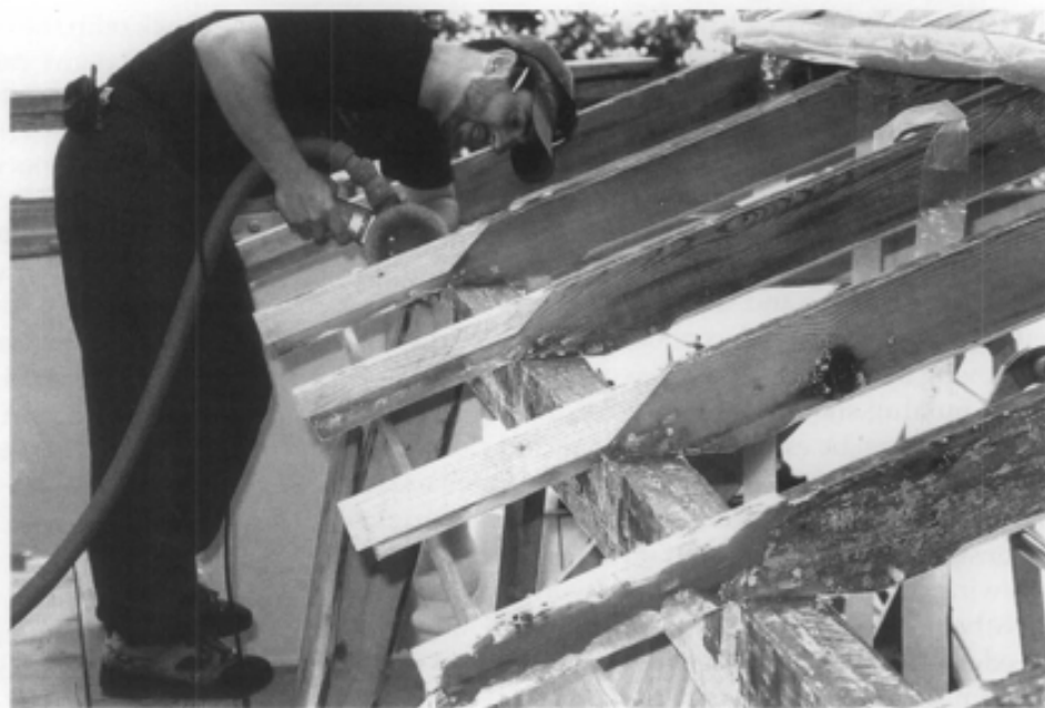
Figure 9. The ends of porch roof rafters are often susceptible to moisture decay. When concealed by a soffit or ceiling, rafters can be repaired by adding new sister boards. Where roof rafter ends are exposed, splicing new wood onto the old (dutchman repair) and use of epoxy consolidants and fillers both preserve sound historic fabric while retaining the historic appearance.
