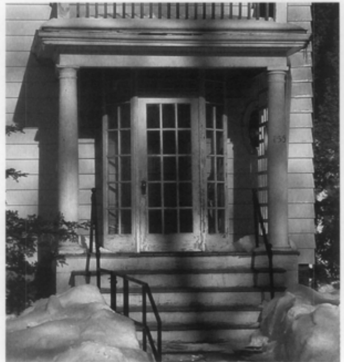
Figure 13. Particularly in New England, there is a cold weather tradition of installing temporary glass and wood panels at entrance doors, thereby creating an enclosed vestibule. These enclosures with their small divided lights were generally removed in the spring.
