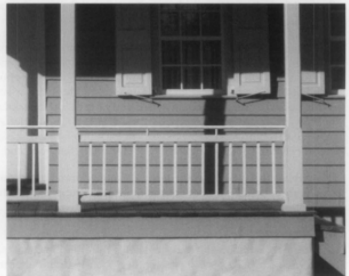
Figure 19. Historic porches generally have railings that measure 28 to 30 inches in height from the floor. When additional height is necessary for safety, a simple rail, added for illustration purposes in this photograph, can usually be installed above the historic railing. Not only does this treatment allow retention of the historic balustrade, but it also has a minimum impact to the appearance of the porch. Photo: Charles Fisher.
