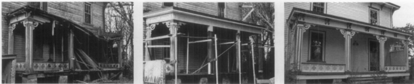
Figure 5. Even historic porches that appear to be in total disrepair may be repairable. While the roof needed replacement, much of this porch was repaired, including such features as the decorative columns, ornamental brackets, and balustrade. Photos: John Leeke.
