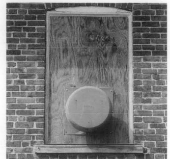
c. The exhaust fan has tamper-proof housing.
