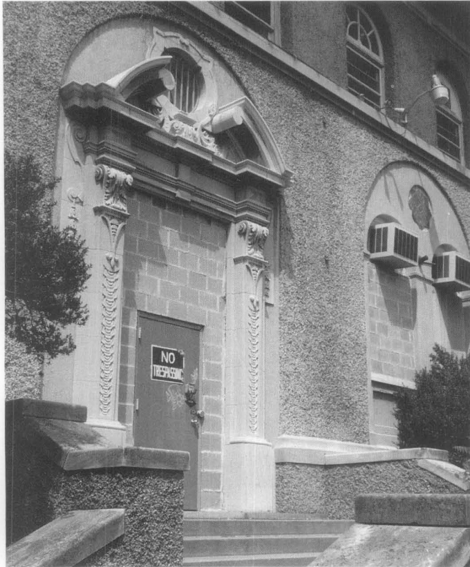
Figure 12. First floor openings have been filled with cinderblocks and doors, window sash and frames have been removed for safe keeping. Note the security light over the windows and the use of a security metal door with heavy duty locks. Photo: H. Ward Jandl, NPS.
