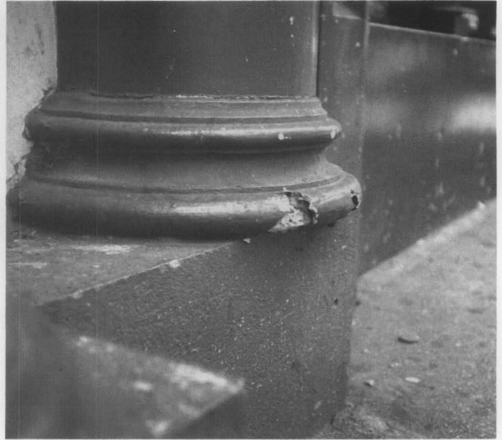
Fig. 20. The location of the feature must be taken into account if a substitute replacement material is being considered. This lightweight fiberglass column at street level sustained damage from impact within a few years of installation. The great strength of cast iron makes it ideal for storefronts and elements that must withstand heavy use. Photo: Building Conservation Associates.
