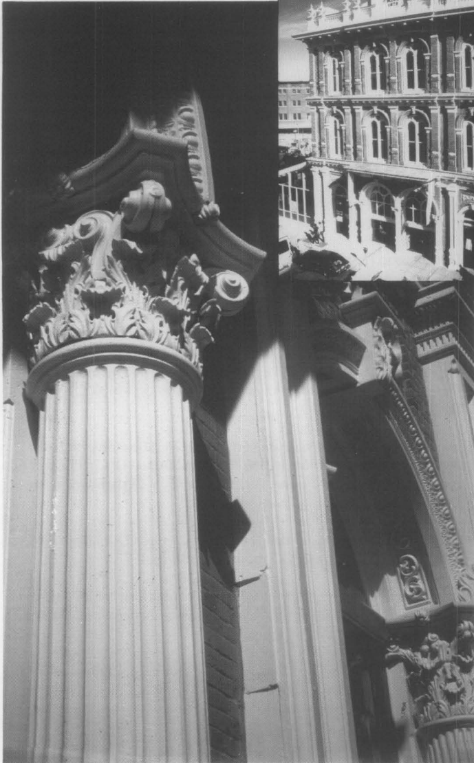
Fig. 19. (a) Fiberglass columns and aluminum capitals were installed to replicate the ornamental features on the east facade of the New Market Theater in Portland, Oregon, that had been destroyed by previous occupants. Like cast iron, crisp ornamental details can be achieved with cast aluminum. Although aluminum may be in contact with fiberglass, galvanic corrosion may result when aluminum is in direct contact with cast iron. Photo: William J. Hawkins, III. (b) The west facade of the theatre retains its original cast iron features. Photo: George McMath.
