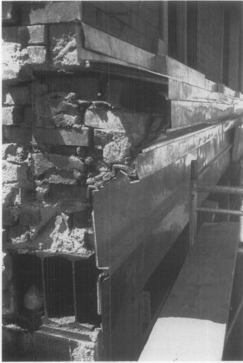
Fig. 18. This cast-iron storefront cornice was corroded beyond the point of repair, and could not be removed easily for replacement. Terne-coated stainless steel, the most durable metal for flashing cast iron, was applied to the cornice and fitted as closely as possible to the historic profile. Although painting is not necessary to protect terne-coated stainless steel, the cornice should be painted to be consistent with the historic character of the building. A primer which is compatible with the terne coating should be used. Photo: Dean Koga, Robert E. Meadows, P.C., Architects.
