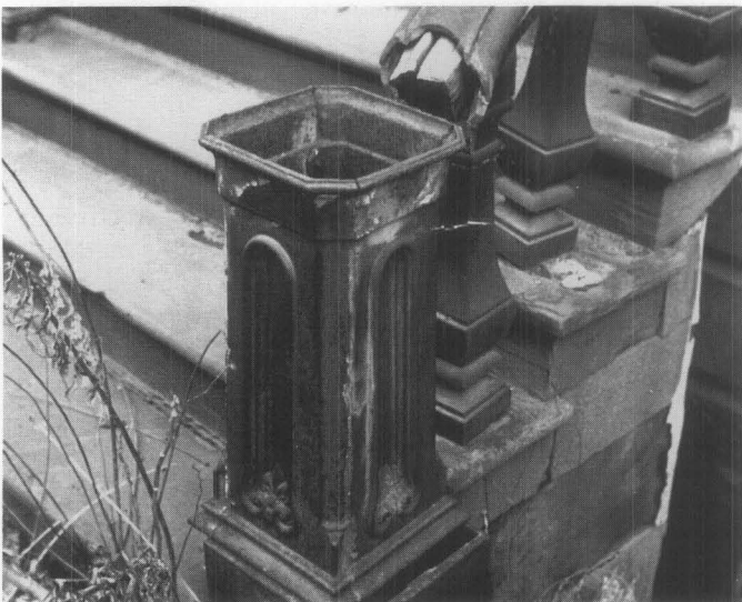
Fig. 15. In an effort to repair this stair railing, concrete was poured around the wood spacer inside the railing casting. Water penetrated the railing and reacted with the concrete to accelerate the corrosion of the iron. Photo: John G. Waite.
