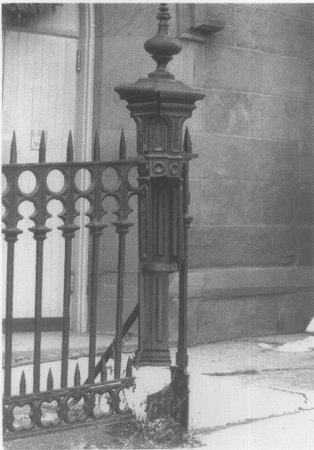
Fig. 7. Despite an impact that shattered the main castings, this fence post remains upright, demonstrating the great strength of cast iron. Originally, the post was held together by a long bolt that extended from the finial to the base. Photo: John G. Waite.
