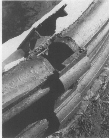
Fig. 9. Galvanic corrosion occurred where a patch of copper was installed alongside the cast-iron cap at the base of a fountain. The use of terne-coated stainless flashings with appropriate caulking would have been a more suitable repair. Photo: John G. Waite.
