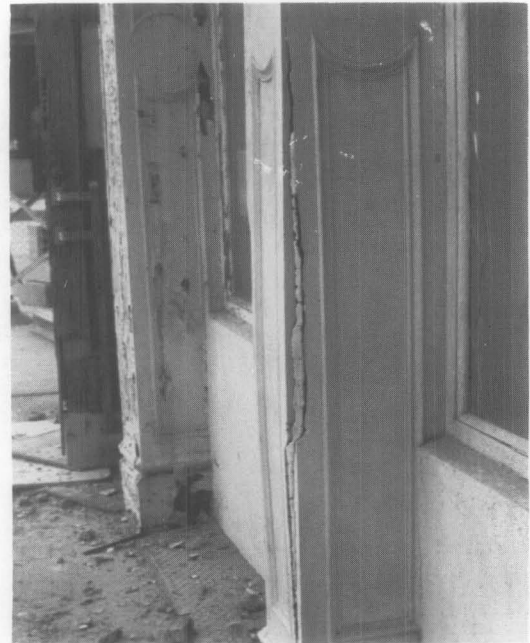
Fig. 11. Major cracks in the piers of this cast-iron storefront in Galveston, Texas resulted from the transfer of load onto the iron from internal brick piers eroded by rising damp. This crack was inappropriately filled with concrete, which trapped moisture and accelerated internal corrosion, pushing the iron further apart. Photo: Ford, Powell & Carson.
