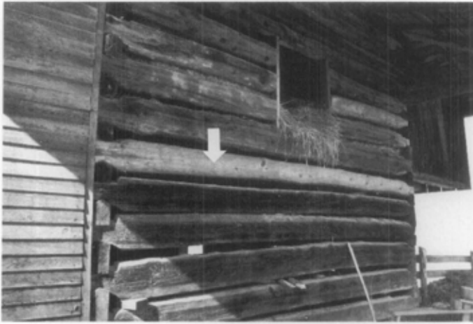
Fig. 22. The lighter-colored replacement log in this barn matches the dimensions and hewing marks of the original logs, and will darken in time to blend visually with the other logs. Photo: Bernard Weisgerber.
