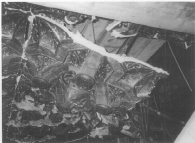
Fig. 21. The Yiddish Arts Theater, New York City, c. 1920s. The concrete roof of this building collapsed, damaging portions of the existing Moorish style coffered ceiling. The square coffer unit was easily identifiable and was removed to a casting shop for reproduction. Photo: David Flaharty.
