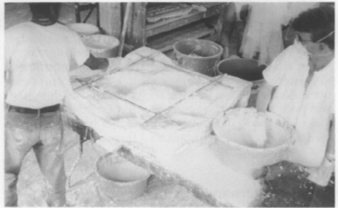
Fig. 8. Casting a Coffering Unit. Ceiling coffers are made the same way today except, historically, a hide glue mold was poured over an ornamental model whereas today urethane molding rubber is used. Now, as then, the plaster casts are made with steel channel irons embedded on the back of each panel. The coffers are hung from carrying irons fixed to the ceiling above by means of twisting wires to level each coffer to its neighbor. Afterward, the panels are fastened together and the joints pointed with plaster. Photo: David Flaharty.
