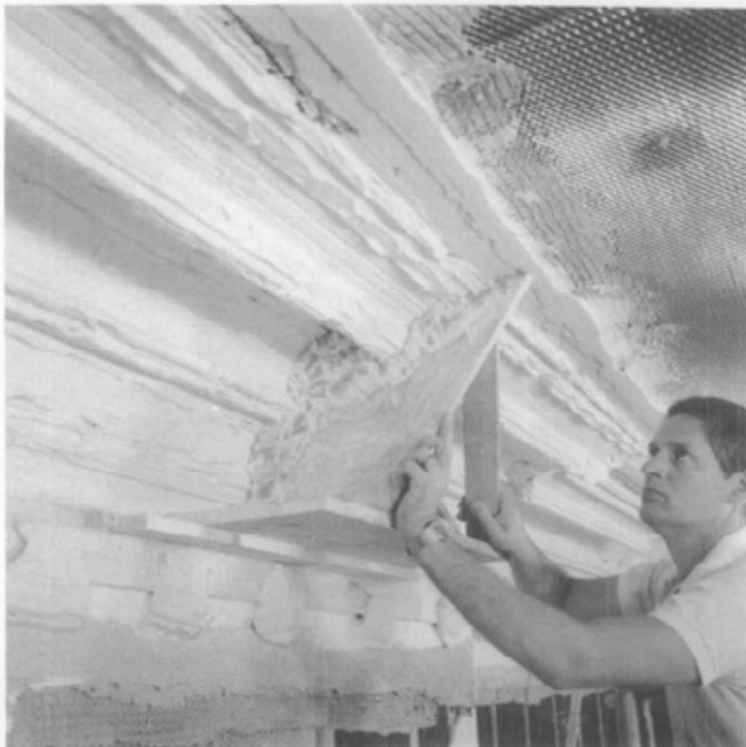
Fig. 4. Running a Cornice. The historic method of producing a cornice is unchanged today. A running mold or template is pushed along a lattice strip nailed to the wall. Base coat plaster is gypsum and sand; finishing plaster is added with small tools and stuffed wearing rubber gloves because lime burns the skin. As many as 20 passes are required to complete a smooth run; this particular cornice was formed in two stages, top and bottom, because it was so large. Cornices this size also have to be blocked and lathed to minimize the amount of applied material. Photo: Old-House Journal.
