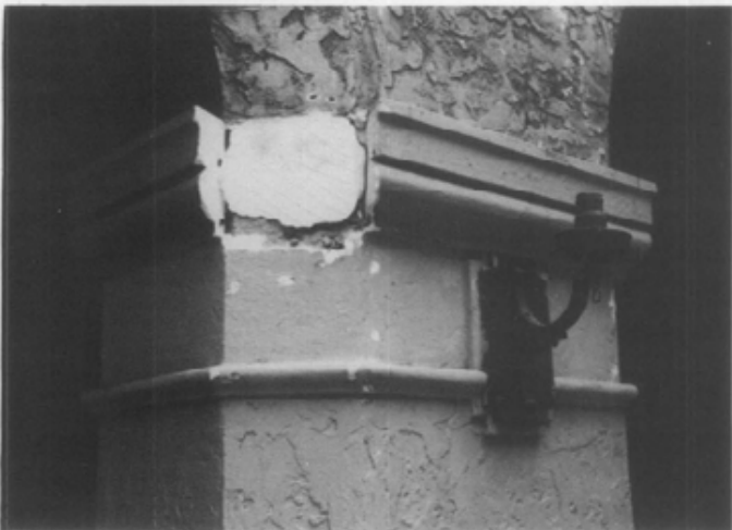
Fig. 14. A mitered portion of this impost capital abacus has fallen, revealing the plaster adhesive material. Repairs are made by obtaining a section through the abacus, making a bench-run length, cutting, fitting, and readhering the missing piece. Finally, the joints are pointed. Photo: Lee H. Nelson, FAIA.
