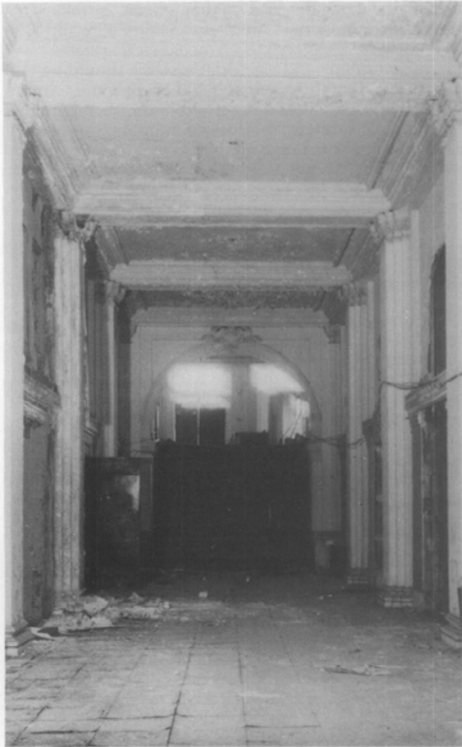
Fig. 13. Water intrusion and freeze/thaw cycles caused extensive efflorescence and ornamental plaster failure. The plaster needed almost total replacement within the rehabilitation project. Photo: Commercial Photographics.
