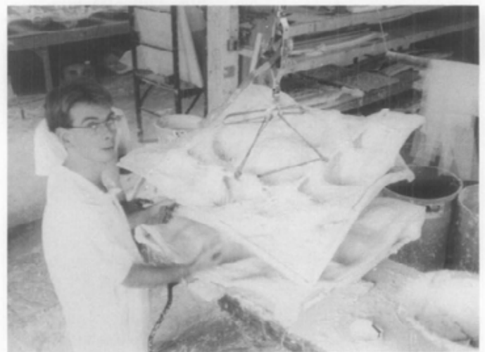
Fig. 22. Repairing a Coffered Ceiling. As part of the theater rehabilitation, the coffered ceiling panels are being reproduced in urethane rubber molds and reinforced with open weave burlap and wood fiber. Steel channel irons can be seen, attached to the backs of the casts. Later, these irons are used to hang the panels from a superstructure at the site. Photo: David Flaharty.
