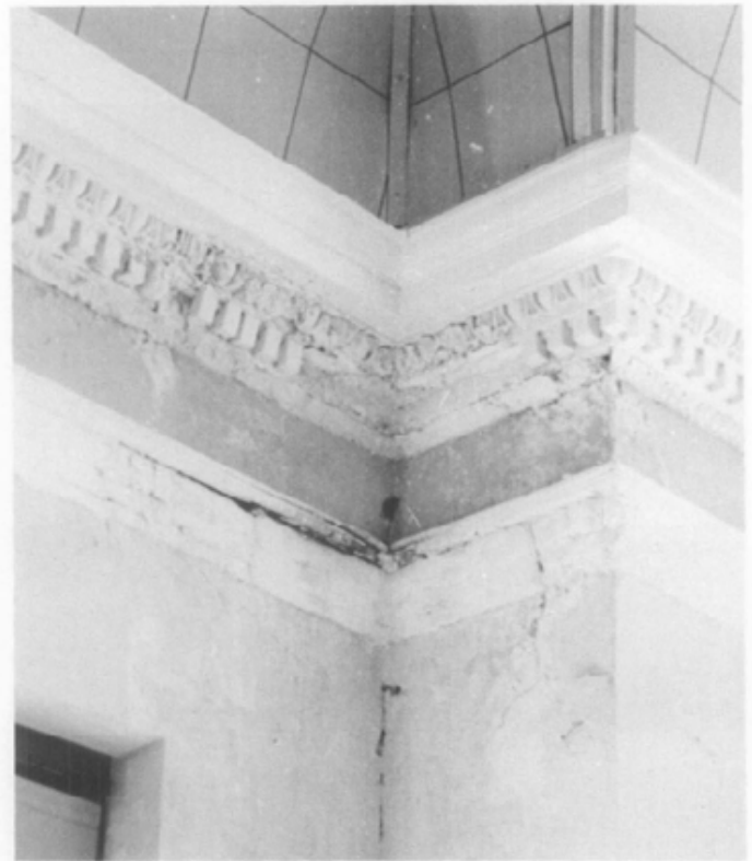
Fig. 11. The cornice of an Iowa courthouse has been severely damaged from a roof leak. In order to repair the ornamental plaster, a thixotropic rubber impression will be taken (with the paint build-up undisturbed). The efflorescence will be removed and fresh plaster casts installed so that egg and dart, dentil and leaf molding are perfectly aligned. Photo: National Park Service files.
