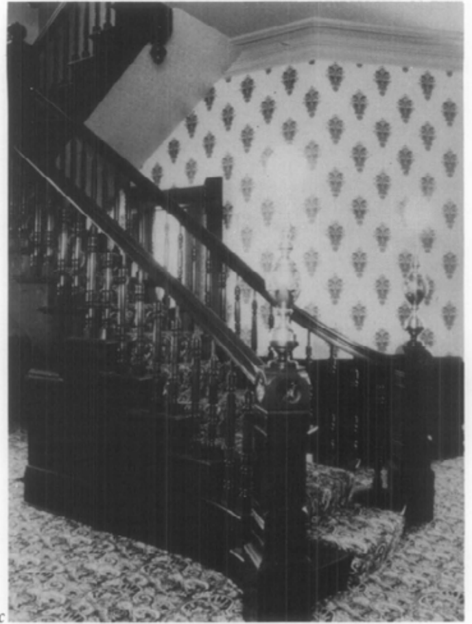
Fig. 18. Repairing a Cornice. (a) In the restoration of the Henry Hirshfeld House, a 19th century residence in Austin, Texas, removal of a tin ceiling revealed a damaged plain-run cornice. Photo: John Volz, AIA. (b) A section through the molding was taken, a template blade cut, horsed-up, and run on a bench using gypsum and lime. Photo: Charles E. Fisher. (c) The new cornice was then cut, fitted, and applied to new blocking between wall and ceiling. The external miter and returns were pointed using the miter rod. After the ceiling restoration was complete, other finishes, such as wallpaper, were applied. Photo: Candace Volz.
