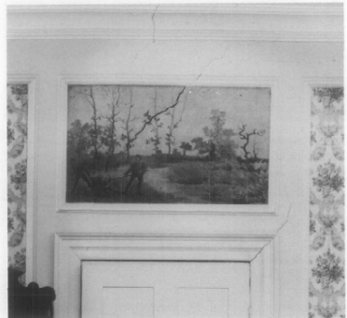
Fig. 12. Settlement caused stress cracking through both flat wall and ornamental plaster. Repairs to the cornice molding involve chamfering the stress cracks to a "V groove" and patching with a mixture of gypsum and lime. The cornice can be countersunk-screwed to its substrate to prevent further movement. Screw heads are then plastered over. The crack running through the painting will need to be filled carefully, and the painting restored by a trained conservator. Photo: Jack E. Boucher, Historic American Buildings Survey.
