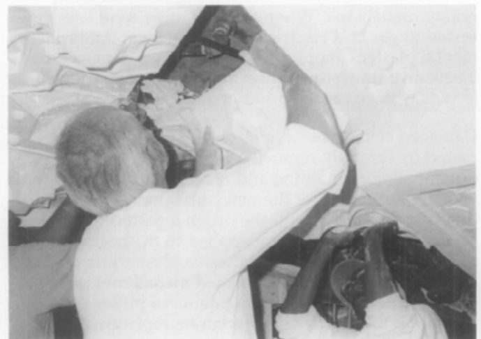
Fig. 23. A pre-cast coffer is lifted into place to abut adjacent panels. Tie wire will be fastened to the channel irons and the superstructure above, twisted to level, and finally wadded with wood fiber soaked in plaster to prevent the wire from stretching. Photo: David Flaharty.
