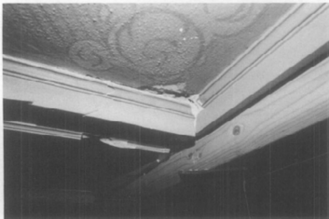
Fig. 10. Structural settling has caused this ceiling to deflect. Prior to restoring the damaged plaster and final repainting, a structural engineer experienced in historic preservation will be engaged to shore-up the ceiling from below and reattach the sagging ceiling plaster with the joists above (see also Fig. 17 under Immediate Action.) Photo: National Park Service files.
