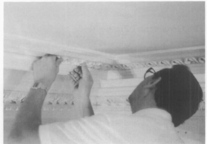
Fig. 6. Enriching a Plain-Run Cornice. After a cornice is run and mitered, cast enrichments are stuck in recessed sinkages planned to receive the casts. Ornamental models are made to engage with one another, resulting in unbroken lines or courses. A shop-cast ornament is soaked in water until saturated and pressed into its sinkage using wet plaster as an adhesive. Once the casts have been installed, they are carefully pointed at the joints and at the miters so that they appear as a continuous, repetitive design. Photo: Old-House Journal.
