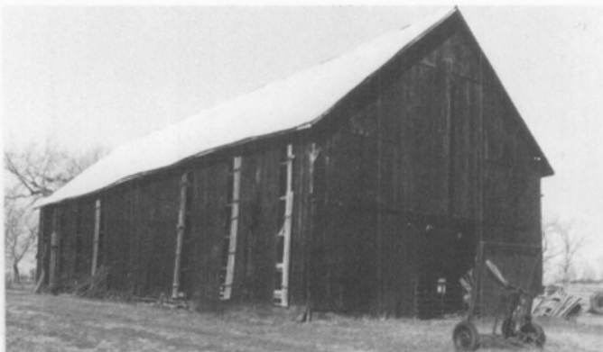
Panels on this 1900 Kentucky tobacco barn open to aid in the curing process. Photo: Christine Amos, Kentucky Heritage Council.
