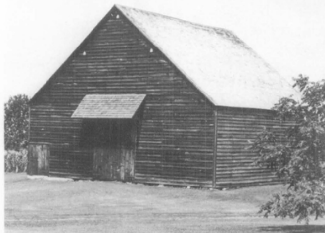
Built in the late 1700s, this New York Dutch barn survives in excellent condition. Gable roof, center wagon doors with pent roof, stock door at the corner and horizontal clapboarding are all typical features of the Dutch barn. Three holes for martins, traditional features of Dutch barns, can be seen near the top of the facade (they have been plugged and are lighter than the surrounding clapboards). Photo: Clarke Blair.
