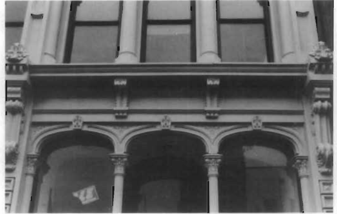
Figure 178. Aluminum Replacement of Minor Structural Elements of a Facade. For minor structural members without great loads, aluminum can be used as a substitute material; however, the capacity of a cast-aluminum column must be designed or checked by a structural engineer and not just assumed to be adequate. When the Grand Opera House in Wilmington, Delaware, was restored, missing cast-iron columns on the first-floor storefronts (flanking center bay entrance, lower center of photograph) were cast in aluminum to match the missing pieces of the original cast iron. (John G. Waite)
