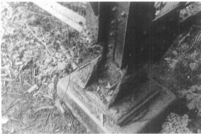
Figure 158. Advanced Corrosion of Rolled Iron. This column base of a New York Central Railroad pedestrian overpass has not been well maintained and has rusted beyond repair. Such exposed ironwork should be painted regularly to keep it from contact with air and moisture. Note the characteristic way that wrought-iron rust exfoliates, or flakes off in layers. (John G. Waite)
