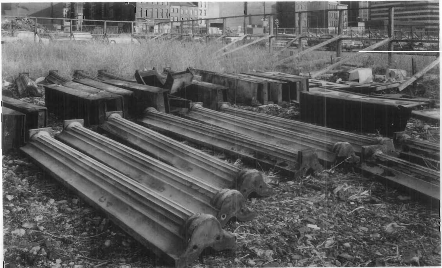
Figure 168. Dismantled Cast-Iron Facades. The Edgar Laing Stores in New York City were erected by James Bogardus in 1849 and had one of the earliest cast-iron facades. The building was demolished in 1971 for an urban renewal project, but its cast-iron facade was carefully dismantled so it could be reerected on another site at a later date. Unfortunately, while the components were in storage, most of them were stolen and apparently sold for scrap. Dismantling of a building should be considered a measure of last resort, to be attempted after all other efforts to save a building in situ have failed. (Jack E. Boucher)
