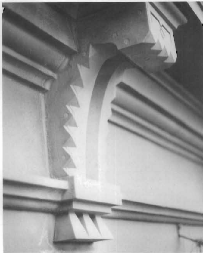
Figure 164. Exposure of Connections and Joints. After the Wilmington Opera House was sandblasted, screw and bolt holes were visible. A cast-iron bracket such as this one may be made of as many as 10 pieces. (Steven T. Baird, AIA)
