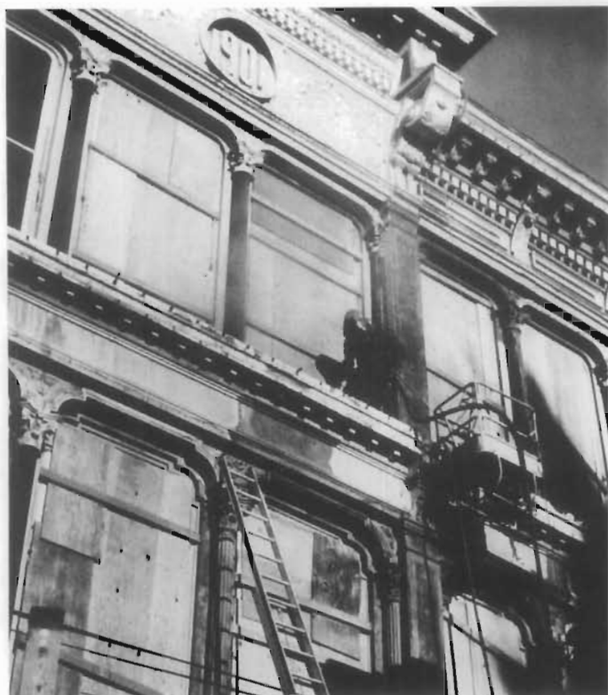
Figure 163. Cleaning Cast Iron. The facade of the Zions Cooperative Mercantile Institute (ZCMI) Store was sandblasted to locate the screws and bolt connections and thereby discover the method of assembly and disassembly. The cast iron should not be heavily sandblasted (down to the bare metal) unless that entire section of the facade is being dismantled. As pieces are being removed, they should be primed immediately to avoid rusting. If the building is not to be dismantled, it is best to remove only the loose paint with a wire brush, being careful not to damage caulked joints and connection holes. Any bare cast iron should be spot primed. (Steven T. Baird, AIA)
