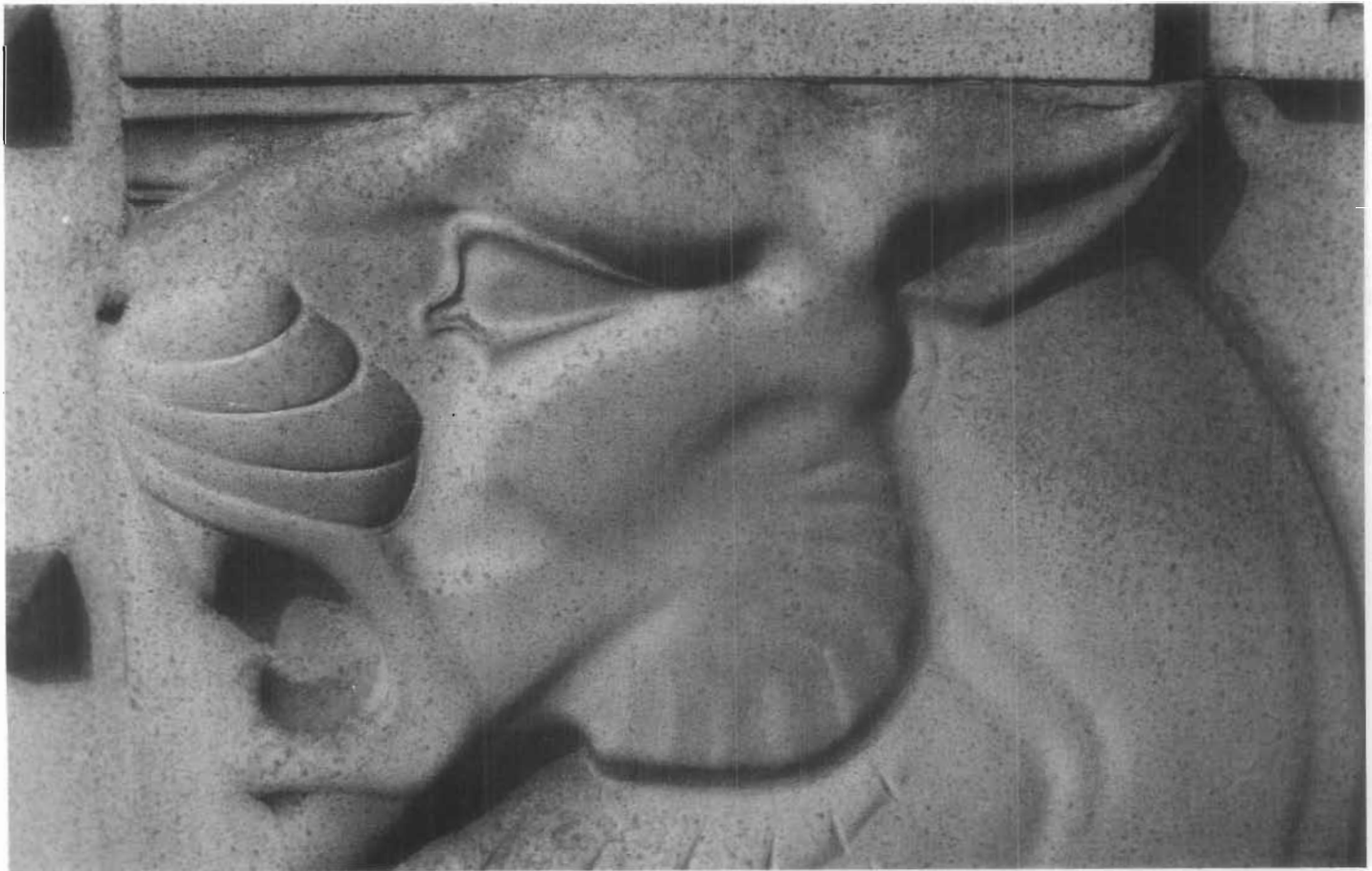
Figure 181. Corrosion and Pitting of Aluminum. Designed by Carl Paul Jennewein, these cast-aluminum doors on the U.S. Justice Building in Washington, D.C., are pitted (see figure 114). Aluminum corrosion is white; however, surface dirt, grime, and pollution have collected on the corrosion products, forming small dark bumps. The pits are actually beneath the bumps and were formed as surface metal oxidized. Pitting is caused by a difference in potential of two or more points on the surface of the same metal and a local breakdown of the protective oxide film. It is encouraged by foreign particles, such as dirt and chlorides which hold moisture next to the surface. (David W. Look)
