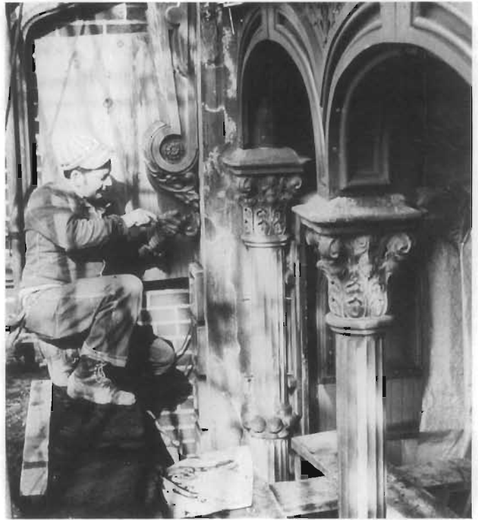
Figure 174. Erection of Cast-Iron Facade. To assemble the Main Street shop facade of the Wilmington Grand Opera House, many assembled sections and individual pieces were shipped to the job site where they were screwed and bolted together in their final positions. (Steven T. Baird)
