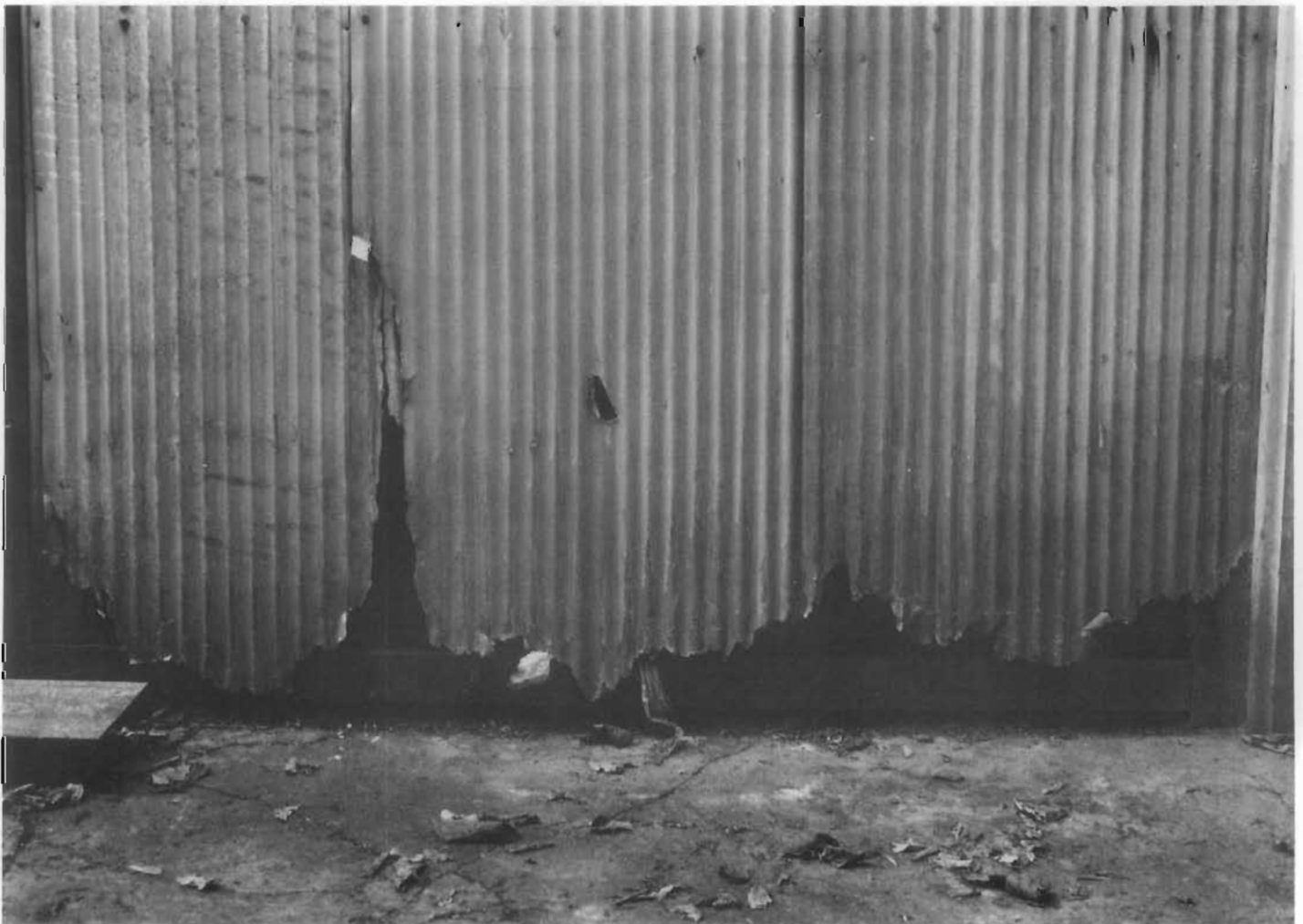
Figure 182. Corrosion and Severe Deterioration of Aluminum. The corrugated aluminum siding on a commercial building in Green Island, New York, has been severely deteriorated by the splashing of water and snow-melting salts. (John G. Waite)
