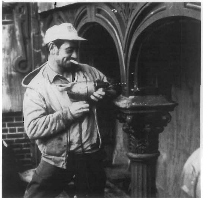
Figure 175. Drilling Holes. Originally, screw and bolt holes were cast into the pieces of iron for new ironwork; however, for the restoration of existing cast-iron facades which may have settled over the years, the holes are sometimes drilled into the replacement parts at the job site to insure correct alignment. (Walter Smalling, Jr.)
