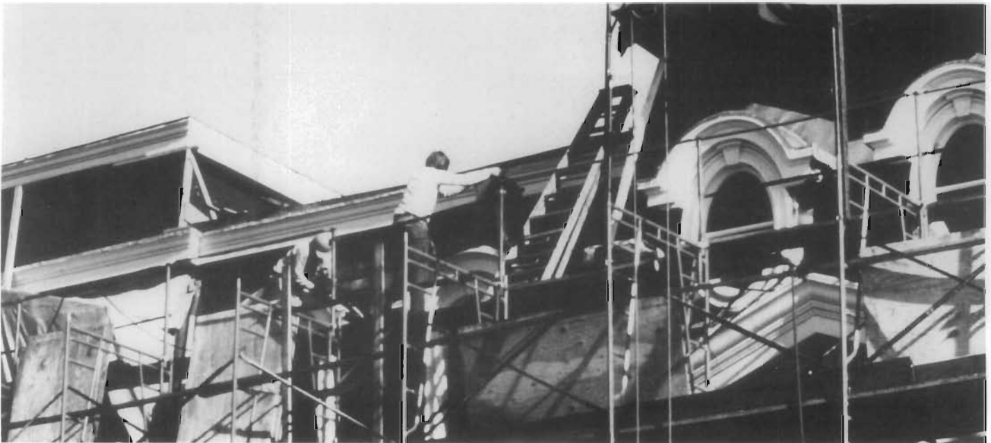
Figure 179. Use of Both Cast Aluminum and Fiberglass as Substitute Materials. After the Mansard roof and dormers of the Wilmington Grand Opera House were destroyed by fire the top floor was rebuilt, but not according to the original design. During restoration of the facade, photographs showing the original Mansard roof and dormers were found, which enabled the re-creation of the missing parts of the facade. The oval windows were cast in aluminum; but the moldings and trim, which may have originally been sheet iron, were made of reinforced polyester. (Walter Smalling, Jr.)
