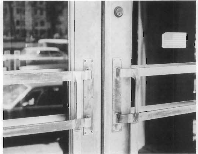
Figure 156. Oxidation of Monel. These exterior doors on the Headquarters of the United Mine Workers of America in Washington, D.C., have a greenish-brown patina of oxidation and an accumulation of dirt and fingerprints. Although the patina is protective, it is not attractive, and detracts from the overall appearance of the building. The push bars are brass with chrome plating which has worn through. To restore the doors to their original appearance, they should be cleaned and polished; and the push bars should be removed, cleaned, polished, replated, and reinstalled. (David W. Look)
