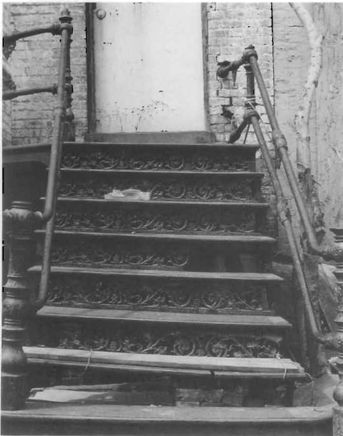
Figure 166. Damaged Cast Iron. This cast-iron perforated stoop in the 700 block of I Street, NW, in Washington, D.C., has fractured in several places because of differential settlement. As the right side of the stairs sank into the ground, the weight of the stoop was redistributed and induced shear, tensile, and torsion forces that were too great for the cast iron to resist. Differential settlement can also be caused by the upward and outward growth of a tree adjacent to a stoop and the downward settlement of a dead tree stump as it decays. No patching or repair work will be effective until the problem is corrected. The stoop should be disassembled and a new concrete foundation poured; the stoop can then be reassembled using welded fractured pieces and recast missing pieces. (David W. Look)
