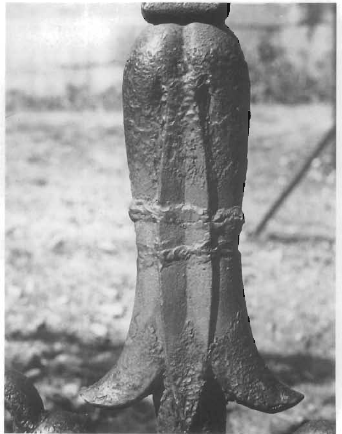
Figure 167. Welding Cast Iron. Although cast iron is very difficult to weld, it can be done by a skilled welder. This is a detail of a weld on the cast-iron fence at the Gardiner-Pingree House in Salem, Massachusetts. "Ni-Rods" welding electrodes, made with a nickel alloy, have been used to weld cast iron since 1947. This weld should have been ground down after completion. (Lee H. Nelson)
