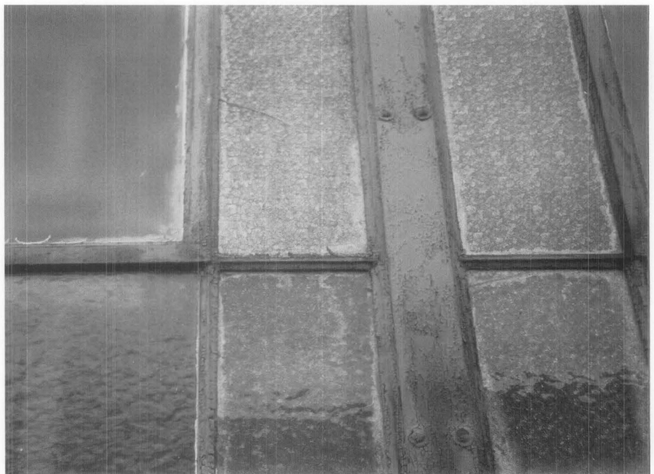
Figure 2. Narrow sightlines, ventilator weathering flanges and mullion boltheads were all distinguishing features of the original steel windows. Photo: Bruner/Cott & Assoc., Inc.
