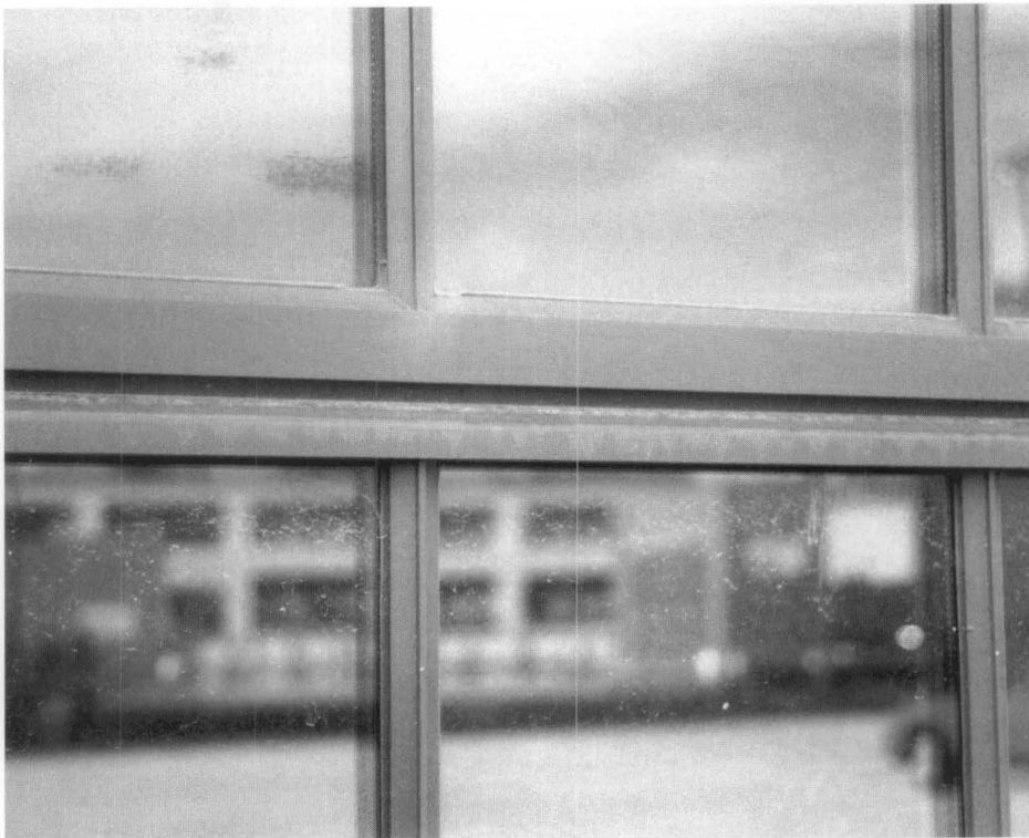
Figure 8. A close up view of the replacement window showing the replicated ventilator drip cap and narrow muntins. Photo: Bruner/Cott & Assoc., Inc.
