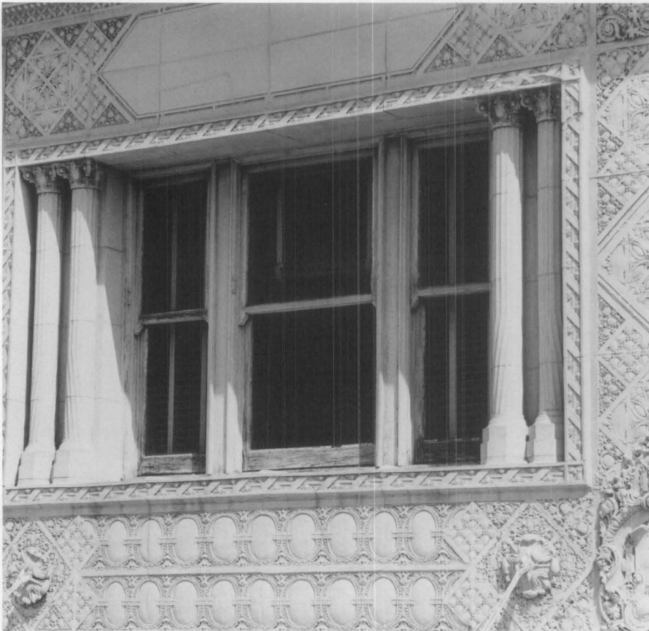
Figure 1. Deeply recessed windows with ornamental terra-cotta surrounds were character-defining features of the building which the owner wanted to retain. Photo: Jack Graves, AIA
