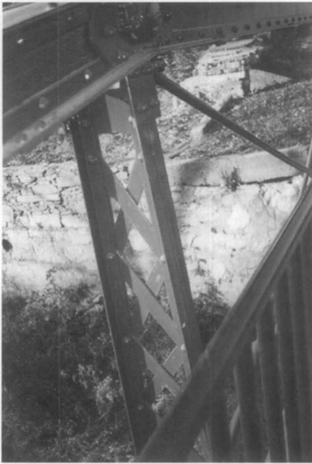
Figure 10. The new lattice girders are shown as installed on the bridge. Photo: Joseph P. Saldibar, III.
