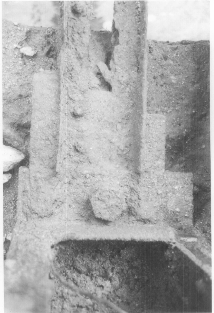
Figures 2 and 3. The extent of damage can be seen in the bent vertical post member (below, left) and the heavily corroded end post (right). Similar problems existed throughout the structure. Photo: Beta Engineering.
