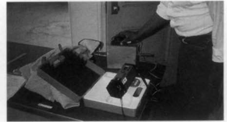
Fig. 7. This electromagnetic detection instrument is designed to locate rebars in concrete for quality control inspections. The diameter of the bar and the depth-of-cover is calculated and digitally displayed. Photo: Marie Ennis, P.E.
