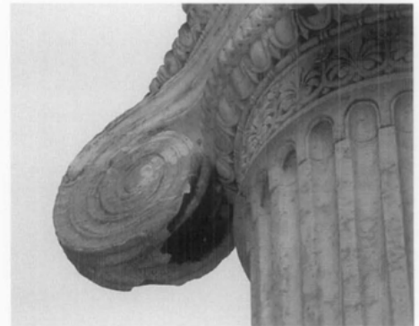
Fig. 9. The column capital volutes were cracked and spalled. Photo: Edmund P. Meade, P.E.
