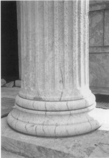
Fig. 10. The column base and plinths had extensive exterior cracks. The internal column cracks were detected by ultrasonic pulse velocity and impulse radar investigation techniques. Photo: Edmund P. Meade, P.E.
