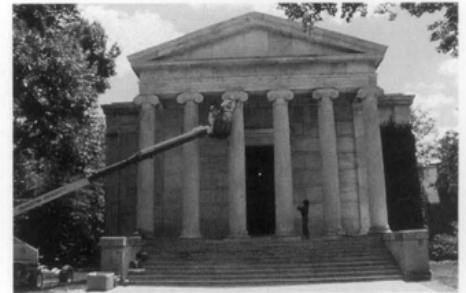
Fig. 13. The non-destructive evaluation of Whig Hall allowed the diagnosis of the condition of the masonry and the specification of a relatively low impact repair. Photo: Edmund P. Meade, P.E.
