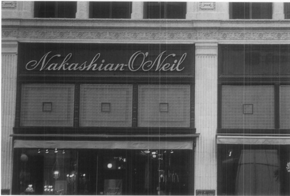
Figure 9. Panels with original tiles are shown on the left next to those featuring replacement textured glass. Photo: Chad Randl.
