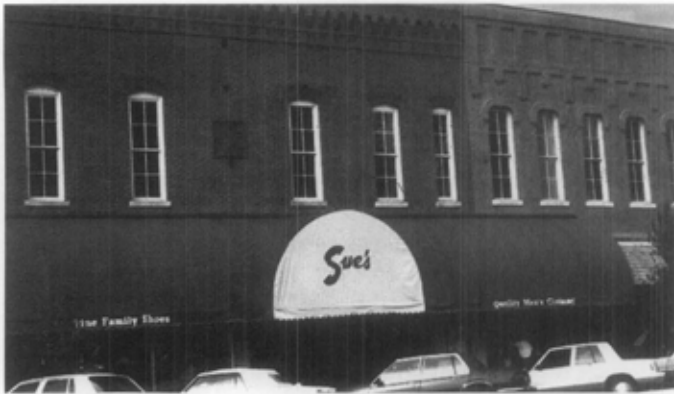
Figure 24. This awning, extending across much of the building, is incompatible in shape. Of greater concern, however, is that its size wholly overshadows the modest historic building behind.
