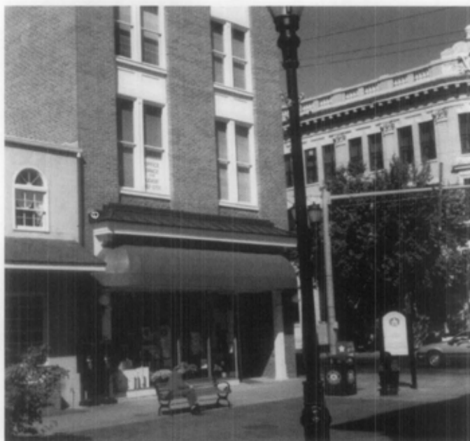
Figure 20. A dome awning was an inappropriate addition to this circa 1890s building. In order to qualify for historic tax credits the new vinyl awning was replaced with a shed awning with a canvas-like woven acrylic covering.
