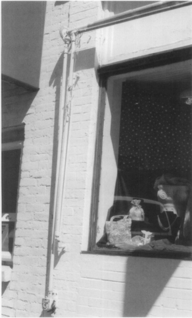
Figure 17. A gearbox, slide rod, roller, front bar, and extension arm reveal that this 19th century building once featured a retractable awning. It is likely that with minor repairs the surviving hardware could again be made operable, recovered with a canvas or acrylic fabric, and reused to service the storefront.
