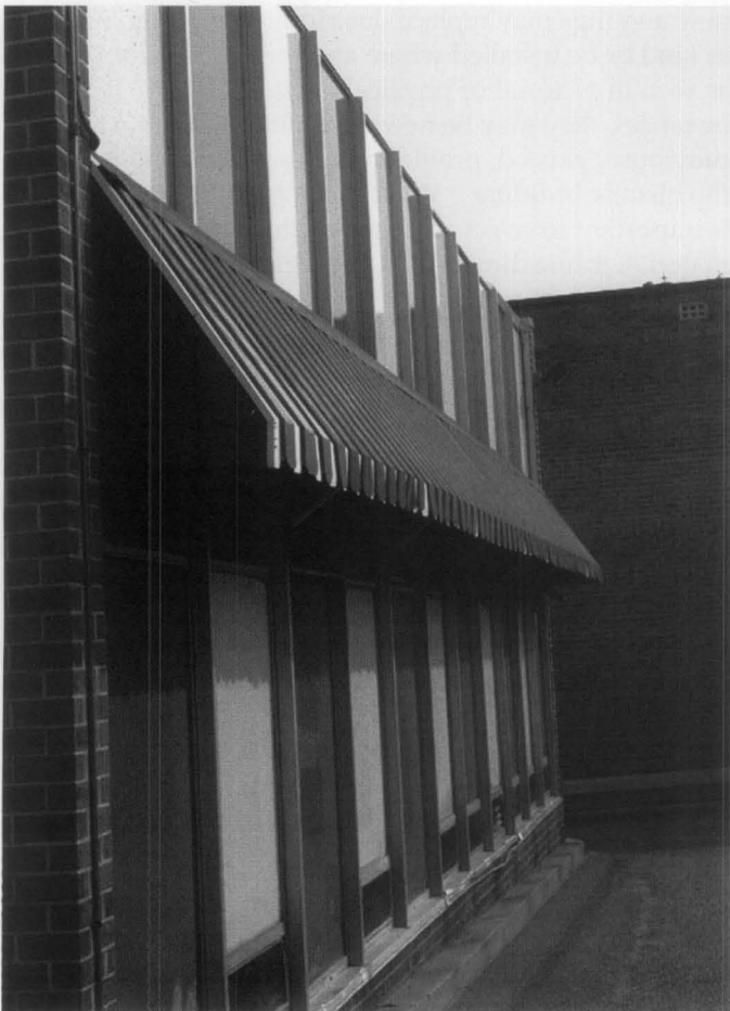
Figure 15. This 1950s-era dry cleaner has an aluminum awning that, with its vertical pattern and alternating stripes, complements the facade's porcelain enamel panes and aluminum mullions. The awning forms an essential element of the building's historic character.
