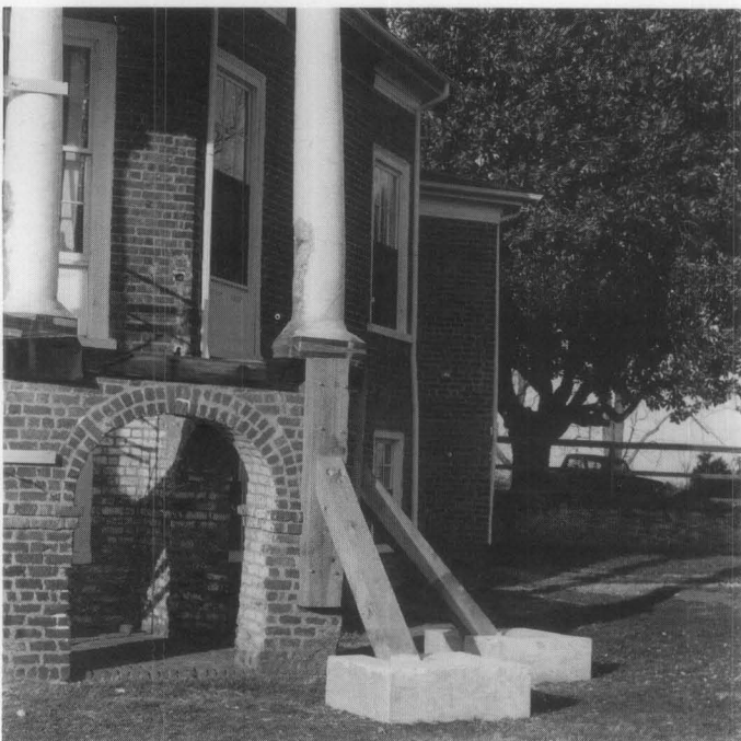
Figure 5. Investigation frequently identifies urgent needs of stabilization. Priority must be given to issues of safety and structural integrity. Supplemental support, such as temporary shoring, may be required to prevent collapse and should be reviewed by a structural engineer.
