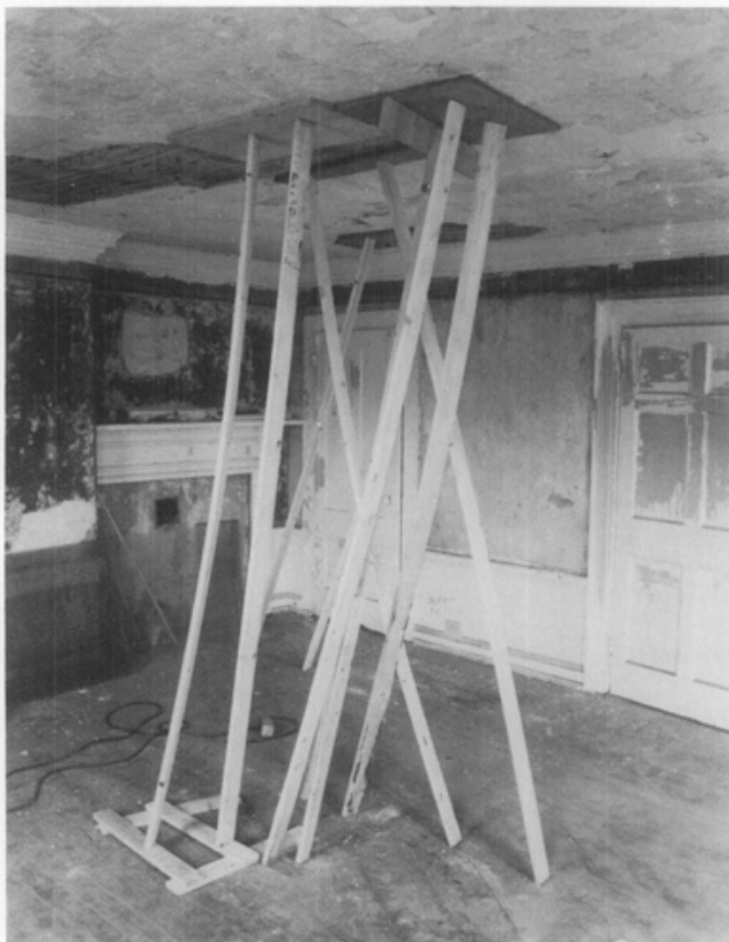
Fig. 15. When ceiling repairs are made with wet plaster or with an injected adhesive mixture, the old loose plaster must be supported with a plywood brace until re-keying is complete. Photo: John Leeke.
