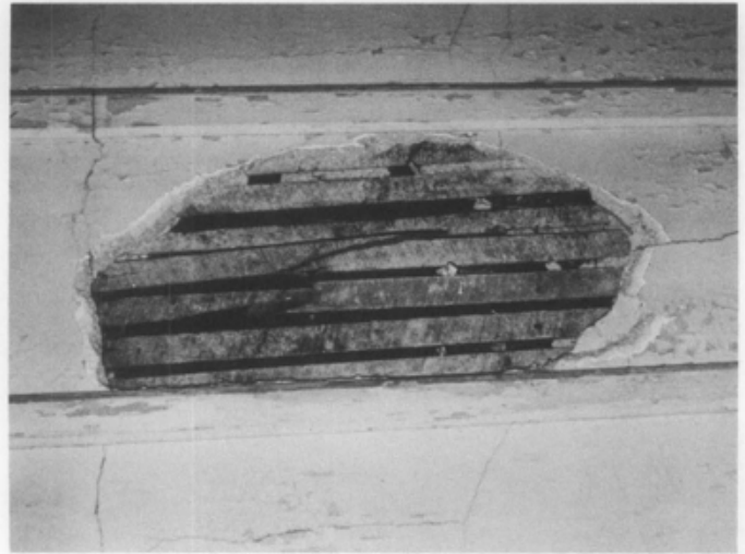
Fig. 13. This beaded ceiling in one of the bedrooms of the 1847 Lockwood House, Harpers Ferry, West Virginia, is missing portions of plaster due to broken keys. This is attributable, in part, to deterioration of the wood lath. Photo: Kaye Ellen Simonson.
