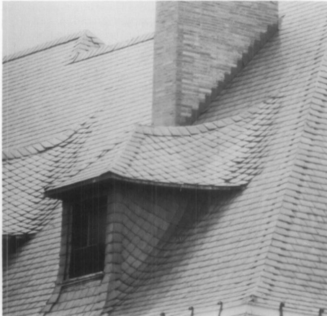
Because of the roof's visibility, the slate detailing around the dormers is important to the character of this structure. Note how the slates swirl from a horizontal pattern on the main roof to a diamond pattern on the dormer roofs and side walls. (18th and Que Streets, NW, Washington, D.C.)
