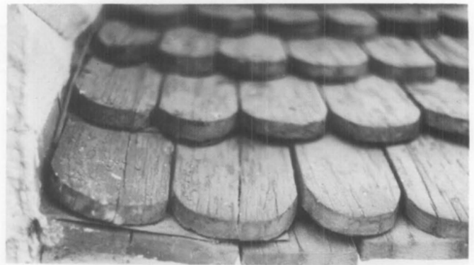
Replacement of particular historic details is important to the individual historic character of a roof, such as the treatment at the eaves of this rounded butt wood shingle roof. Also note that the surface of the dormer was carefully sloped to drain water away from the side of the dormer. In the restoration, this function was augmented with the addition of carefully concealed modern metal flashing. (Mount Vernon, Virginia)
