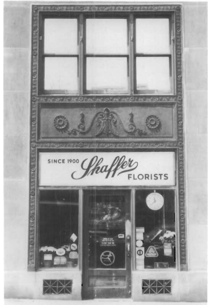
Figure 32. Bronze Storefront, Grilles, Spandrel Panel, and Window, Southern Railway Building, 912 Fifteenth Street, NW, Washington, D.C., 1928; Waddy Butler Wood, architect. This building is typical of many large commercial buildings with extensive use of bronze. Everything from the grilles to the windows and spandrels to the storefronts were fabricated of bronze. Although many storefronts have been remodelled beyond recognition, this one still has its original design and materials. (David W. Look)
