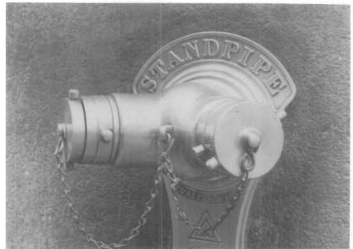
Figure 37. Brass Siamese Standpipe Connection, Rookery Building, 209 South LaSalle Street, Chicago, Illinois, 1886; Burnham and Root, architects; W. D. Allen, manufacturers. Brass fittings can be functional and very attractive when kept well polished. Even though the natural weathered dark patina on brass is protective, it is generally considered to be unsightly and great effort is expended to recapture the metallic gleam. (Margot Gayle)
