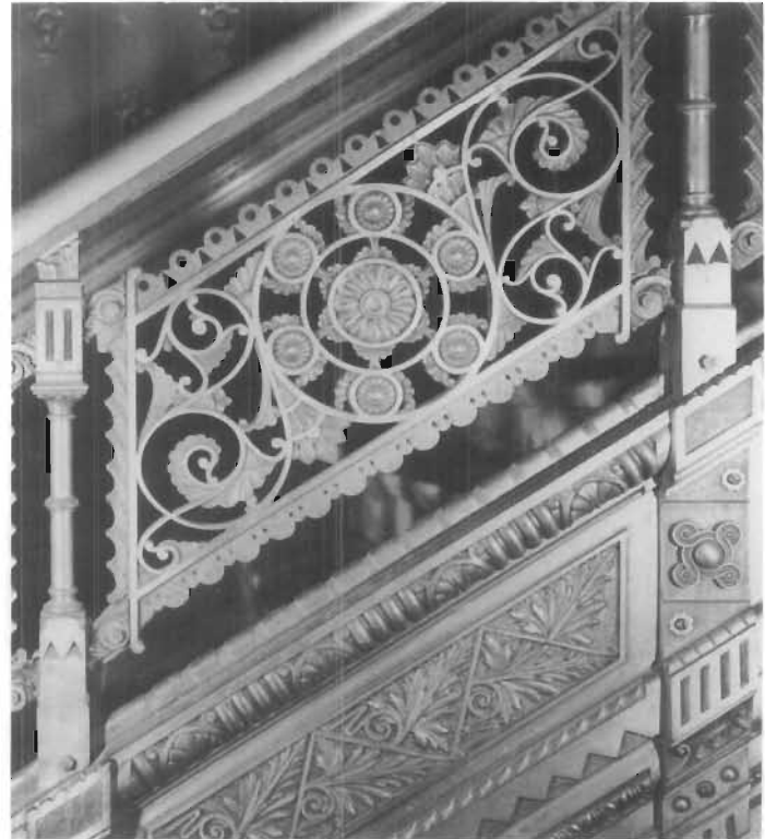
Figure 26. Copper-Plated Cast-iron Stair Railing, Christian Heurich Mansion, 1307 New Hampshire Avenue, NW, Washington, D.C., 1892–1894; John Granville Meyers, architect. This iron railing was sand cast in many pieces, and the flat areas of the design were ground smooth before the pieces were copper plated. Most of the parts were bolted together, but a few pieces of the newell post were brazed. The railing has a brass hand rail. (Jack E. Boucher, NAER)
