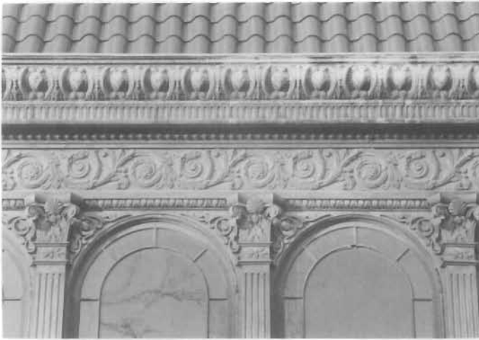
Figure 23. Pressed Copper Sheet Metal Cornice, Frieze, and Pilasters; Conservatory of the Christian Heurich Mansion, 1307 New Hampshire Avenue, NW, Washington, D.C., 1902; Appleton Clark, architect. The copper work was assembled from many pieces of sheet copper pressed with low relief designs. (Jack E. Boucher, NAER)
