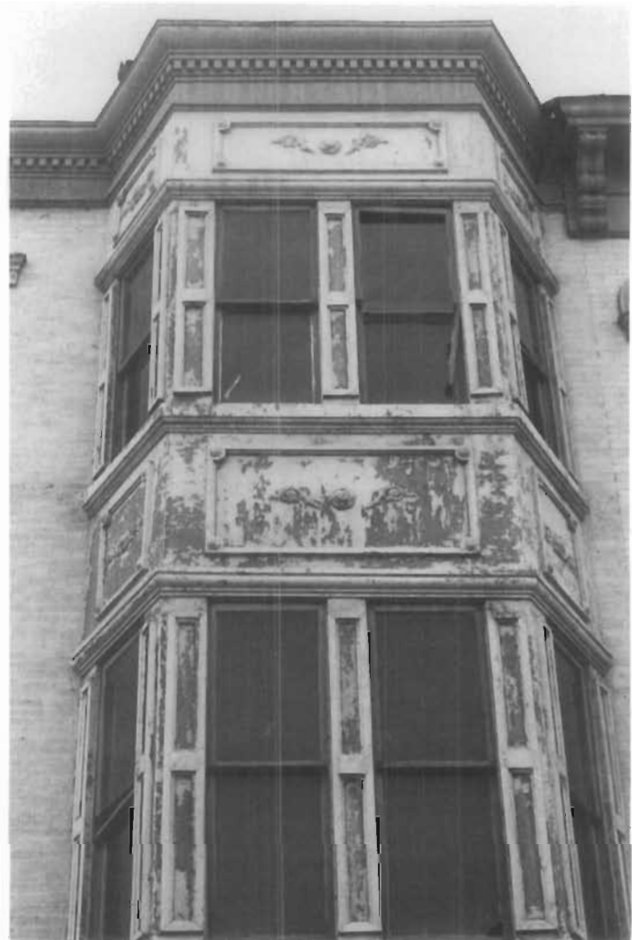
Figure 18. Galvanized Sheet Iron Bay with Applied Zinc Ornament, 608 Indiana Avenue, NW, Washington D.C. When sheet metal work is kept well painted, it is very difficult to identify it as sheet iron or steel, galvanized or tinned. However, if the metal is not maintained, its composition becomes more obvious. Paint does not adhere well to pure zinc, or to galvanized iron or steel. When the paint peels, it usually comes off completely, including the primer, to reveal a clean metal surface. If the metal is galvanized, it will have a spangled appearance and may show some rust or rust stains from the iron base metal. If it is cast or pressed zinc, it will have a grayish-white appearance. This bay is covered with galvanized sheet iron with pure zinc ornaments on the surface. Even if well painted, a magnet test will reveal what is galvanized iron or steel (which is magnetic) and what is pure zinc (which is non-magnetic). (David W. Look)
