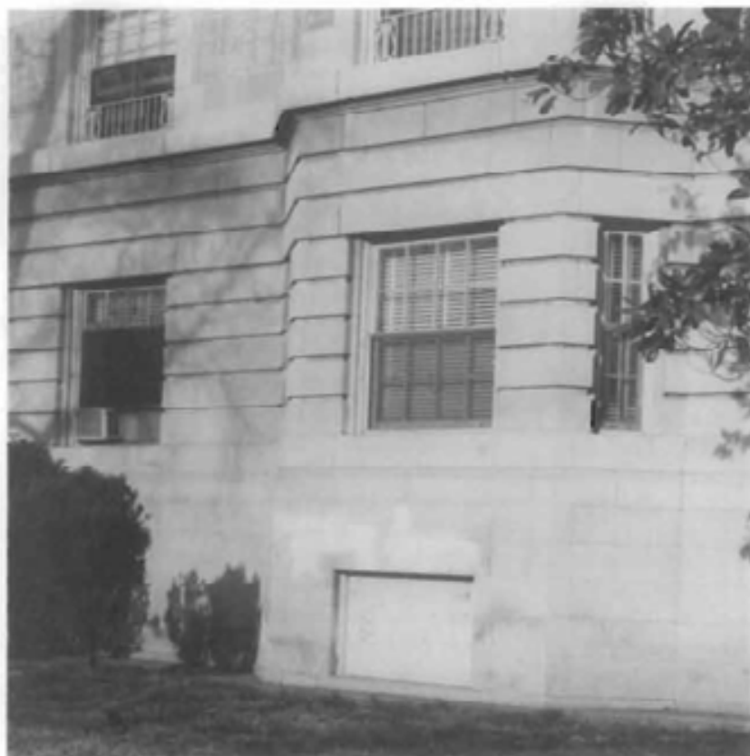
Figure 1. When an inappropriate chemical cleaner was used to remove graffiti, it resulted in permanently bleaching the limestone foundation, and left a mark as unsightly as the graffiti.
