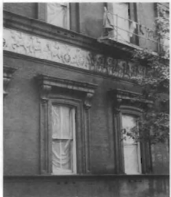
Figure 11. Removal of 100 years of grime from the brick and terra cotta facade of the Pension Building (now the National Building Museum), Washington, D.C., was accomplished by workmen on a swing stage using a chemical cleaning product. Note the polyethylene covering the windows to prevent damage. Also note the protective clothing for the workmen which hangs on the platform while not in use. Photograph: Christina Henry
