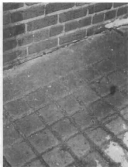
Figure 14. Although the sodium hydroxide-based test cleaning patch on the right side of this wall of common brick appears to have been successfully cleaned, closer inspection reveals that a minute portion of the brick surface has been dissolved and removed by the cleaner. As a result, considerable brick dust can be seen in the cracks of the pavement beneath the wall.
