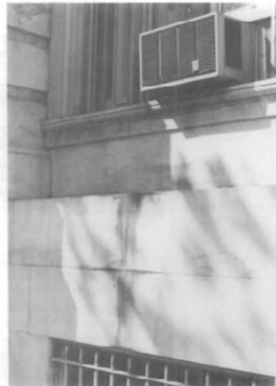
Figure 22. The discoloration on this white marble is a green-colored algae growth on a shady side of the building and caused by water dripping from the air-conditioner above it.
