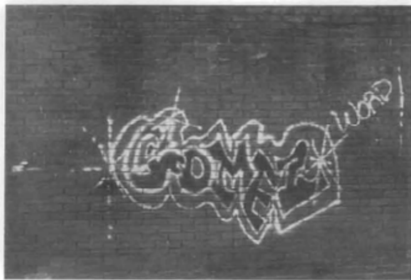
Figure 24. Spray-painted graffiti on this brick wall can be removed with paint remover, and in this case, probably will not require poulticing.
