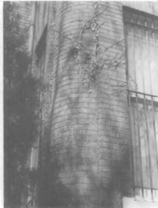
Figure 21. After the ivy was cut at the roots, it has been allowed to wither and die before being pulled off the wall. Most of the ivy has been removed, but a few tendrils still cling higher on the wall. After these have completely dried and have been pulled off, the remaining dried plant material can then be removed from the brick by scrubbing with water and a bristle brush.
