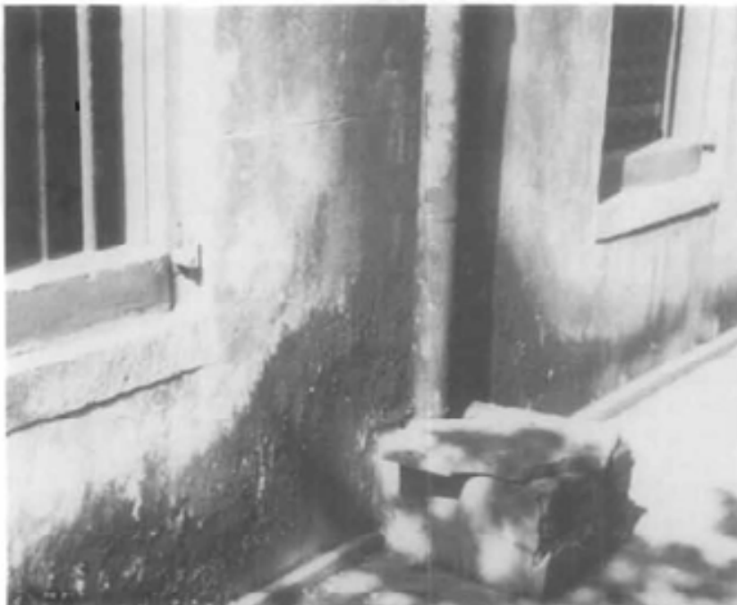
Figure 23. The moss growing around the downspout and along the base of this stucco building clearly indicates the presence of excess moisture—here due to rising damp as well as a leaky downspout. Photograph: Lee H. Nelson, FAIA
