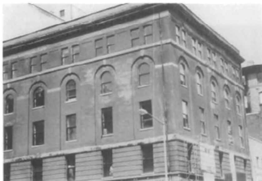
Figure 26. Efflorescent salts appearing on many of the brick piers of this turn-of-the-century building may indicate the existence of clogged interior gutters that, because they no longer function have been supplemented by an exterior rain removal system. Photograph: National Park Service
