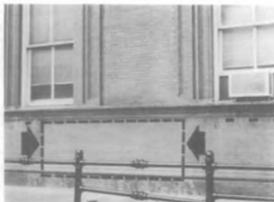
Figure 9. A test patch on brick to remove a century of dirt reveals only a slight difference in appearance between the cleaned and the uncleaned brick. The hard-baked outer skin of the brick provides a surface that is not only impervious to dirt penetration, but resists dirt accumulation. Photograph: Christina Henry
