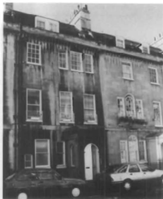
Figure 2. The building on the left is an obvious candidate for cleaning, as the heavy black crust may be concealing or contributing to deterioration of the stone. Despite its more recent cleaning, the stone facade of the house on the right exhibits the same distinctive, and hard-to-eliminate rainwater wash patterns under the eaves and window sills, as its unwashed neighbor.
