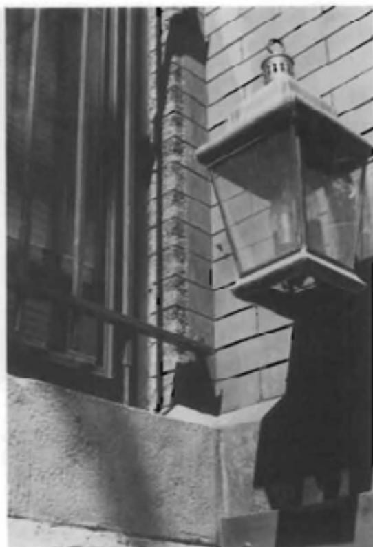
Figure 27. Heavily pitted by sandblasting, this window recess provides a vivid contrast to adjacent un-damaged brick protected from abrasion by a metal signboard.
