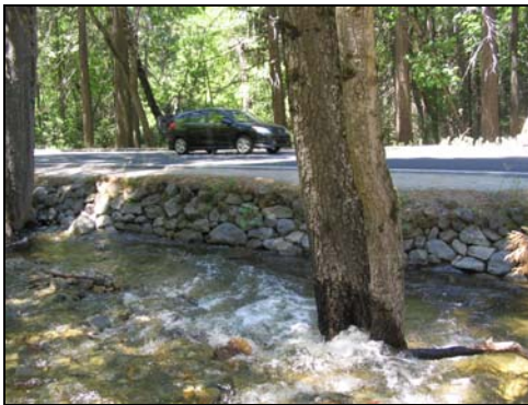
Seasonal flooding at Bridalveil Creek drainage
