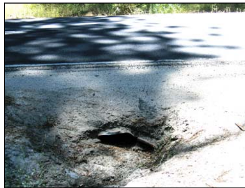
Dysfunctional culvert at El Capitan Straight
