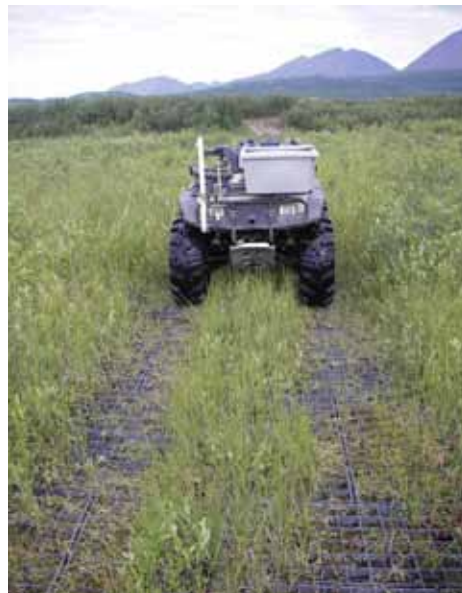
Trail repairs on BLM lands off the Denali Highway. This is a good example of the type of trail hardening proposed within the Nabesna ORV EIS.
