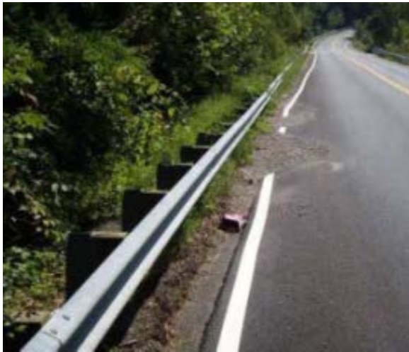
Sediment collecting along roadways hinders bicycle safety
