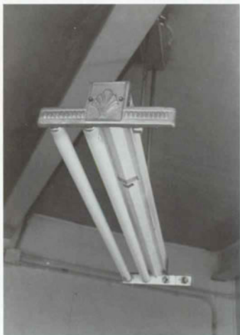
Fig. 45. Room 205 (Records Office), Light Fixture Type FL-C [1988].
