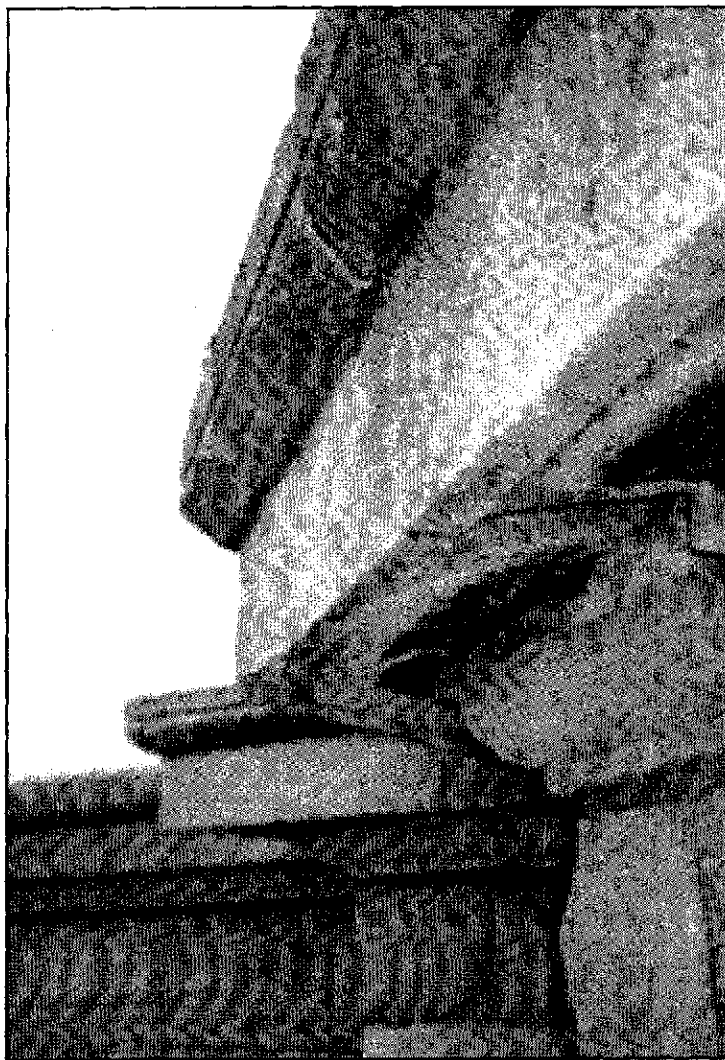
Figure 5.12: Monument Lodge, west facade, detail gypsum crust on underside cornice.
