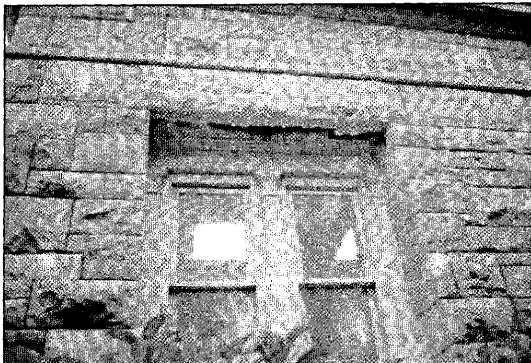
Figure 5.9: Monument Lodge, exterior, detail of gypsum crusts at north window to mens' rest room.
