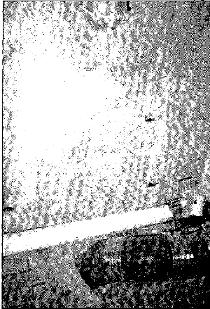
Figure 5.34: Monument Lodge, interior, boiler room, note concrete delamination at southeast ceiling.
