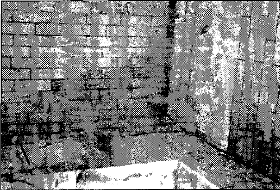
Figure 5.16: Monument Lodge, east façade, south end of vault over portico, note water infiltration.
