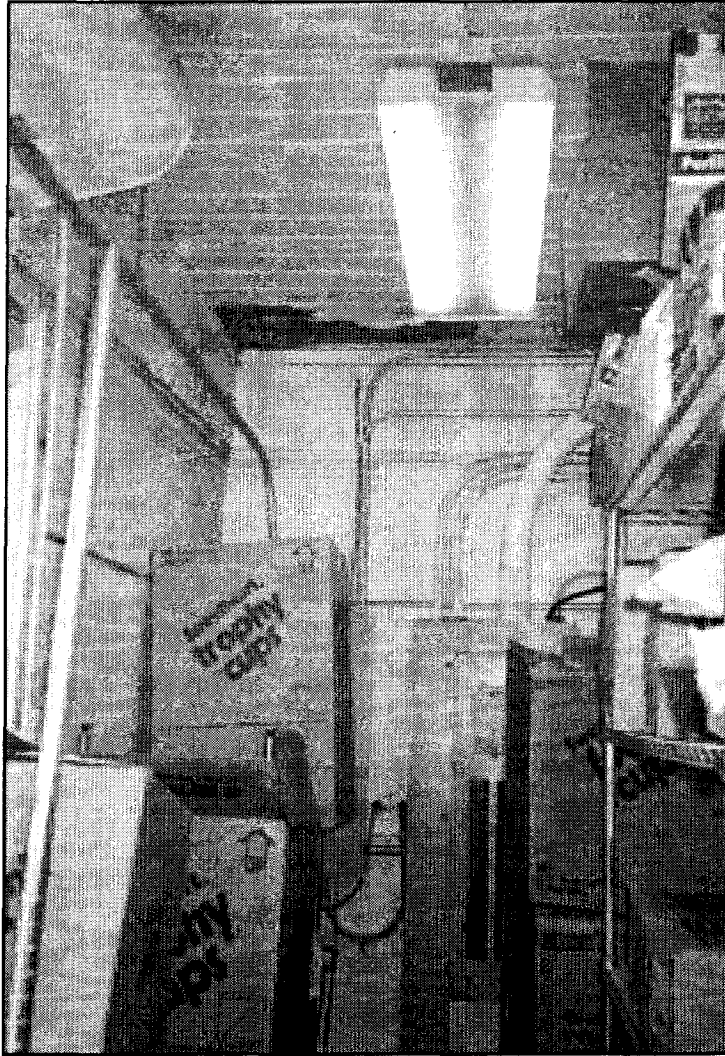
Figure 5.26: Monument Lodge, interior, Concession Addition, storage, southwest corner, note damage at ceiling.
