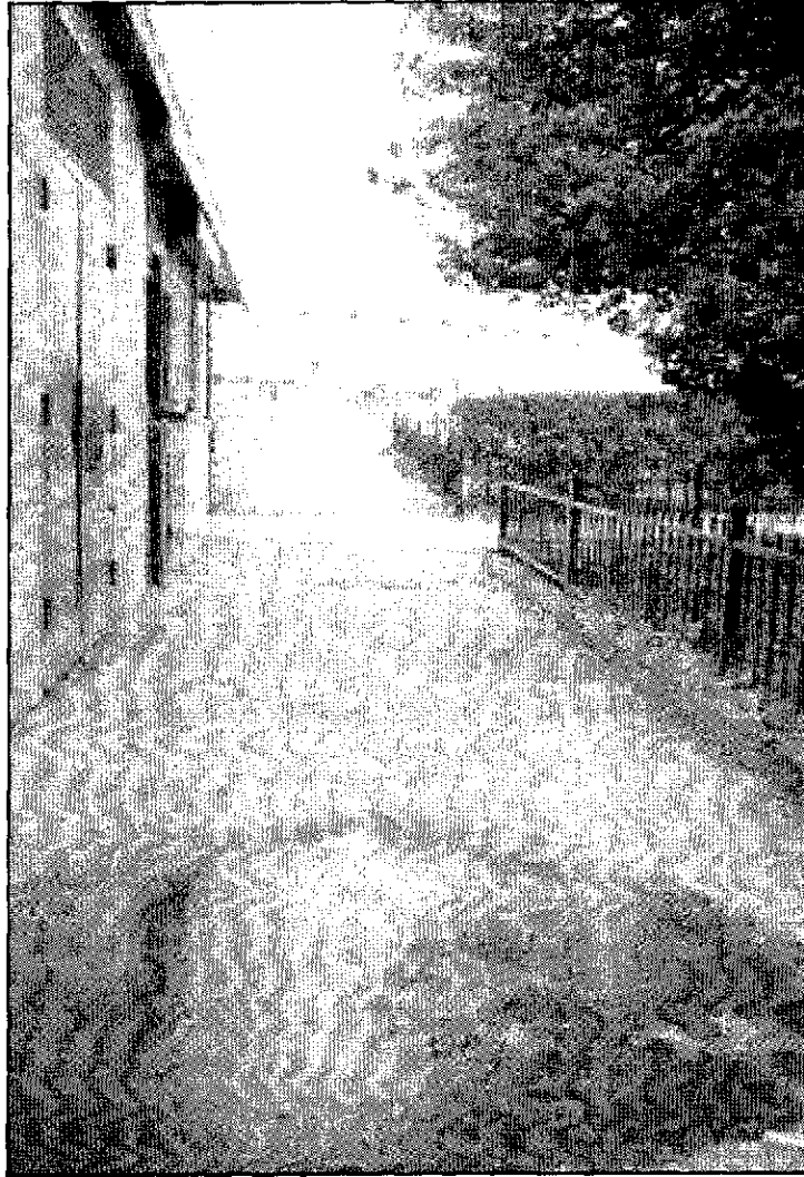
Figure 5.2: Monument Lodge, Concession Addition, north façade, uneven paving showing pooled water.
