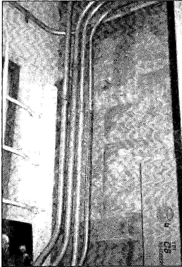
Figure 4.44: Monument Lodge, interior, concession addition, souvenir shop storage, junction of lodge masonry and concession addition at northeast corner.
