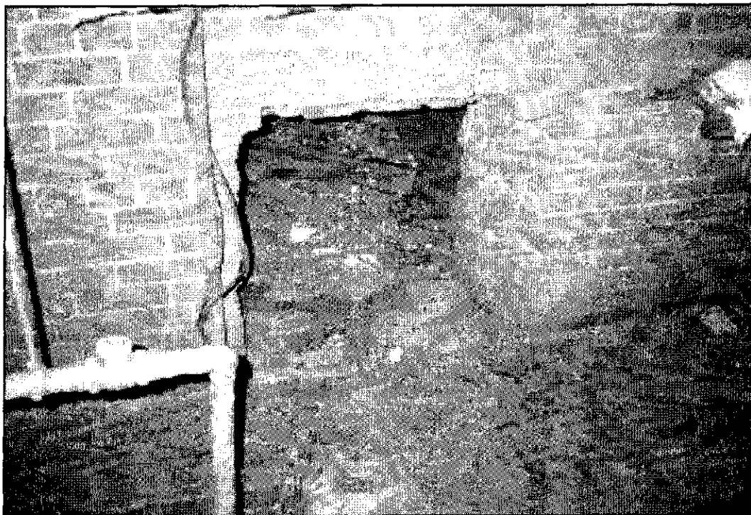
Figure 4.43: Monument Lodge, interior, boiler room, entrance and threshold to concrete coal bin on north.
