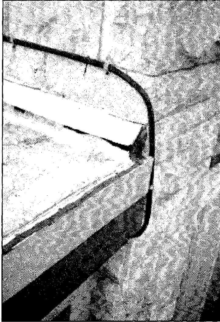
Figure 4.16: Monument Lodge, concession addition roof, flashing at southeast edge.
