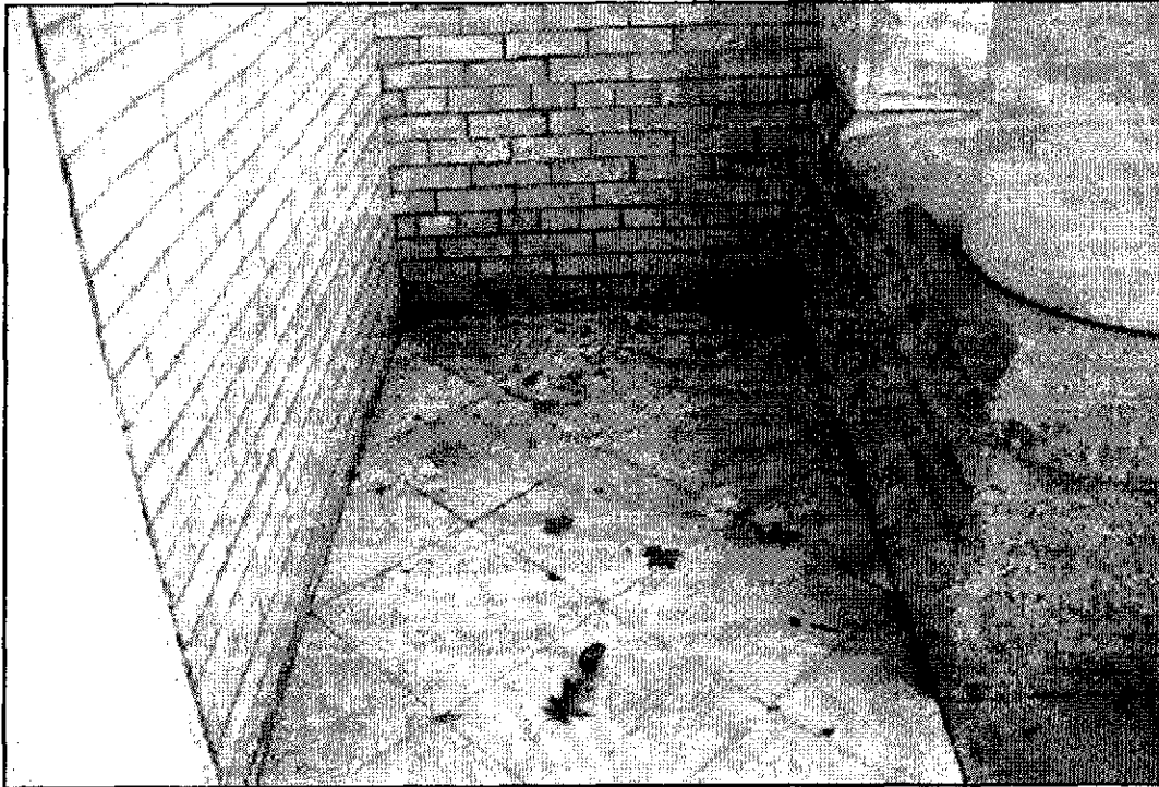
Figure 5.6: Monument Lodge, east façade, northern end of portico paving, note biological growth on brick.
