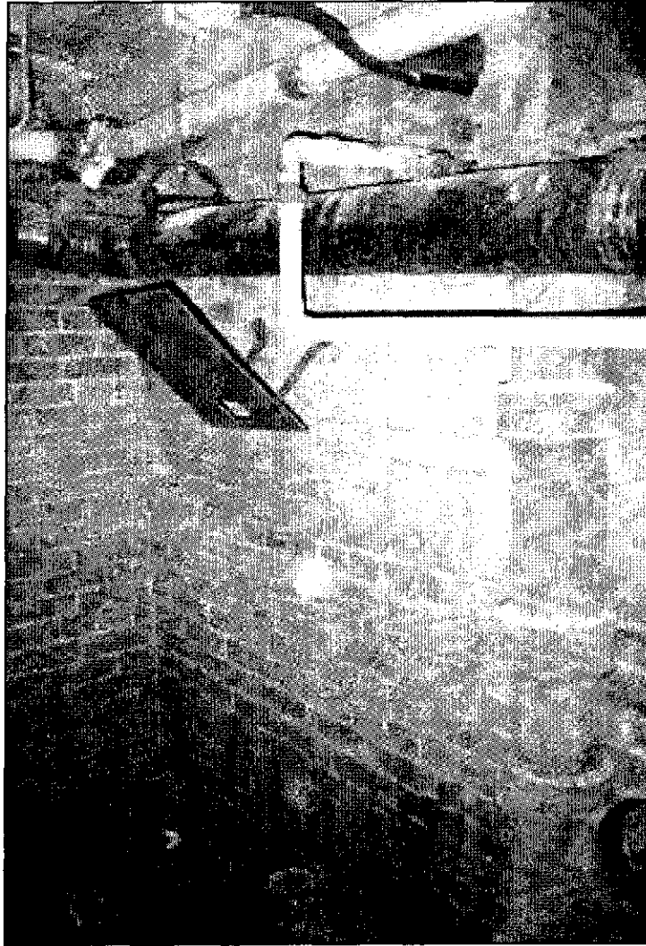
Figure 4.40: Monument Lodge, interior, boiler room, looking southeast.
