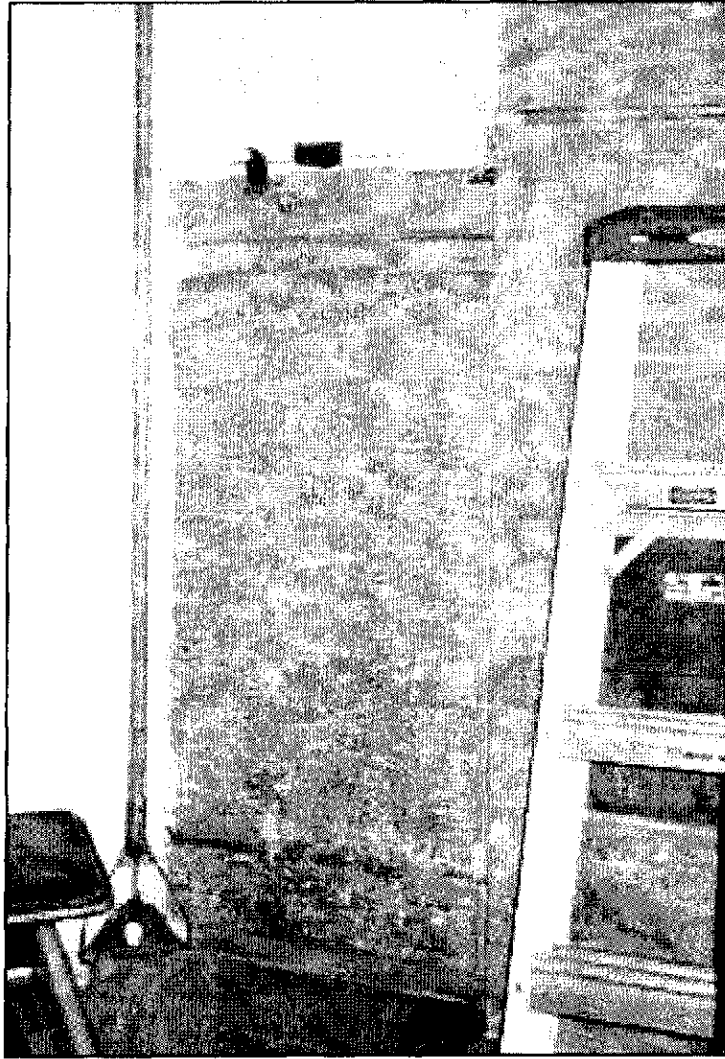
Figure 4.47: Monument Lodge, interior, concession addition, mechanical room with exposed stone panel detail.
