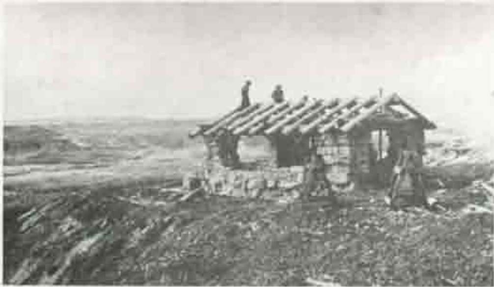
Illus 16. Shelter at Little Missouri River overlook, under construction (photograph from park files, taken ca. 1937)
