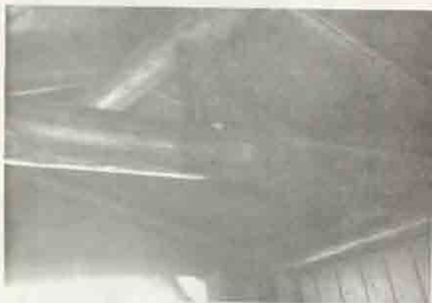
Illus 12. Details of ceiling, large shelter at Squaw Creek campground (photograph by author, taken October 1977)
