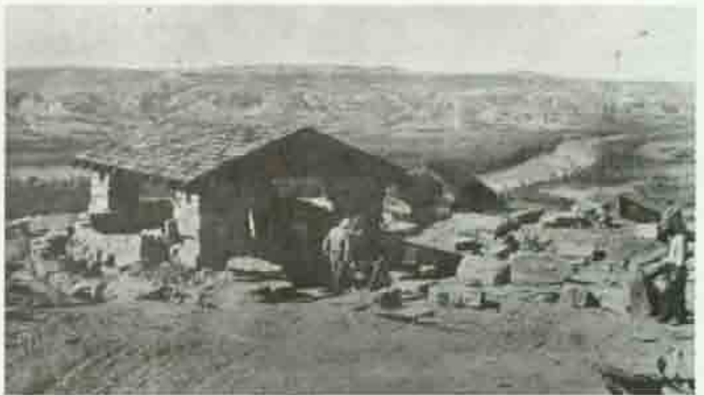
Illus 17. Shelter at Little Missouri River overlook, under construction (photograph from park files, taken ca. 1937)
