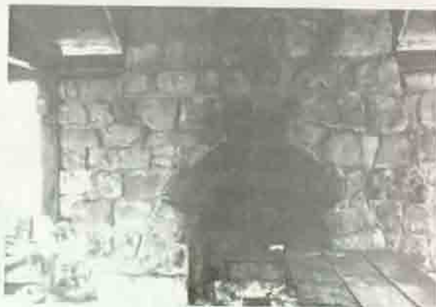
Illus 13. Fireplace in front chamber, large shelter at Squaw Creek campground (photograph by author, taken October 1977)
