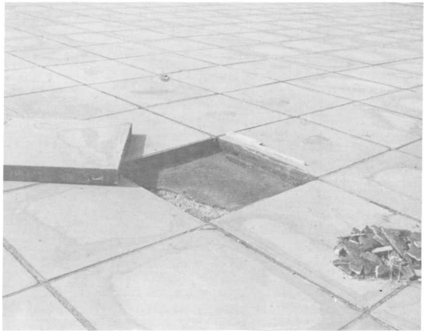
ILLUSTRATION 147. General view of lower plaza sandstone pavers showing typical stained condition.
