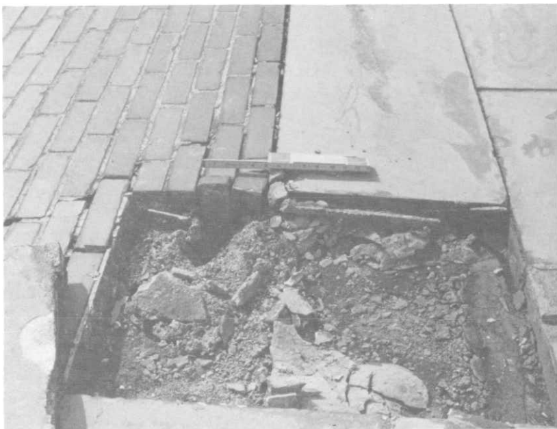
ILLUSTRATION 129. Detail view of condition of concrete fill slab and setting bed below sandstone and brick pavers of upper plaza.
