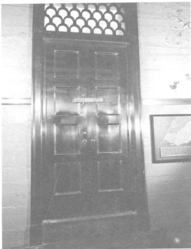
ILLUSTRATION 89. View of bronze door from observation gallery indicating faulty or missing hardware, lack of weather-stripping and dissimilar finish of bronze.
