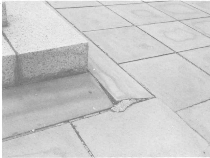
ILLUSTRATION 148. Detail view at east end of granite steps showing inclined pavers due to settling of lower plaza.
