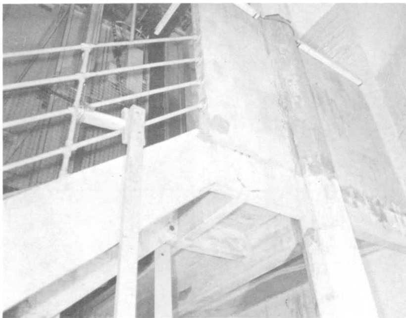
ILLUSTRATION 41. View of underside of upper elevator landing showing typical octagonal column and backside of concrete wall at landing level.
