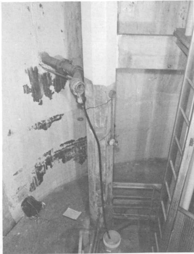
ILLUSTRATION 216. View of interior rainwater conductor serving the observation deck. The floor drain on the deck has been reworked for a free fall to the outside. However, during heavy rains, water will flow from this pipe into the bucket.
