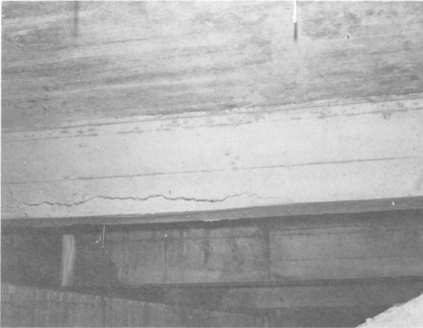
ILLUSTRATION 127. View of a typical beam with crack formed by rusting steel bars behind.
