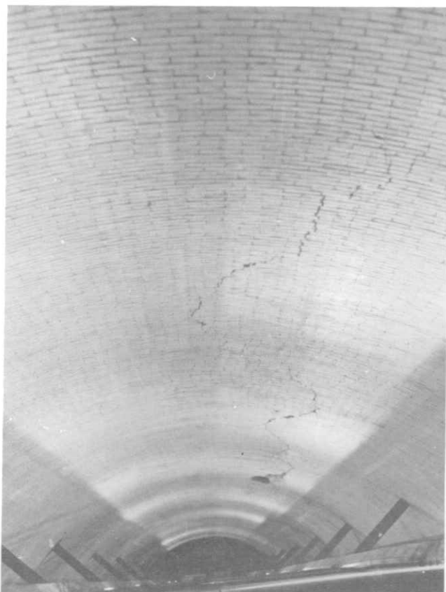
ILLUSTRATION 54. Overall view down column shaft at south quadrant showing major crack.
