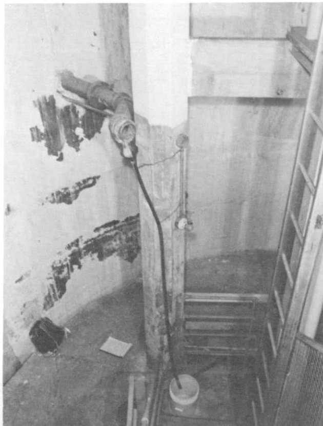
ILLUSTRATION 77. View of interior of penthouse at the southwest column showing pipe from original floor drain of observation gallery. Peeled paint is the result of moisture penetration.
