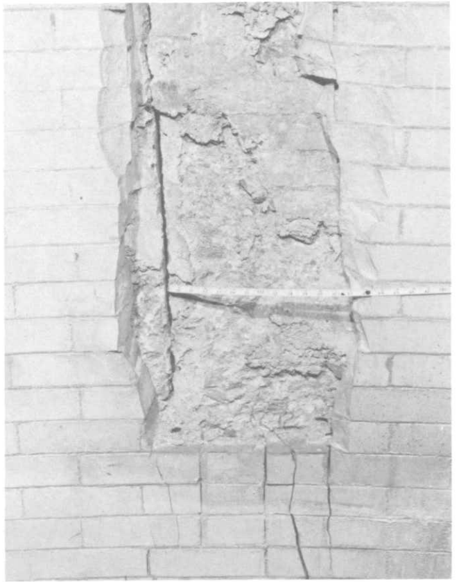
ILLUSTRATION 47. Detail view showing structural concrete with major crack; brick and mortar with wire loop, minimum depth of crack.
