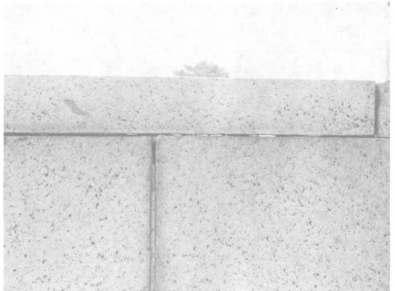
Illustration 156. Detail view of typical mortar joints in retaining walls. Note that daylight may be seen through horizontal joint indicating a lack of mortar.
