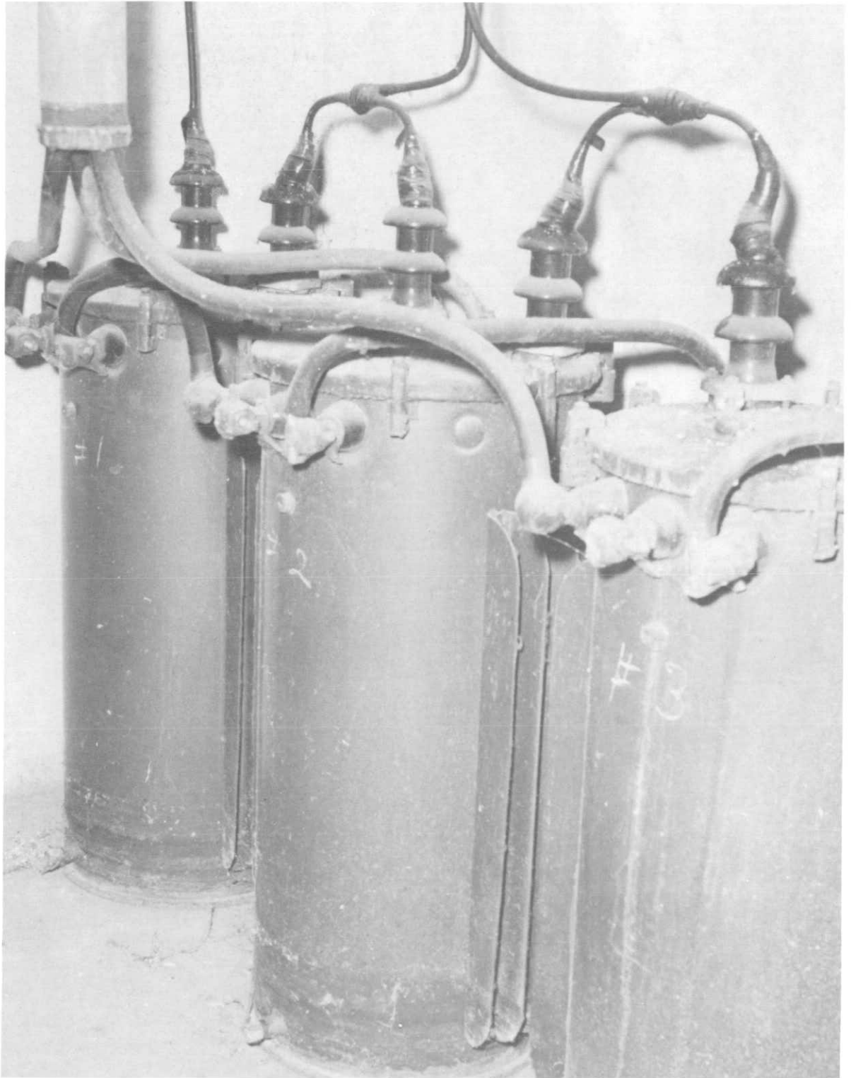
5a. 3-PHASE TRANSFORMER BANK These transformers should be cleaned, rust removed, and painted with a rust resistant transformer paint. The right side transformer tested fair. We recommend a re-test in one year.
