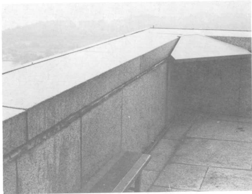
ILLUSTRATION 72. View towards northeast of parapet walls around observation gallery. Metal map of battle appears at corner.
