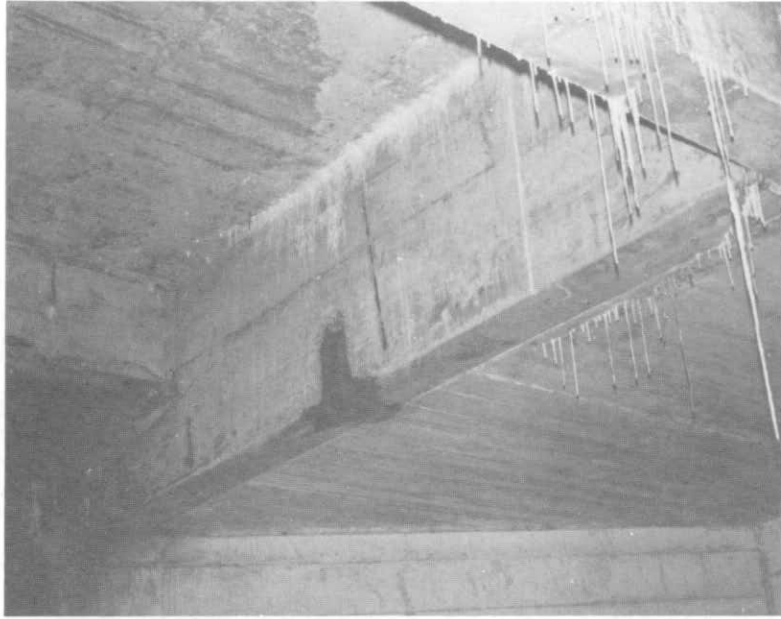
ILLUSTRATION 169. General view of underside of a planting box slab which is typically in the same plane as the bottom of the beam. Note that no drains were evident. Dark stain is probably seepage through bottom of box.
