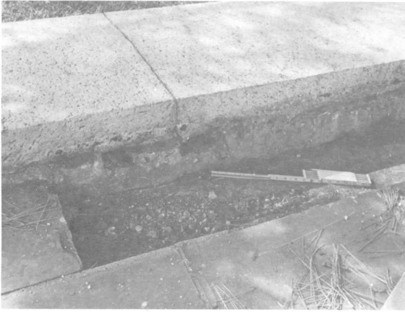
ILLUSTRATION 150. Detail view showing granite curb at the top of a concrete grade beam. Note that the top of the paver is about 2" below its original level, indicated by the line of rough to smooth granite.
