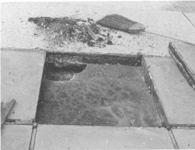
ILLUSTRATION 140. Detail view of top tread of granite steps at upper plaza and typical setting bed condition under sandstone paver.
