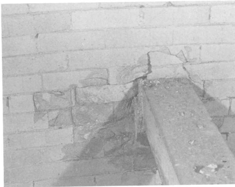
ILLUSTRATION 51. Detail of spalled brick at 6" by 6" concrete column brace and face of brick.
