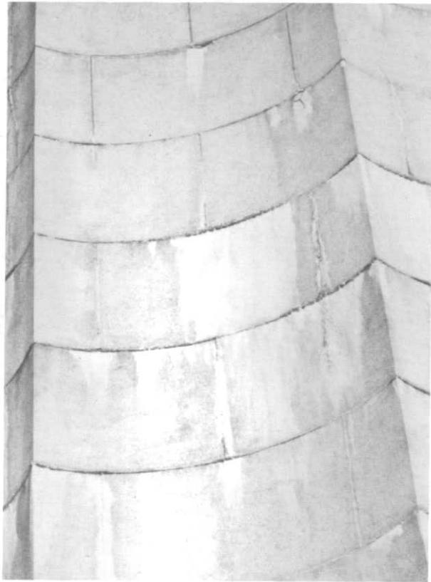
ILLUSTRATION 32. Typical detail of efflorescence and improperly sealed joints.
