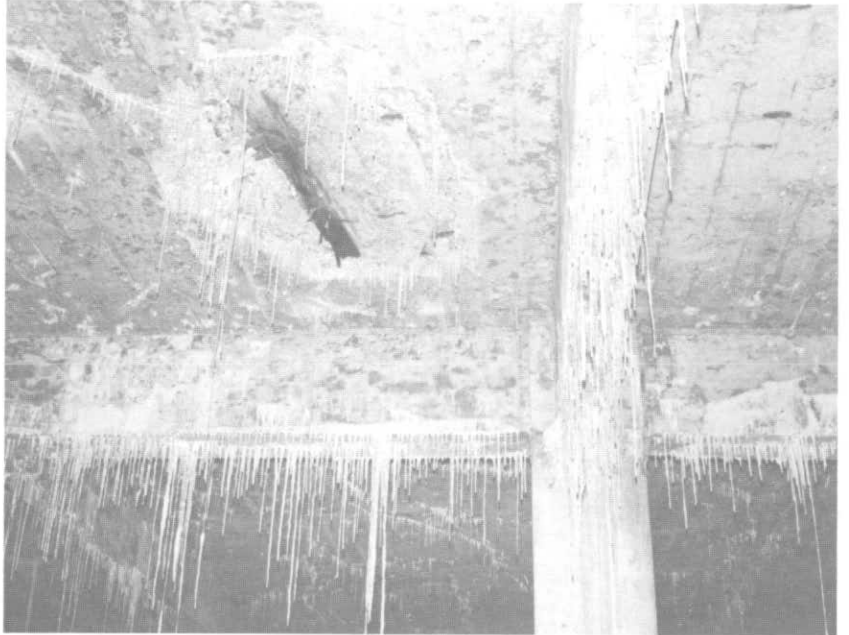
ILLUSTRATION 114. Typical condition of stalactites at underside of upper plaza slab and beams.
