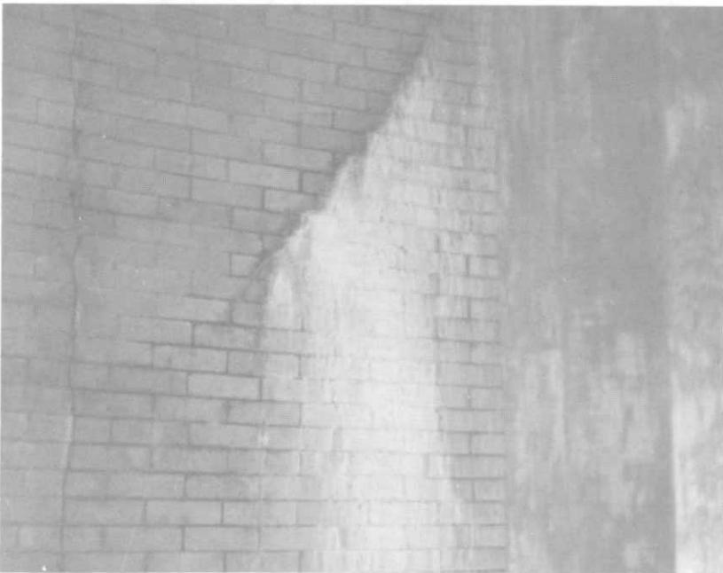
ILLUSTRATION 50. Detail of a major efflorescent stain, located in west quadrant at level 3.
