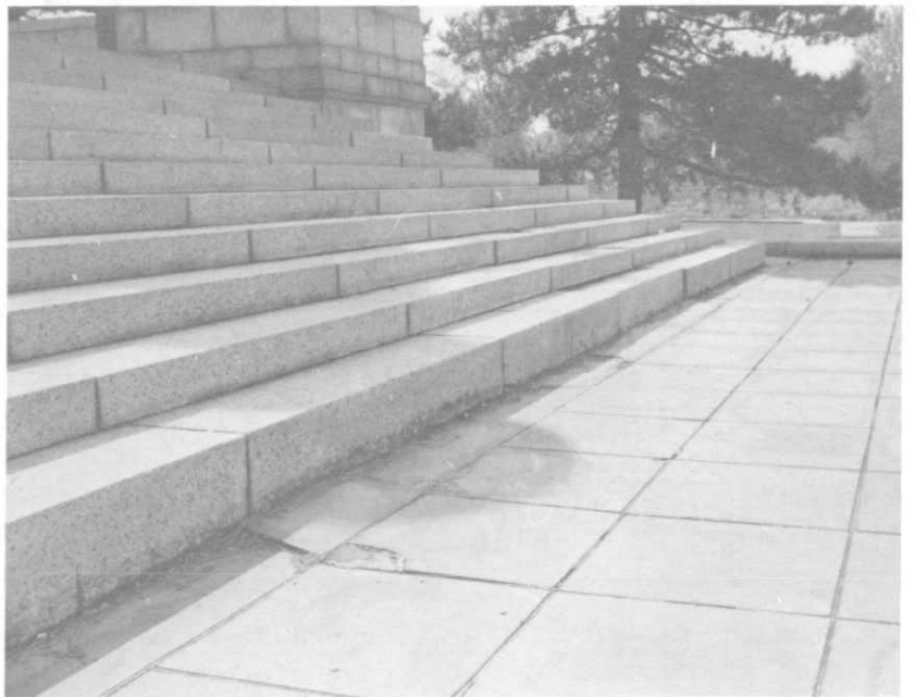
ILLUSTRATION 142. View along lower risers of granite steps looking toward the west. Note settling of lower plaza and misaligned steps.
