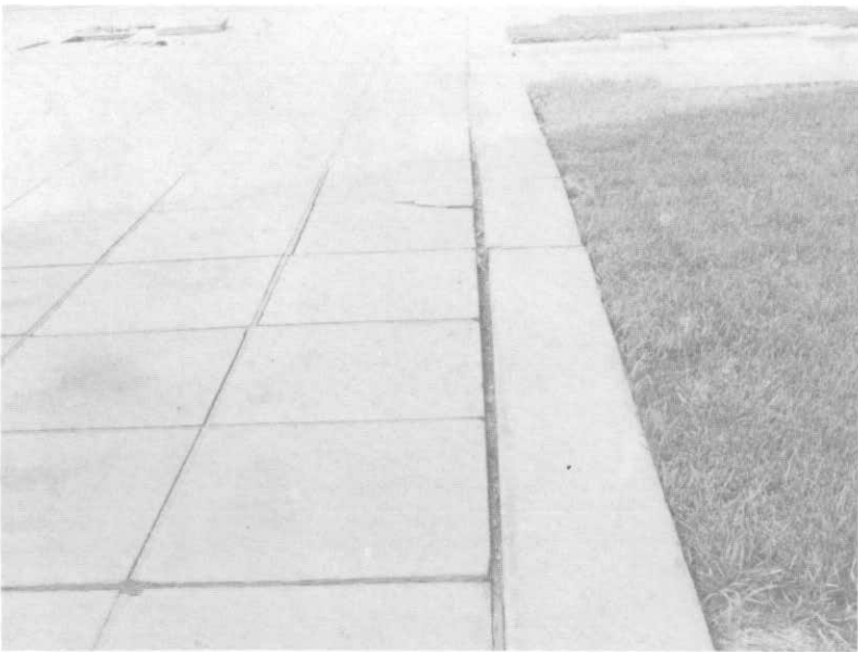
ILLUSTRATION 170. General view of upperside of a typical planting box. Note poor joints between sandstone pavers and sandstone curbstones. See Illustration 171 for section through planting box and recommended waterproofing.
