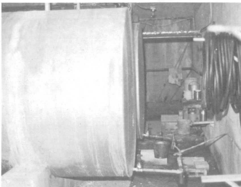
ILLUSTRATION 205. View of the fuel oil storage tanks. Note the pipe stubbed out from the wall immediately below the coiled hose is the discharge pipe from the sump pump in the equipment room located behind this wall.
