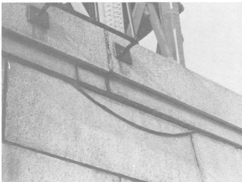
ILLUSTRATION 78. Detail at cornice of penthouse indicating sealant failure. Pipe railings were added with navigational lights at later date.
