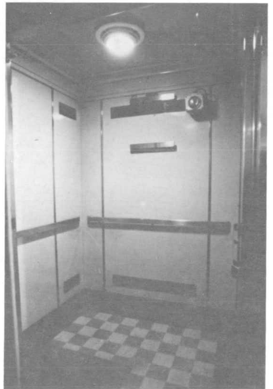
ILLUSTRATION 260. Existing elevator. Note emergency battery lighting unit in rear.
