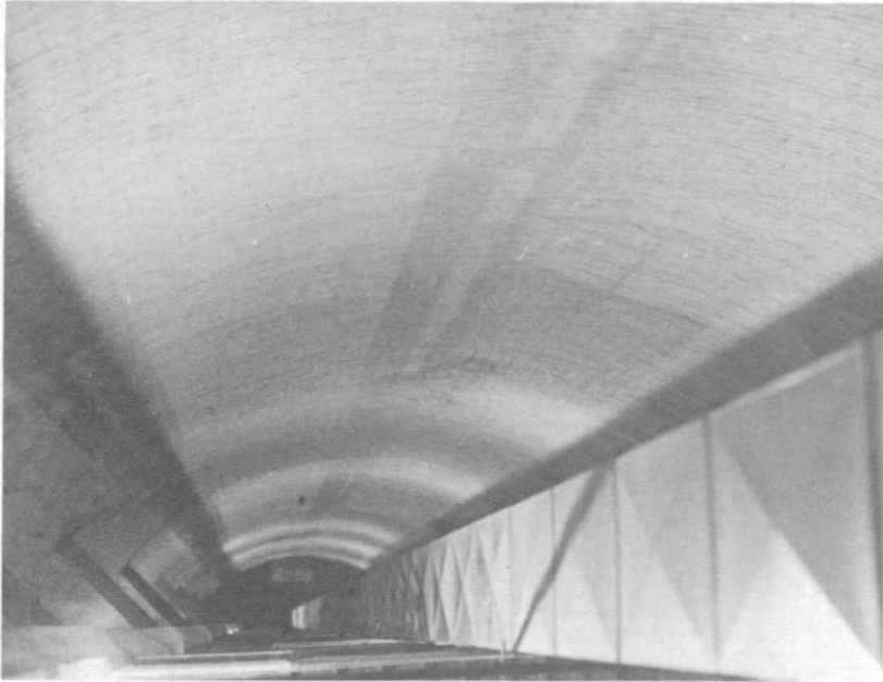
ILLUSTRATION 189. View of supply air duct within the column shaft. Photo taken from an upper level looking down.
