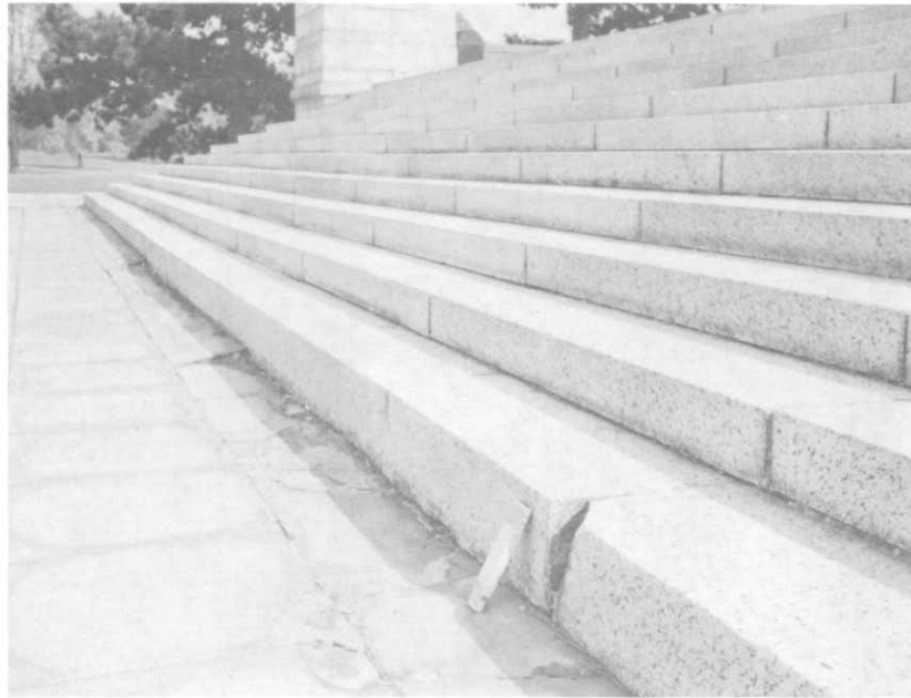
ILLUSTRATION 143. View along lower risers of granite steps looking toward the east. Note chipped stone and poor joints.
