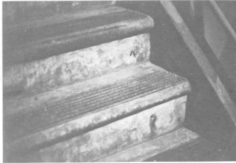
ILLUSTRATION 38. View of stair tread and riser showing the typical existing safety tread with round nosing in good condition.
