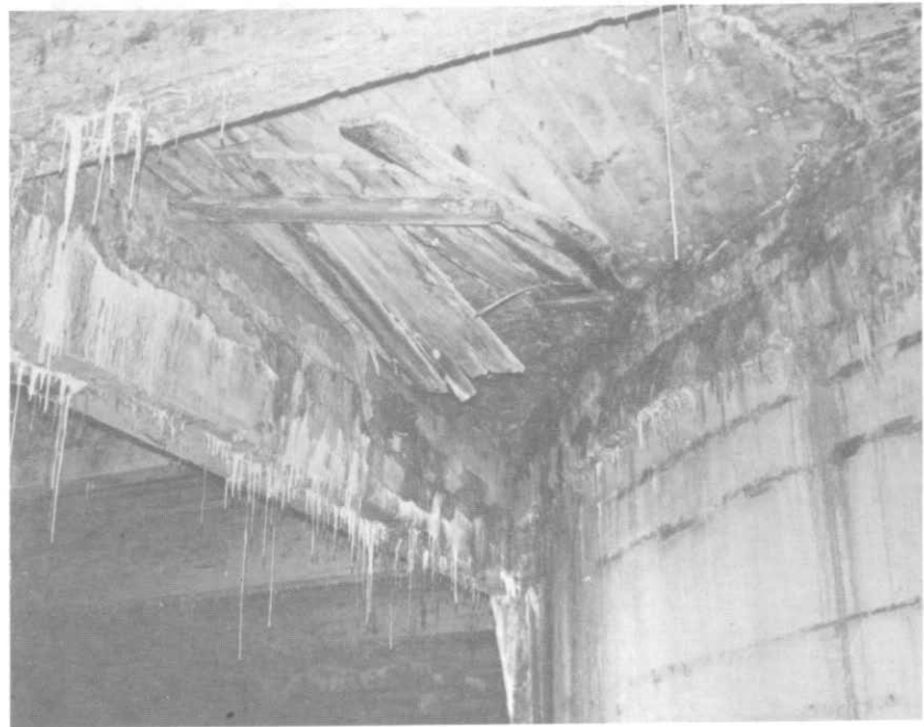
ILLUSTRATION 26. Top of column foundation at approximately northwest side, just below upper plaza.
