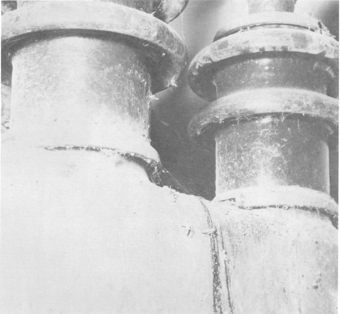
4d. MAIN OIL CIRCUIT BREAKER The extremely dirty bushings should be cleaned, and the connections tightened and insulated.
