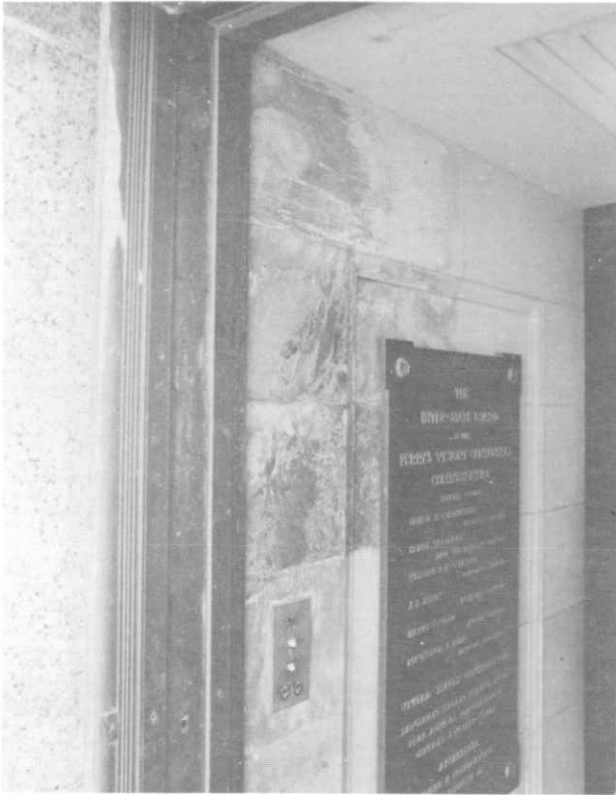
ILLUSTRATION 181. Detail view of north door frame showing corrosion and missing frame screws.
