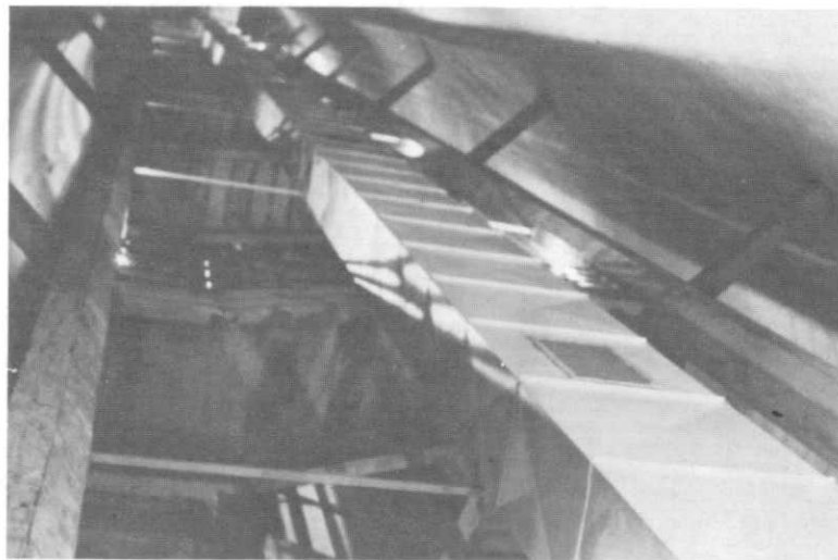
ILLUSTRATION 190. View of the return air duct within the column shaft looking up.
