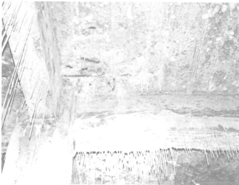
ILLUSTRATION 115. Detail view of typical beams to column intersection showing stalactites at various stages of formation.
