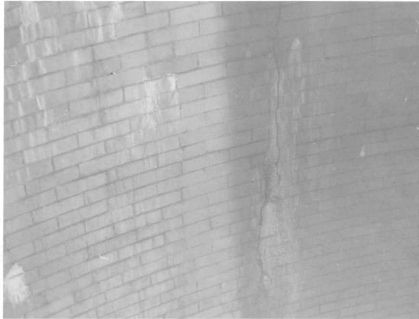
ILLUSTRATION 49. Typical efflorescence and brown stains which occur throughout shaft.
