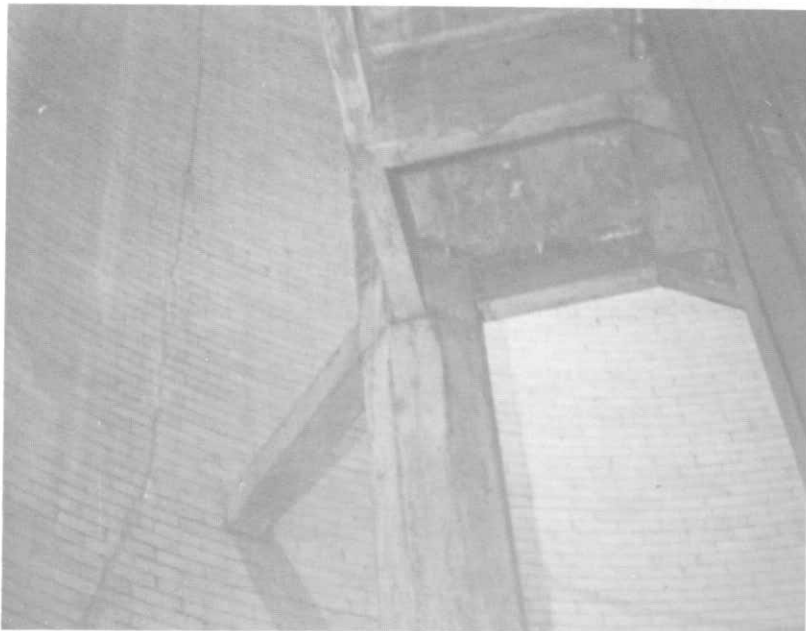
ILLUSTRATION 56. General view of brick crack in north quadrant of column shaft at approximately level 7.
