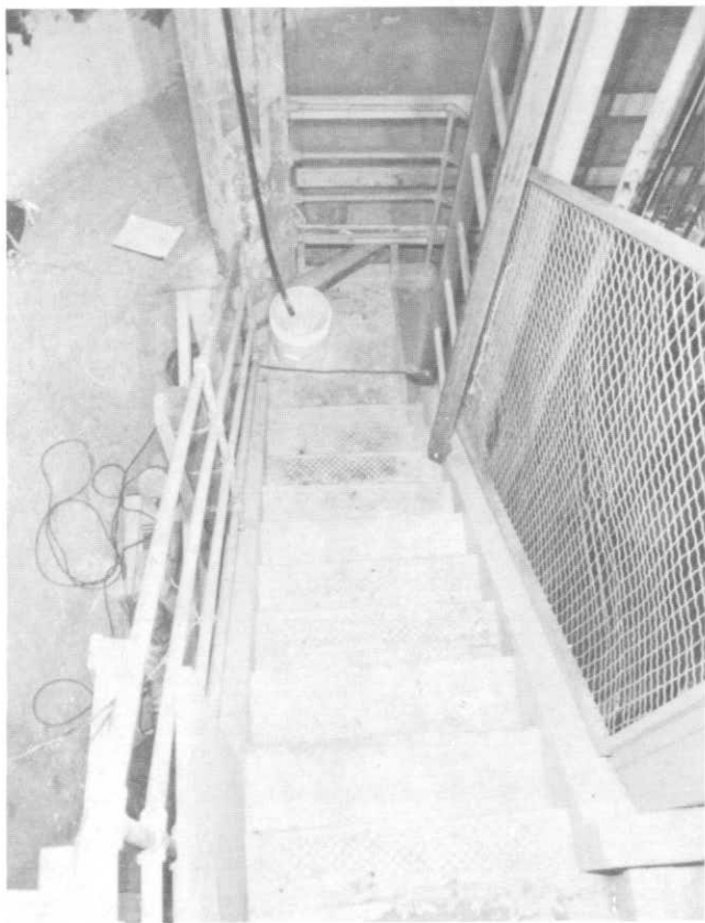
ILLUSTRATION 37. View of uppermost stair run and platform showing replacement safety tread and treads with cement wash only.
