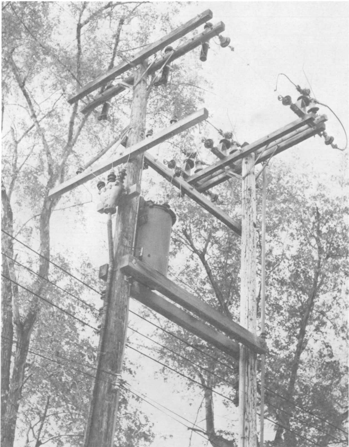
1. OHIO EDISON SERVICE The pole farthest from the transformer is in poor condition and should be replaced.
