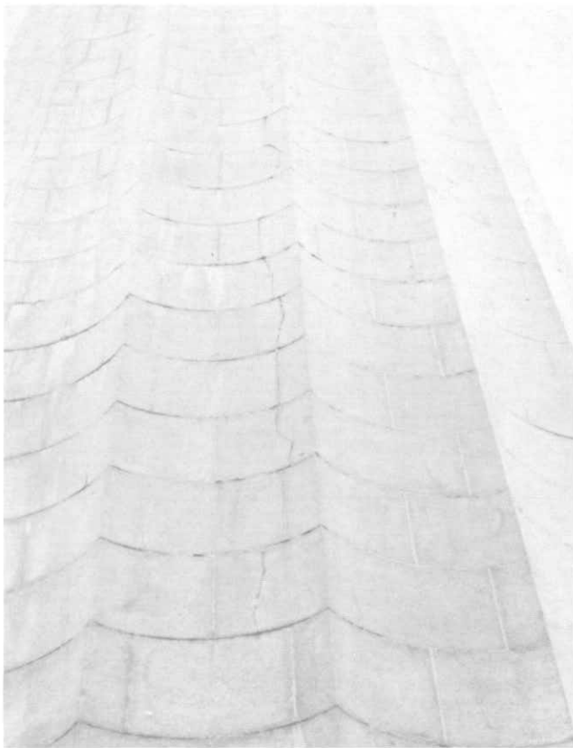
ILLUSTRATION 31. Overview of lower part of southwest side of column showing extent of major crack at flute M, courses 10 through 23.
