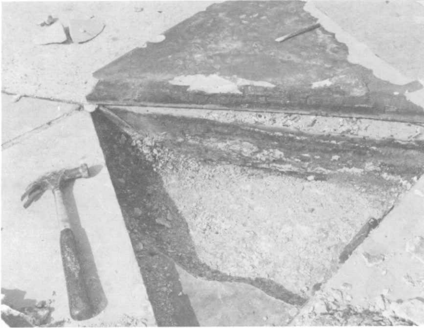
ILLUSTRATION 108. Detail view of edge of granite paver at foot of column. Note lack of waterproofing on the top of the slab.
