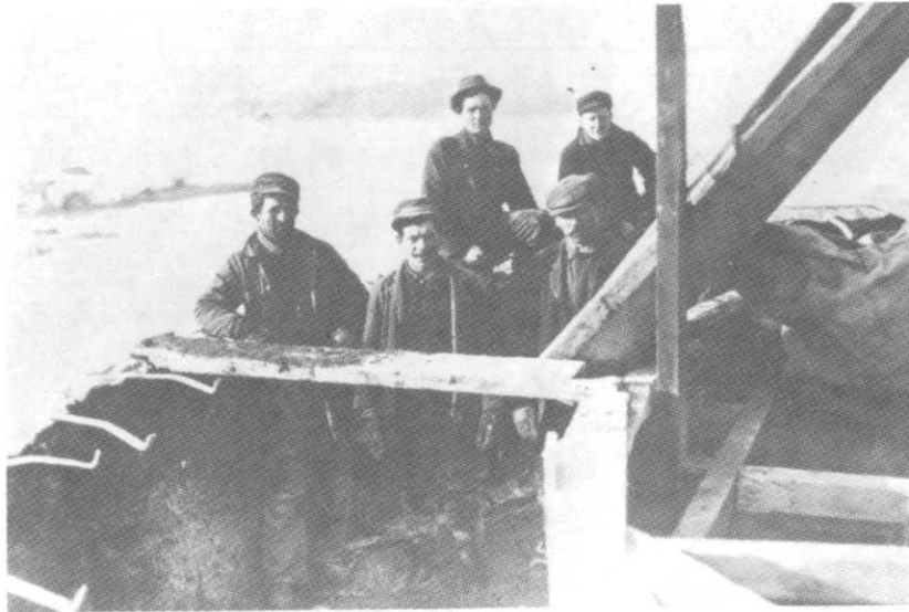
ILLUSTRATION 8. Memorial column construction progress, Aug. 15, 1913. Indiana Limestone framing interior doors and wall slabs of rotunda in place. Workman setting iron strap under granite block of partially completed fourth ("D") course of granite.
