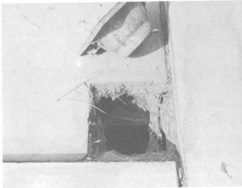
ILLUSTRATION 215. Close-up of floor drain serving the upper plaza surface.
