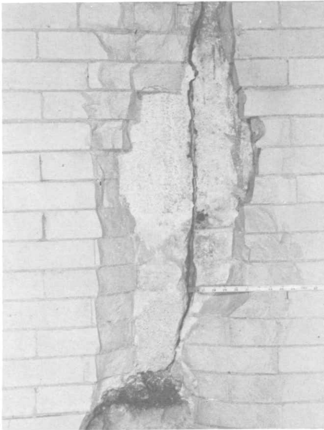
ILLUSTRATION 48. Detail view similar to Illustration 47, above, but also showing chunk of wood embedded in concrete which is an example of foreign matter which may be a cause of brown stains.
