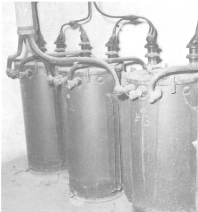
ILLUSTRATION 228. Main transformer bank. Note: Terminals in front should be tape insulated.
