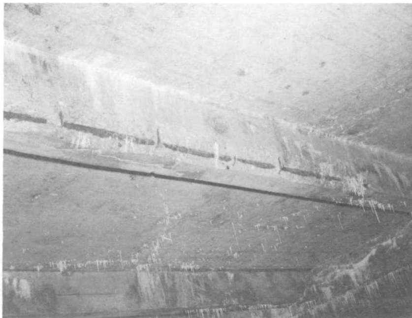
ILLUSTRATION 128. View of a typical beam after rust has caused concrete to spall.
