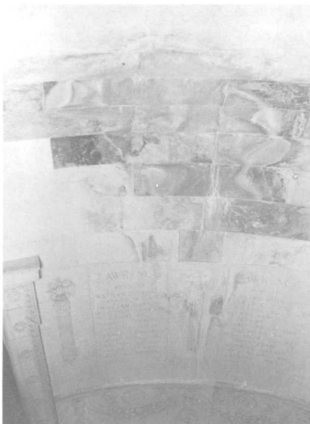
ILLUSTRATION 177. Detail view of stained limestone blocks and memorial engravings on southwest wall of rotunda.
