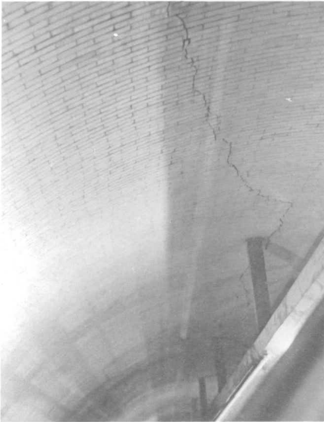
ILLUSTRATION 42. Typical view looking down column shaft showing octagonal column and column bracing into brick wall.
