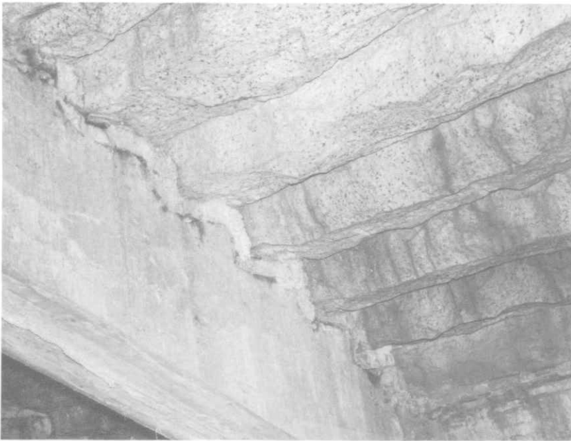
ILLUSTRATION 144. Detail view at underside of granite stair showing sloped and stepped support beam.
