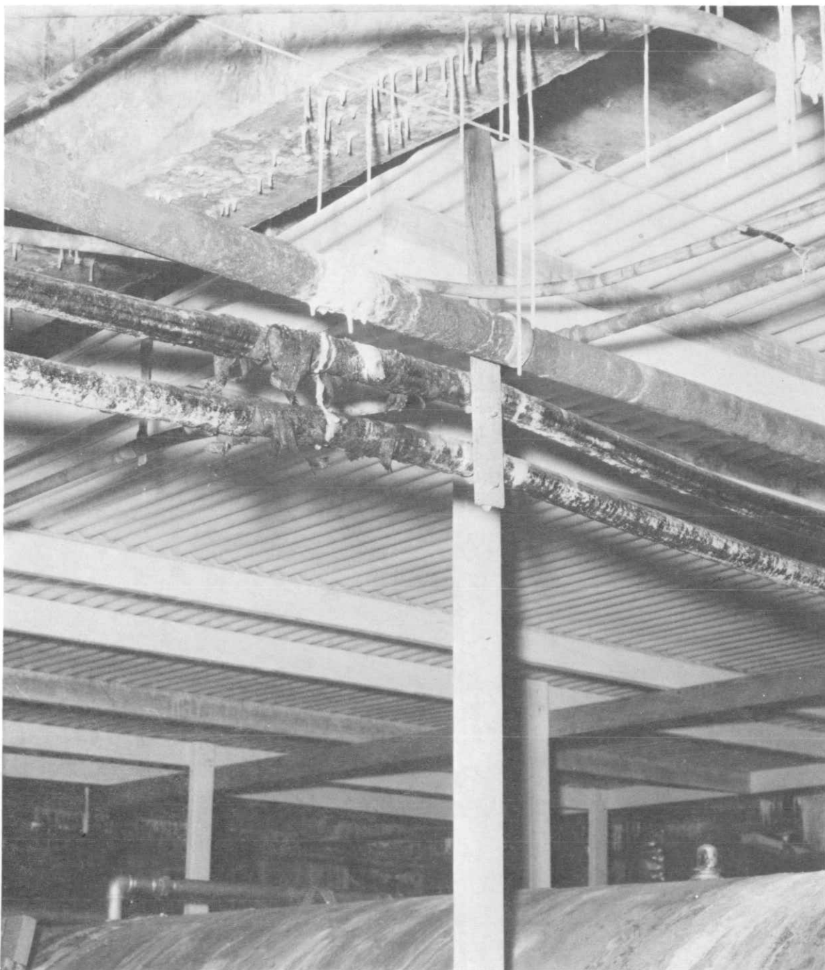
9a. BASEMENT CABLE The cables for floodlighting, elevator, and interior lighting are inadequately supported and exposed to damage and high stress concentrations at the support point. A cable tray and conduit system should be installed to continuously support these circuits. As an alternative, a stress spreading support plate should be installed at all attachment points. The outer jacket should be repaired with vinyl type tapes where the severe jacket damage and rotting are noted.
