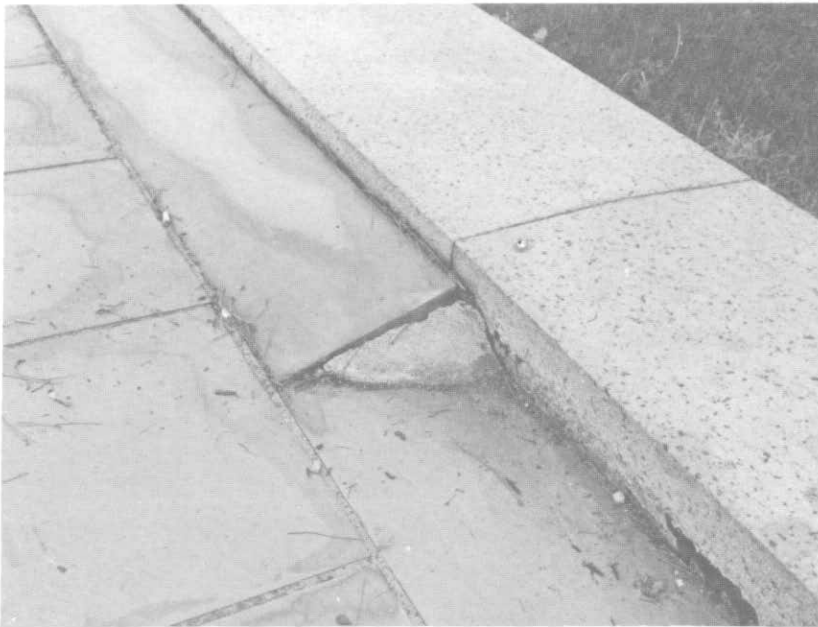
ILLUSTRATION 149. Detail view at east edge of lower plaza showing inclined pavers and flat pavers. Note rough cut of bottom edge of curbstone.
