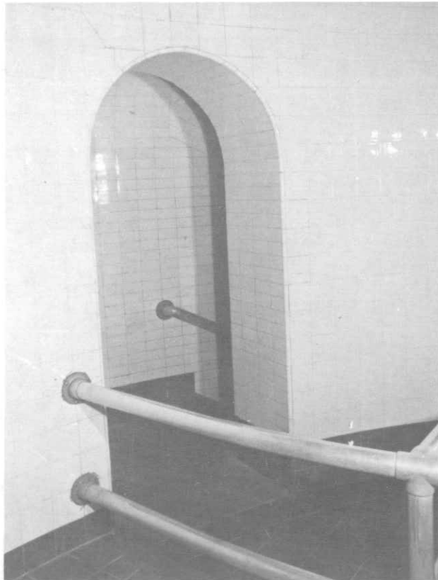
ILLUSTRATION 66. View of the top of the entrance granite stairs at the upper elevator landing showing the bronze railing.
