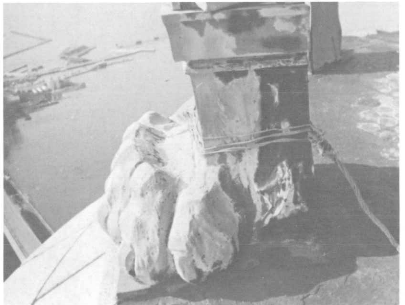
ILLUSTRATION 244. Typical (unacceptable) grounding of lantern base.
