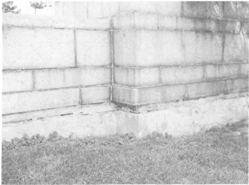
ILLUSTRATION 157. Partial view of southeast corner of retaining wall and lantern base. Note condition at intersection of concrete and granite.
