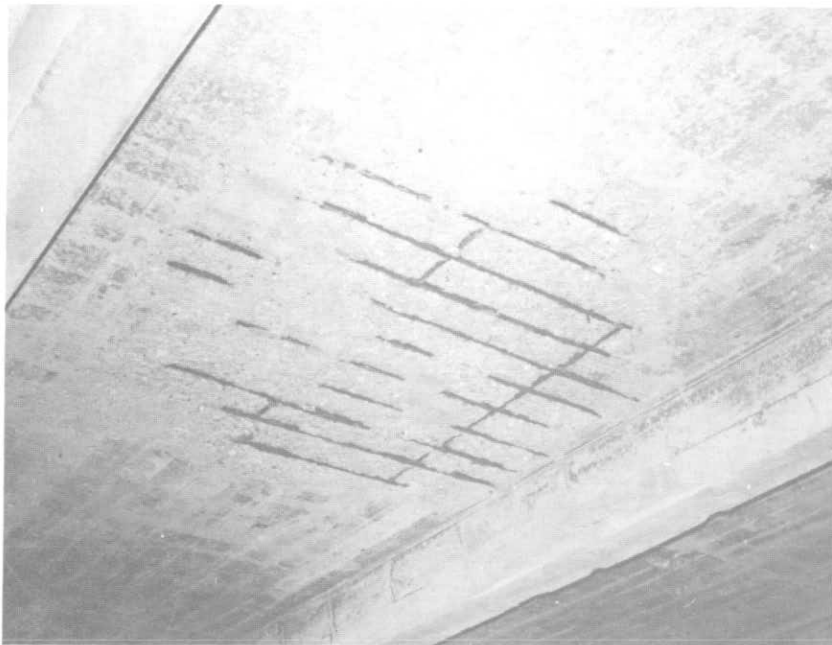
ILLUSTRATION 111. View of underside of upper plaza slab showing rusting condition of steel and spalled concrete.
