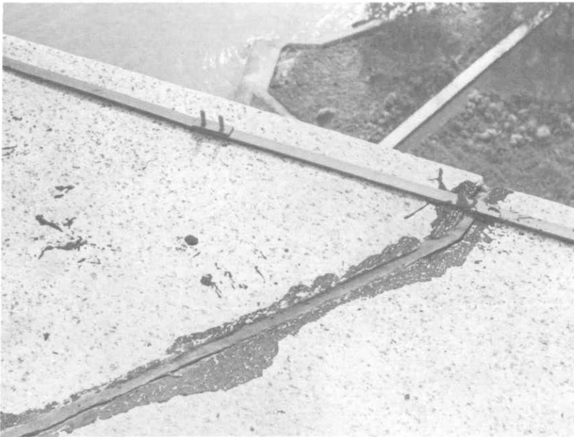
ILLUSTRATION 85. Detail of typical joint indicating improper removal of previous sealant prior to installation of new sealant. Metal bar is part of the lightning grounding system.
