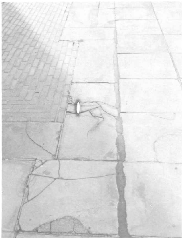
ILLUSTRATION 130. General view at northeast quadrant of upper plaza showing deteriorated joints, cracked and spalled sandstone pavers and brick paving inlay pattern.
