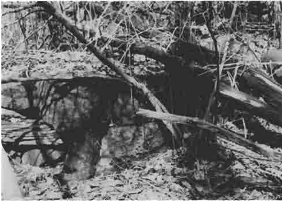
Photograph (47) Remains of the upper end of the guard bank at dam 4 at mile 97.5
