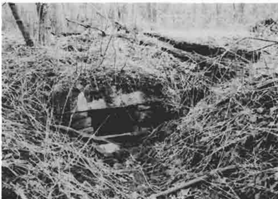
Photograph (64) A well preserved flat lintel stone towpath culvert at mile 23.1 below Hollidaysburg
