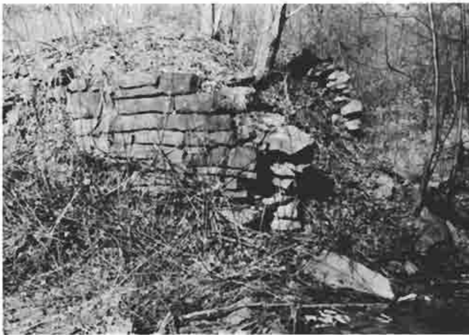
Photograph ⑥ Remnant of the Flat Run towpath bridge west abutment at mile 47.5
