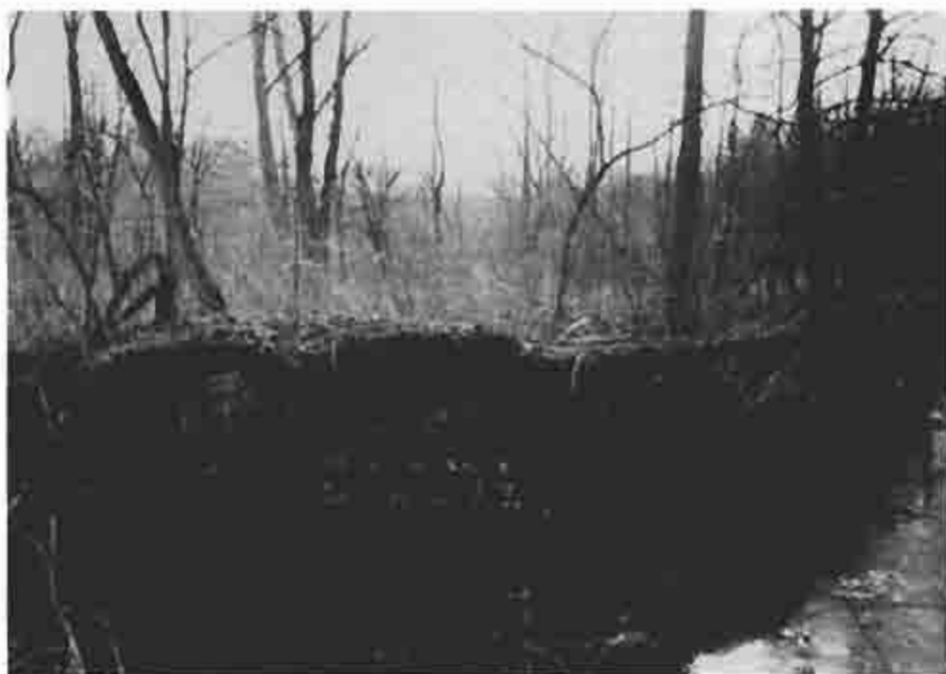
Photograph (58) Remnant of a wing wall and abutment at Small Aqueduct at mile 20.45 below Hollidaysburg
