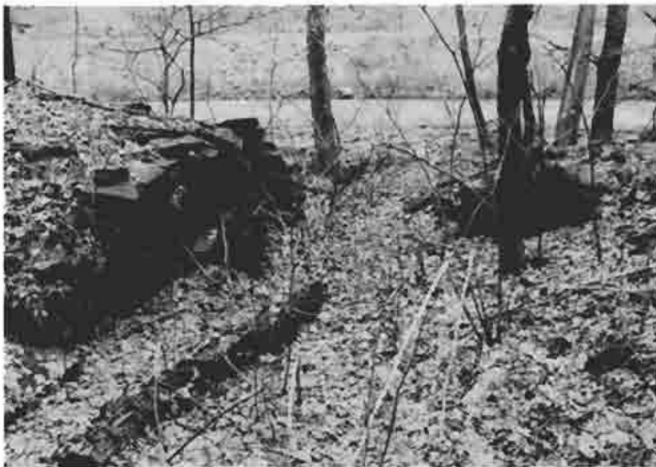
Photograph (42) Remains of the waste gate at the lower end of lock 8 at mile 81.0
