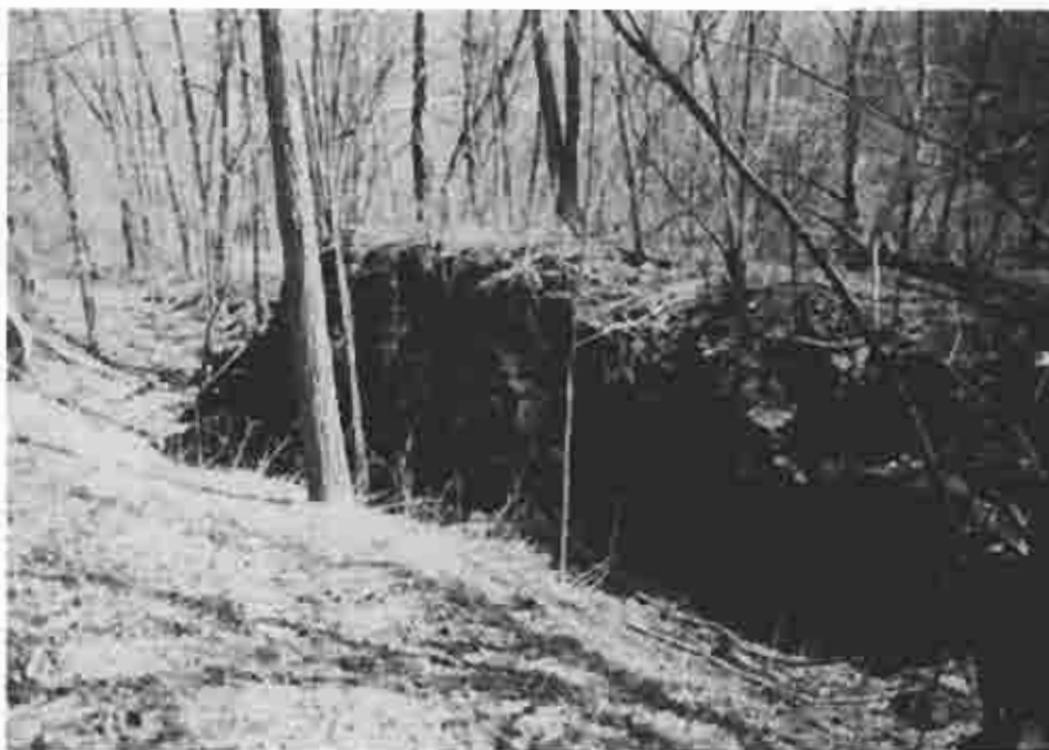
Photograph (55) Remnant of the south wall of guard lock 25 at Schmucker's Dam at mile 17.6 below Hollidaysburg
