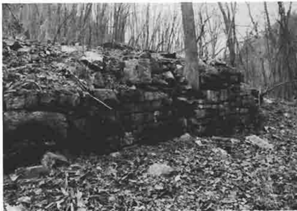
Photograph (65) Crumbling stone remains of the Little Water Street Dam northwest abutment at mile 24.1 below Hollidaysburg
