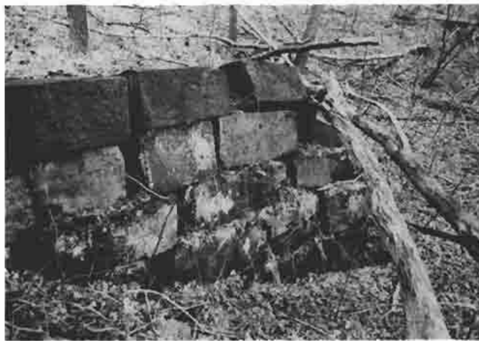
Photograph (40) Remains of the revetment wall above guard lock 2 and the dam at mile 79.15
