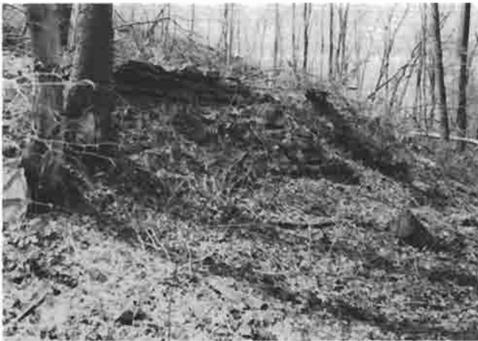
Photograph (36) Remains of a revetment wall at mile 78.45
