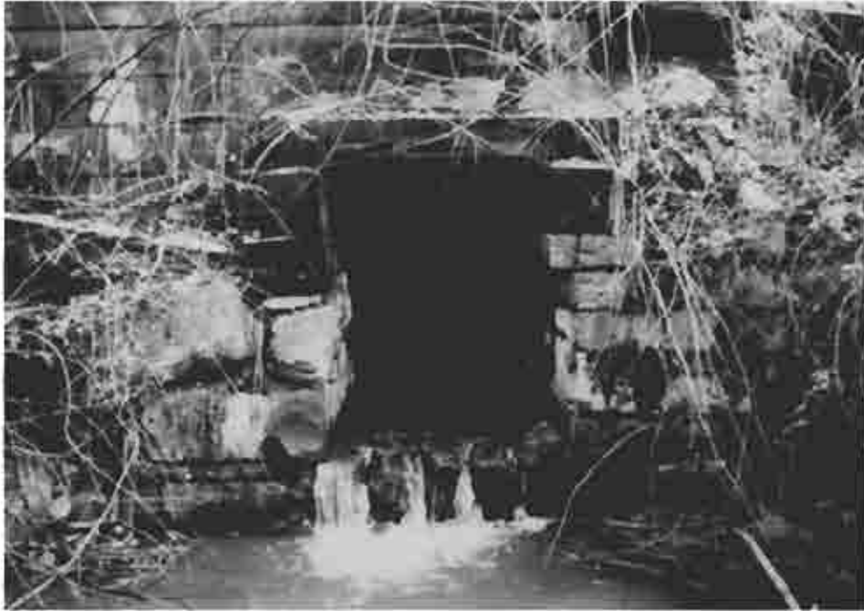
Photograph ① The lower end of the culvert at mile 30.05. The arched canal culvert is visible inside a larger railroad culvert
