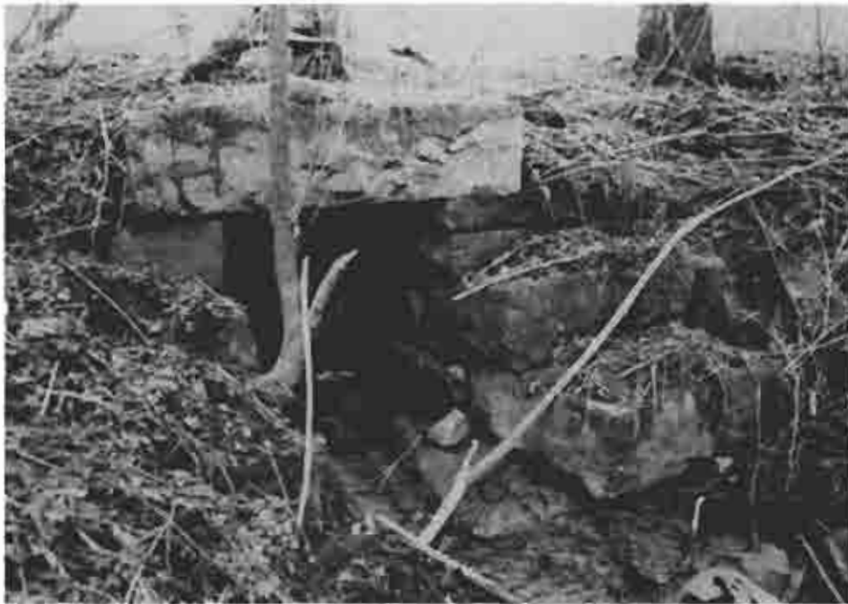
Photograph (63) A well preserved flat lintel stone towpath culvert at mile 22.9 below Hollidaysburg
