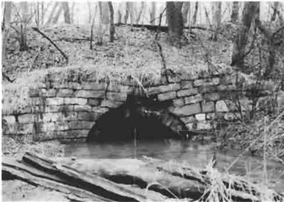
Photograph (45) Partly collapsed end of the Reed's Run canal culvert at mile 85.2
