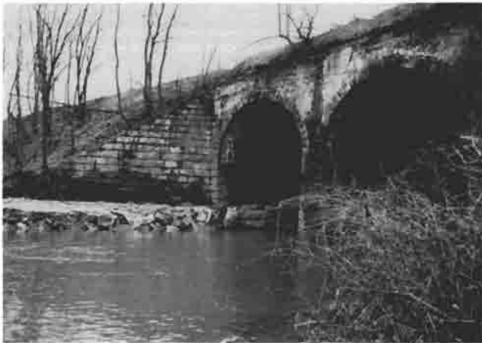
Photograph (43) Remains of the Tubmill Creek aqueduct east abutment at mile 81.95 which has been incorporated into a later railroad bridge
