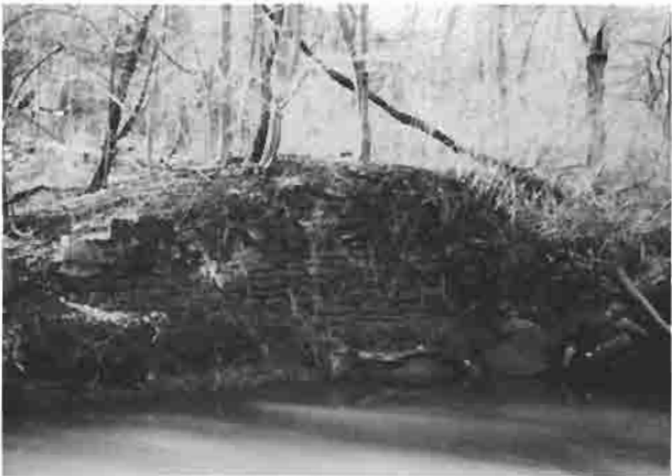
Photograph (26) Remains of the west abutment of the McGee Run towpath bridge at mile 74.2
