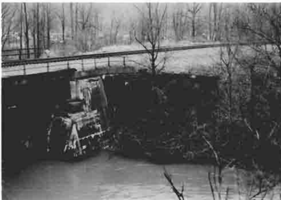
Photograph (44) Remains of the Lockport aqueduct wing walls and abutments at mile 84.0 which have been incorporated into a later railroad bridge
