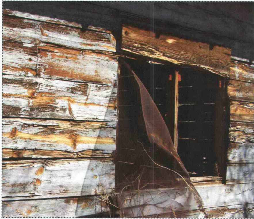
M, A, B. Detail view of window on west elevation. Note the wire mesh screen coming off & new board above opening
