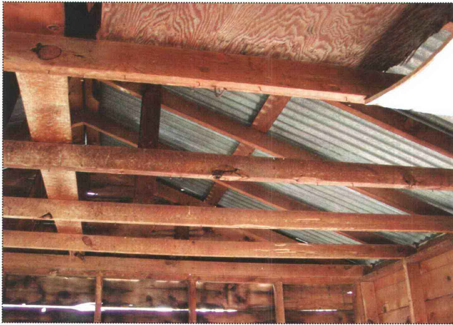
View of the roof trusses. Note the relatively new metal sheeting on the roof
