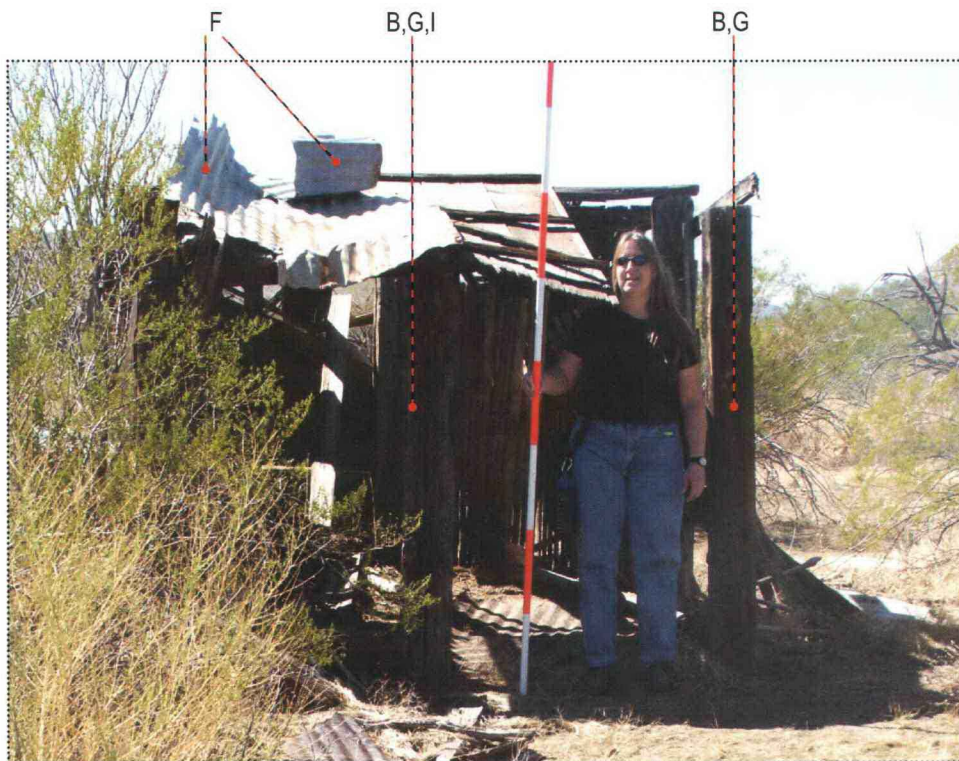
East elevation of the Ocotillo Shed (Letters refer to notes in condition assessment table ahead)
