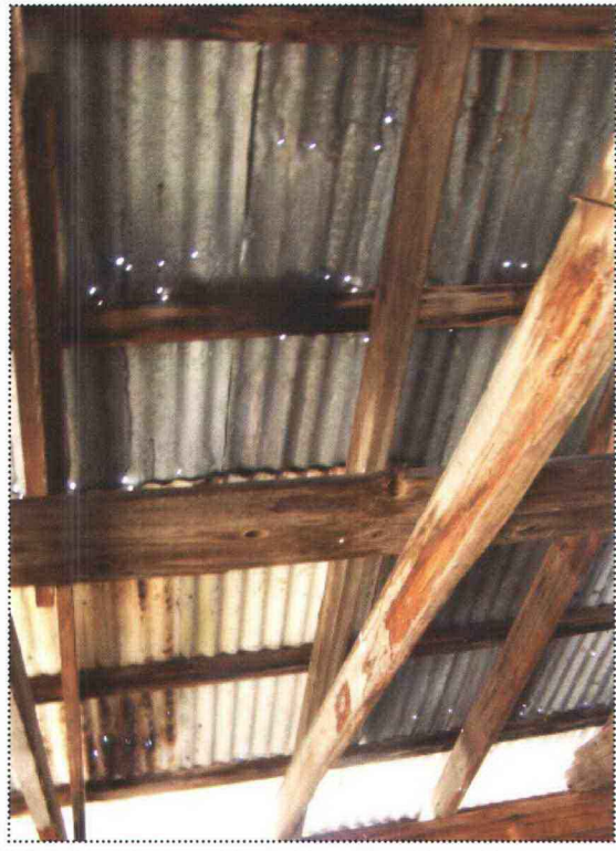
E. Detail view of metal roofing from the interior. Notice the rusting of sheets.
