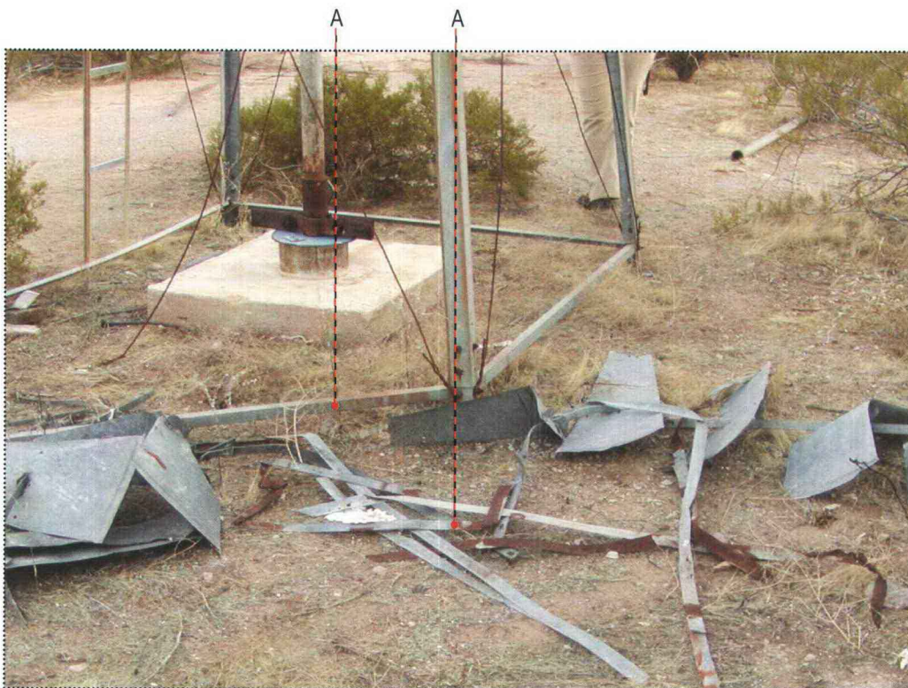
Base of Windmill 1 with associated debris (letters refer to notes in condition assessment table below)
