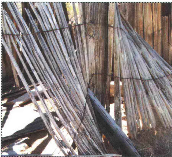
The failure of the saguaro rib cladding
