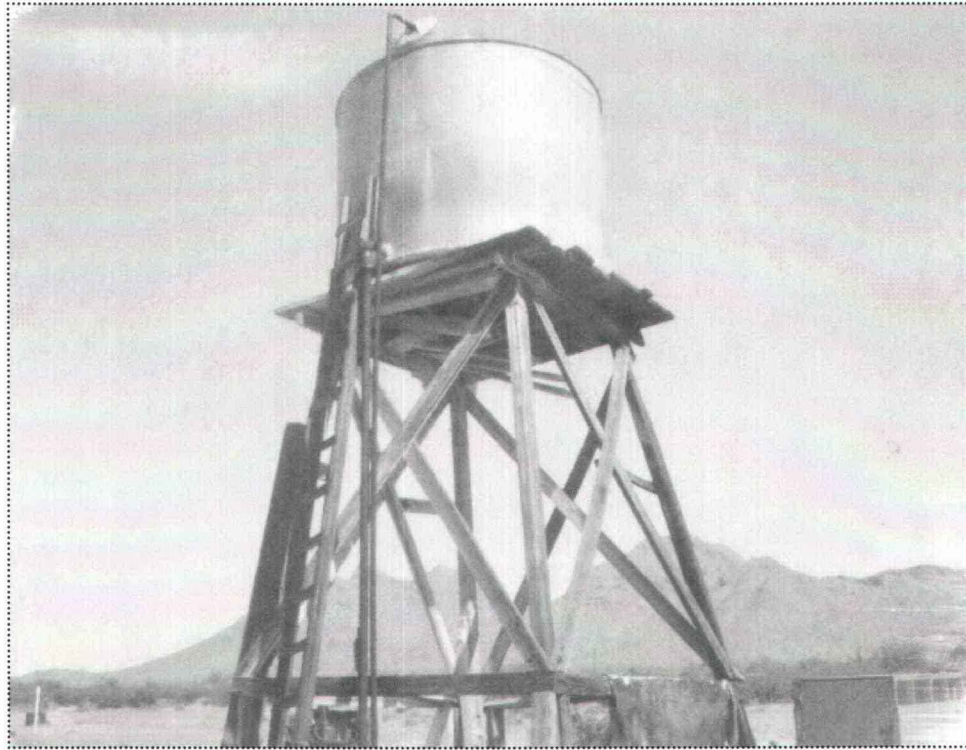
Bates Well water tower, May 1979, Organ Pipe Cactus NM Photo Archive No. 614
