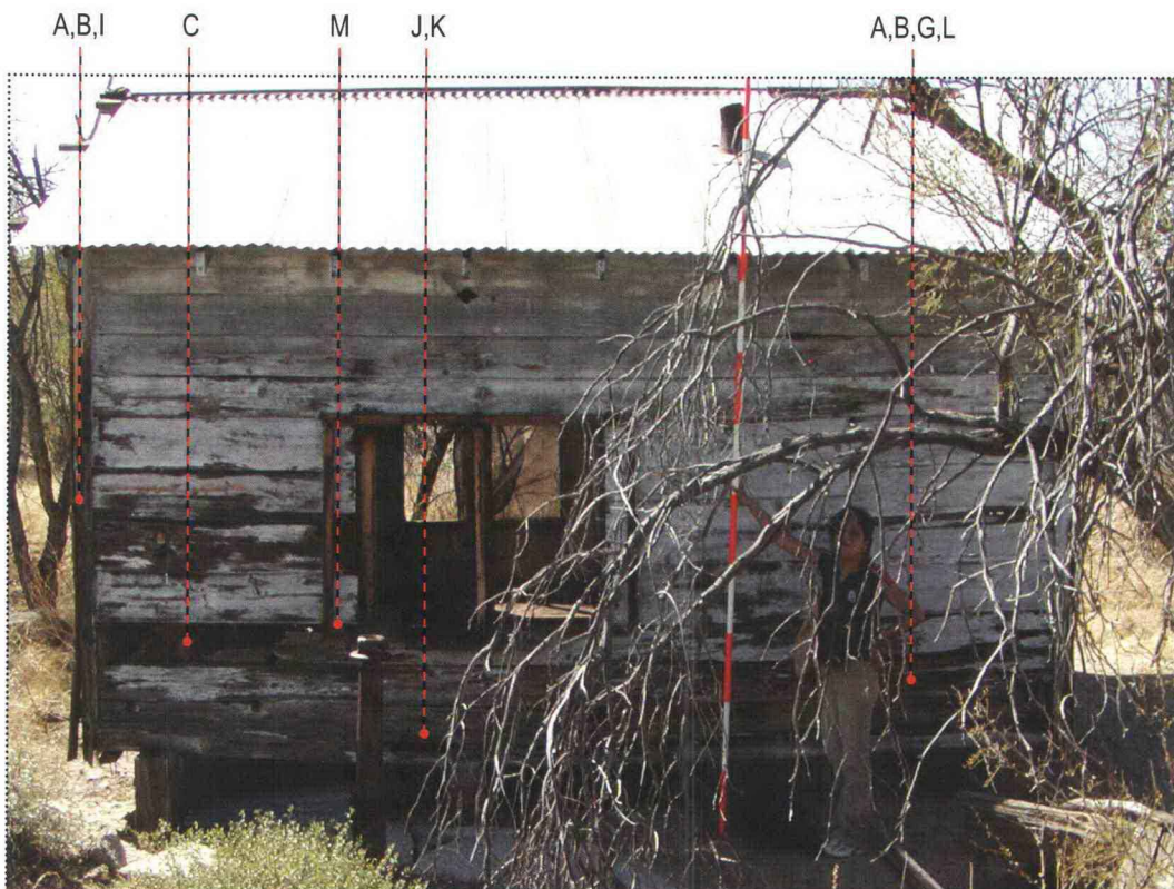
East elevation of the Bunkhouse (Letters refer to notes in condition assessment table below)
