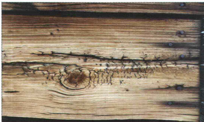
B. Rotting of wood due to microorganisms/ pests (also termite) infestation.
