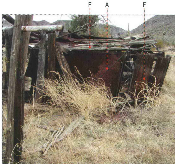
West elevation of Blacksmith Shop (letters refer to notes in condition assessment table below)
