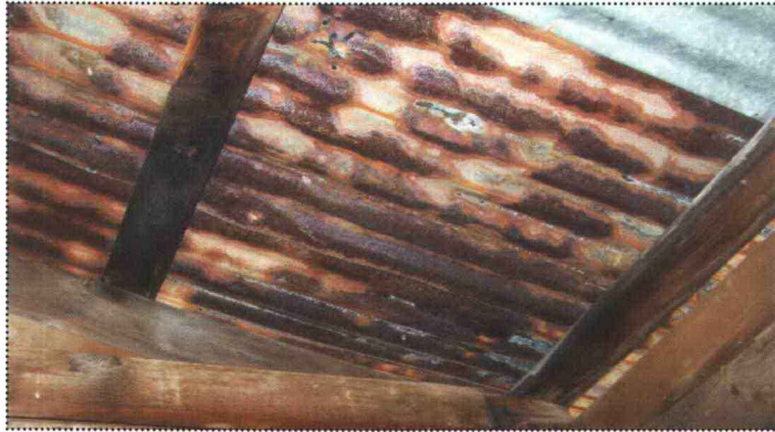
E. Rusting of the corrugated metal roof due to water damage
