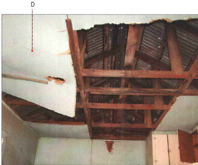
Interior Ceiling of the Main Residence (letters refer to notes in condition assessment table below)
