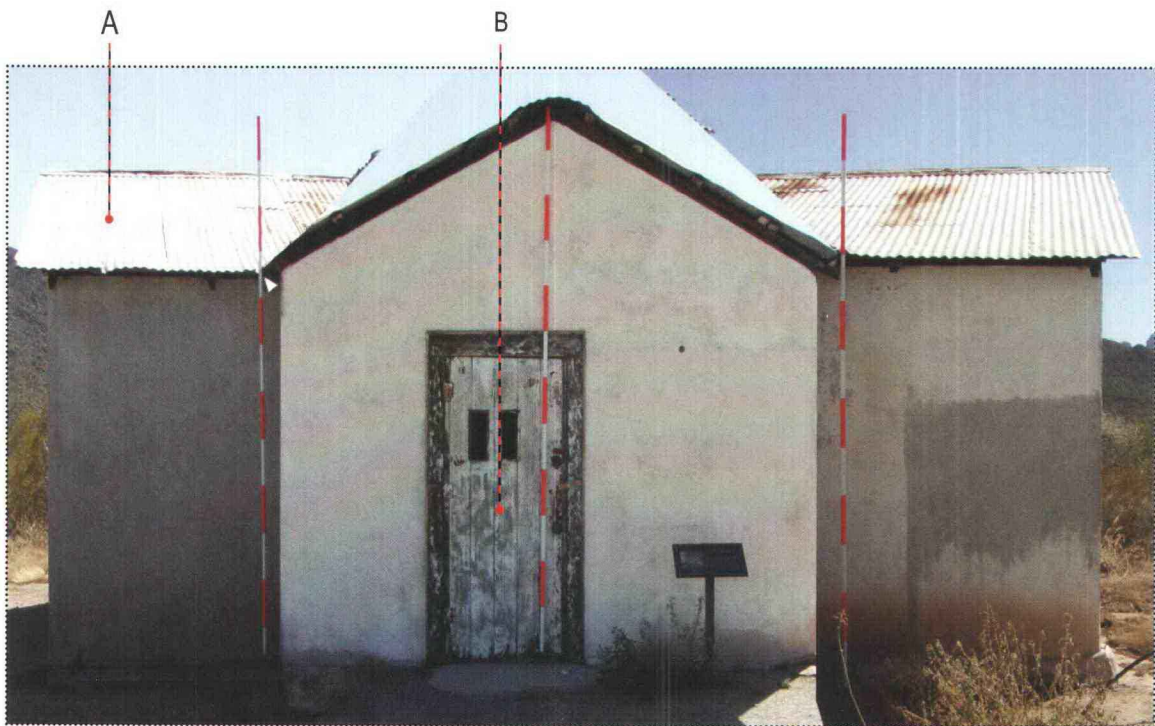
North elevation of the Main Residence (letters refer to notes in condition assessment table below)
