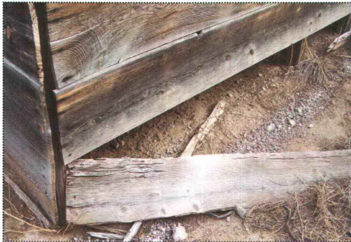
J. Falling apart of the wooden planks near the base of the structure.
