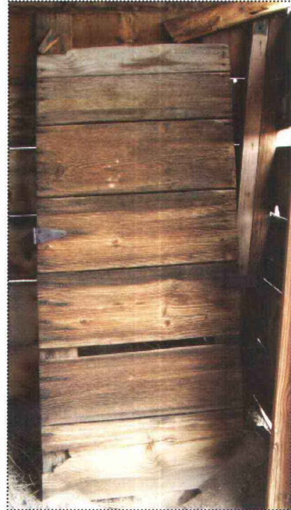
H. Dis-hinged entrance door lying inside the structure.
