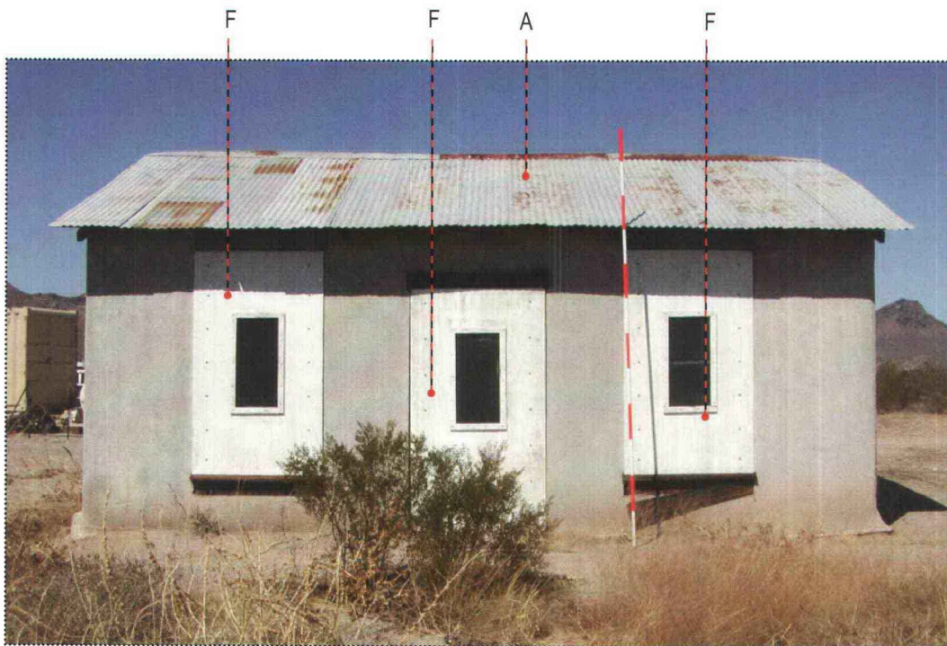
South elevation of the Main Residence (letters refer to notes in condition assessment table below)
