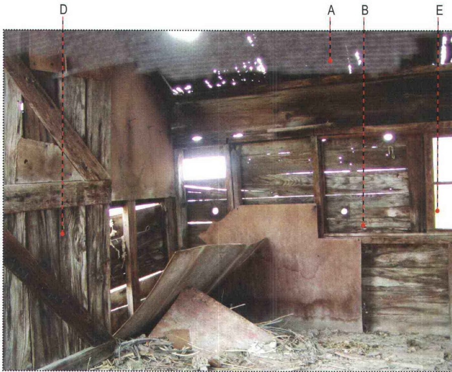
Interior elevation of the Small Residence (letters refer to notes in condition assessment table below)
