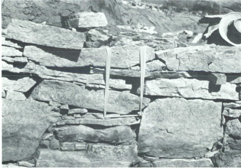
Figure 24. The east wall of Structure 1 before stabilization with a soil epoxy mortar.
