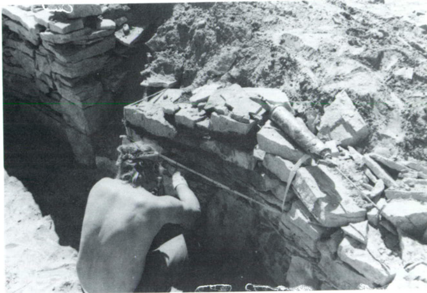
Figure 16. The south wall of Structure 1 after stabilization using an unamended mud mortar.
