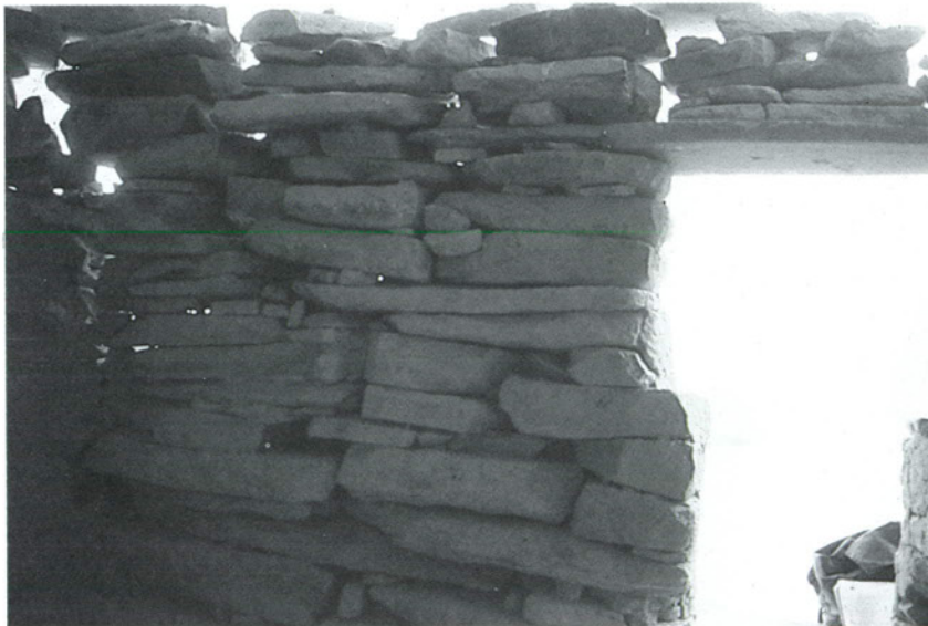
Figure 34. The interior wall of the In-and-Out House (42Ka595) reveals a much less stable configuration than the exterior, since the interior retains less mortar. This mortar was replaced with both soil epoxy and calcium-aluminate soil cement.
