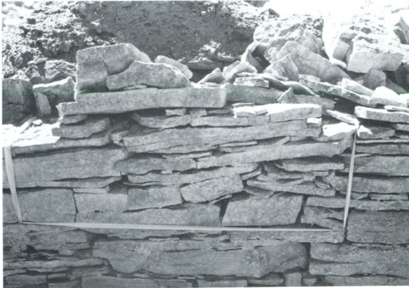
Figure 23. The west wall of Structure 2 after inundation, but before stabilization with a soil-calcium aluminate cement mortar. Compare the wall height with that in Figure 48.
