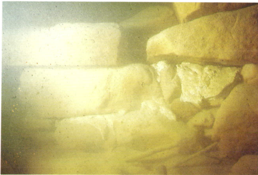
Figure 36. The resultant remortared area of the wall is best shown at the area designated by the arrow. This photograph was taken three months after the application.
