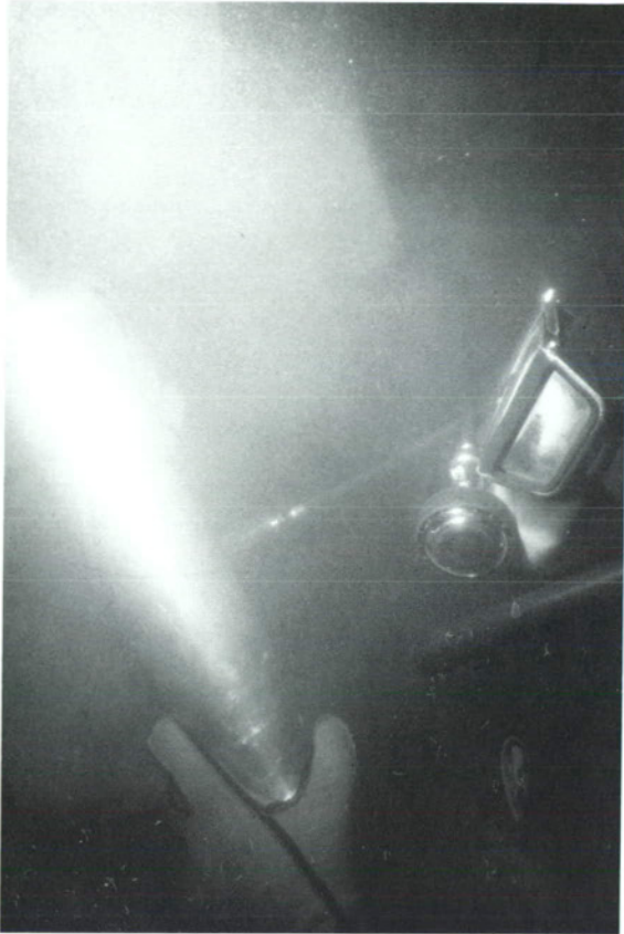
Figure 35. At a depth of ca. 17 meters, a handheld grout gun was used to replace mortar which had been eroded when the site went underwater.
