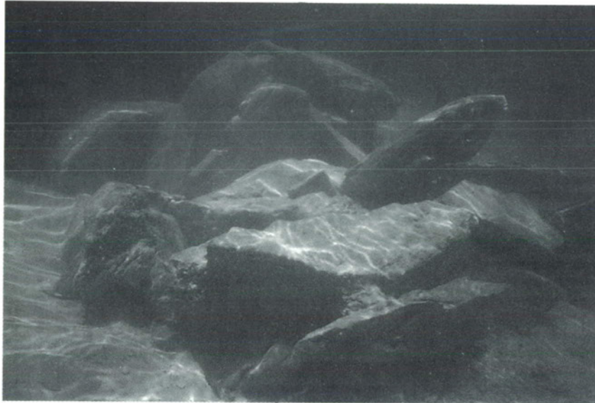
Figure 32. The remains of some of the masonry material which fell are shown here, at a depth of 1.5-2.0 meters. This portion fell as a monolith, with some of the soil epoxy mortar (shown at the arrow) still bonding the stones together.
