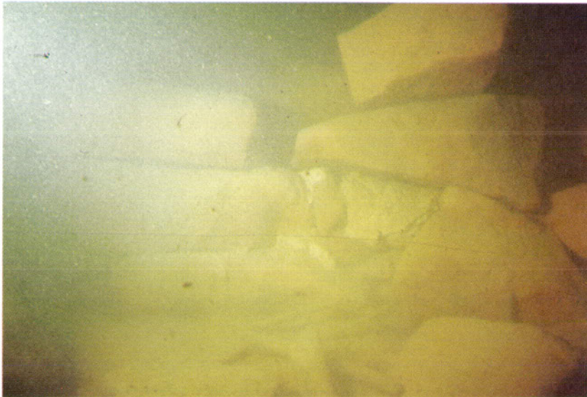
Figure 29. The section of masonry wall in Structure 4 after stabilization with soil epoxy mortars.
