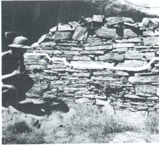
Figure 22. The west wall of Structure 2 before inundation. White line indicates the extant wall height following unundation. Photo courtesy of the University of Utah.
