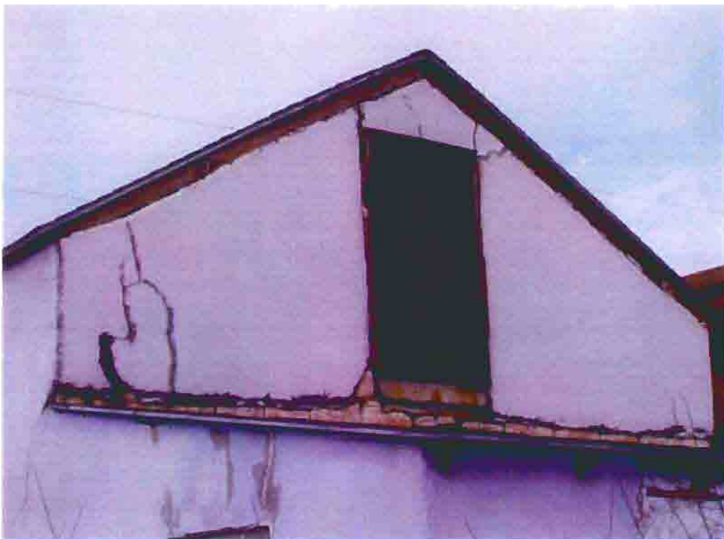
Photo F-18. The Fletcher-Switzer House, cracks at the second floor window, February 2001. Photo by Wiss, Janney, Elstner Associates, Northbrook, Illinois.
