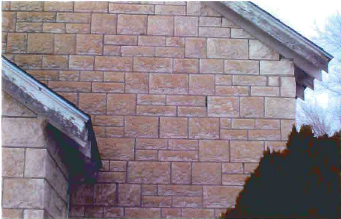
Photo T-13. The Township Hall, step cracking on the south wall, February 2001. Photo by Wiss, Janney, Elstner Associates, Northbrook, Illinois.
