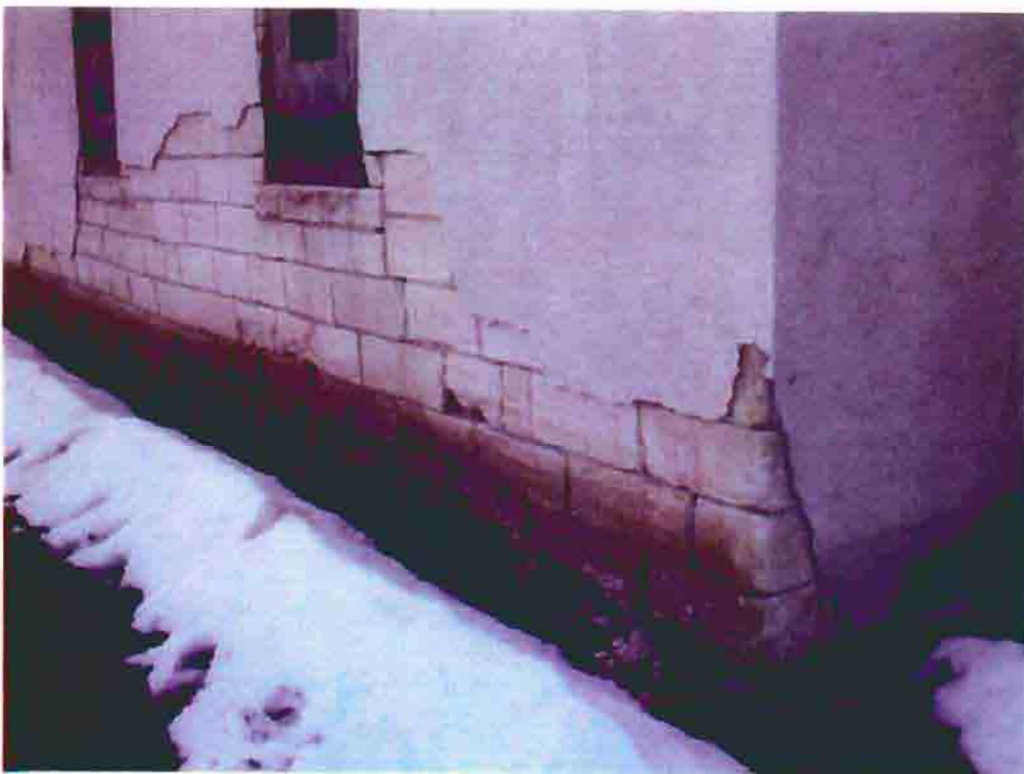
Photo A-20. The A.M.E. Church, failed stucco along the south wall, February 2001. Photo by Wiss, Janney, Elstner Associates, Northbrook, Illinois.
