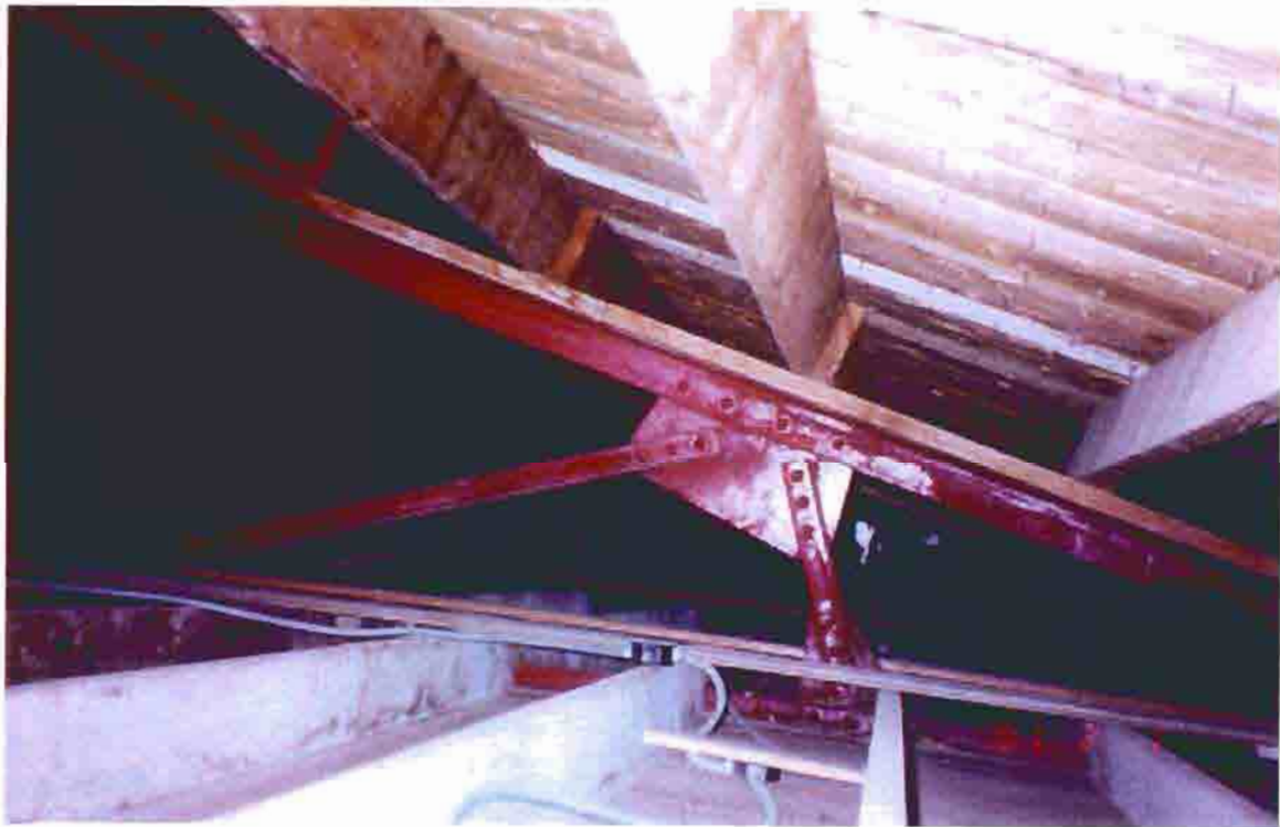
Photo T-24. Township Hall, view of roof structure above the main hall, February 2001. Photo by Bahr Vermeer Haecker Architects, Lincoln, Nebraska.
