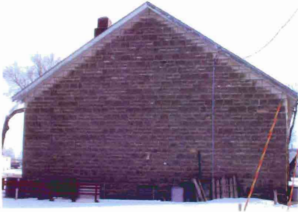
Photo T-11. The Township Hall, north elevation, February 2001. Photo by Wiss, Janney, Elstner Associates, Northbrook, Illinois.
