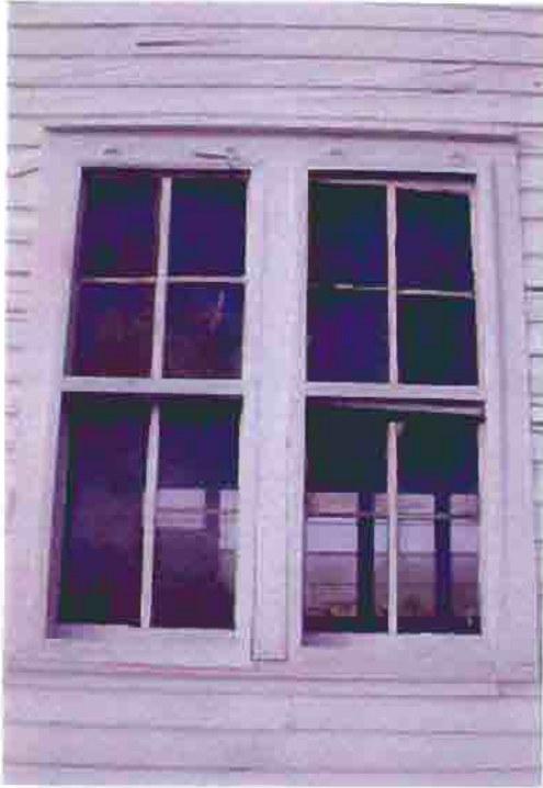
Photo S-17. The District No. 1 School, paired windows on the south elevation, February 2001. Photo by Wiss, Janney, Elstner Associates, Northbrook, Illinois.
