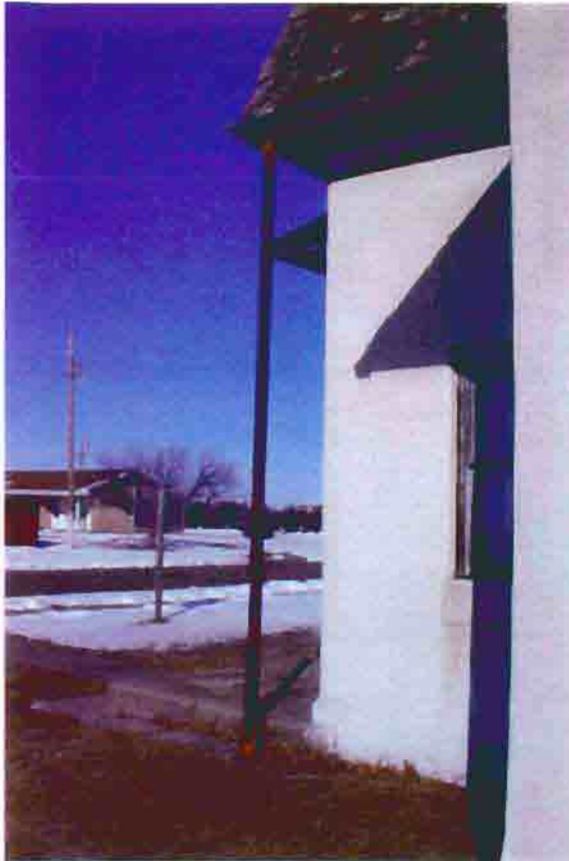
Photo B-19. The First Baptist Church, post at corner of vestibule, February 2001. Photo by Wiss, Janney, Elstner Associates, Northbrook, Illinois.
