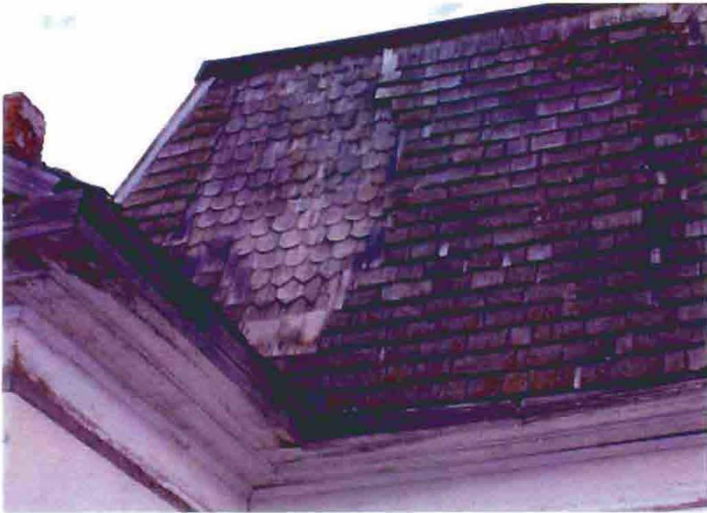
Photo B-15. The Old First Baptist Church, two layers of wood shingles on the vestibule roof, February 2001. Photo by Wiss, Janney, Elstner Associates, Northbrook, Illinois.
