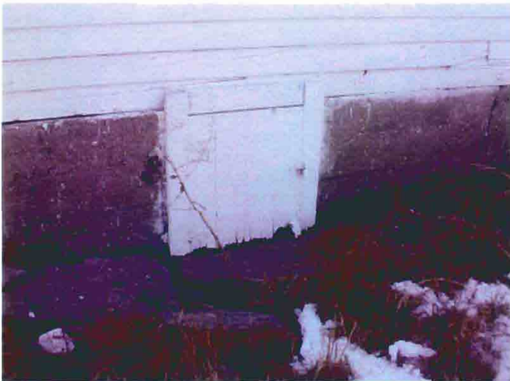
Photo S-20. The District No. 1 School, foundation access door, February 2001. Photo by Wiss, Janney, Elstner Associates, Northbrook, Illinois.
