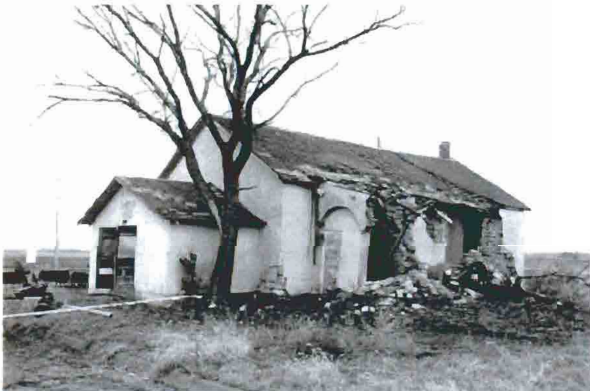
Photo A-10 The A.M.E. Church, view from the northeast, 1990s. The northeast vestibule and much of the north wall had collapsed. Photo from National Historic Landmark files.
