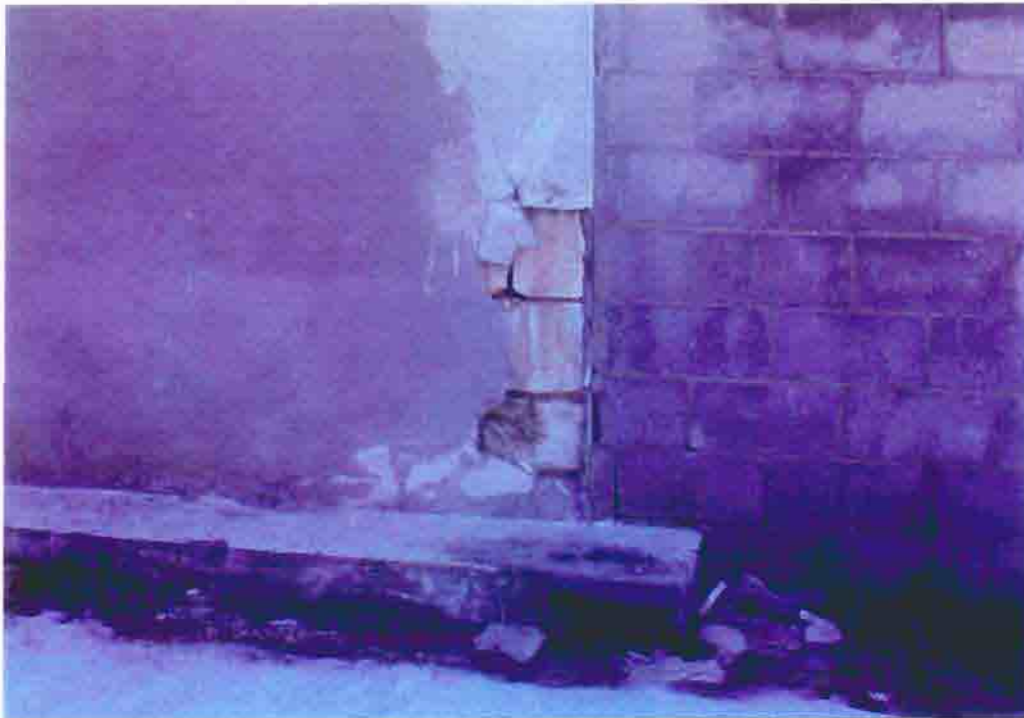
Photo B-16. The Old First Baptist Church, failed stucco on the north elevation, February 2001. Photo by Wiss, Janney, Elstner Associates, Northbrook, Illinois.
