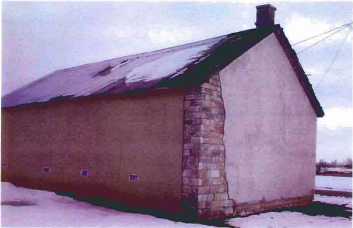
Photo A-13. The A.M.E. Church, view from the northwest, February 2001. Photo by Wiss, Janney, Elstner Associates, Northbrook, Illinois.
