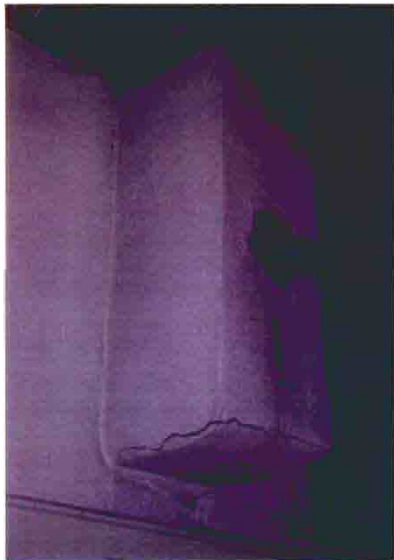
Photo B-24. The First Baptist Church, chimney in kitchen, February 2001. The chimney is suspended above the serving counter between the sanctuary and kitchen. Photo by Wiss, Janney, Elstner Associates, Northbrook, Illinois.
