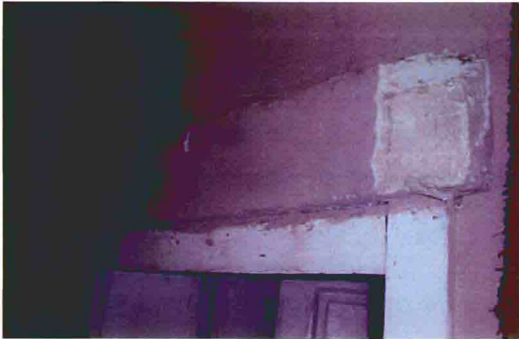
Photo F-23. The Fletcher-Switzer House, cracked stone lintel, February 2001. Photo by Wiss, Janney, Elstner Associates, Northbrook, Illinois.
