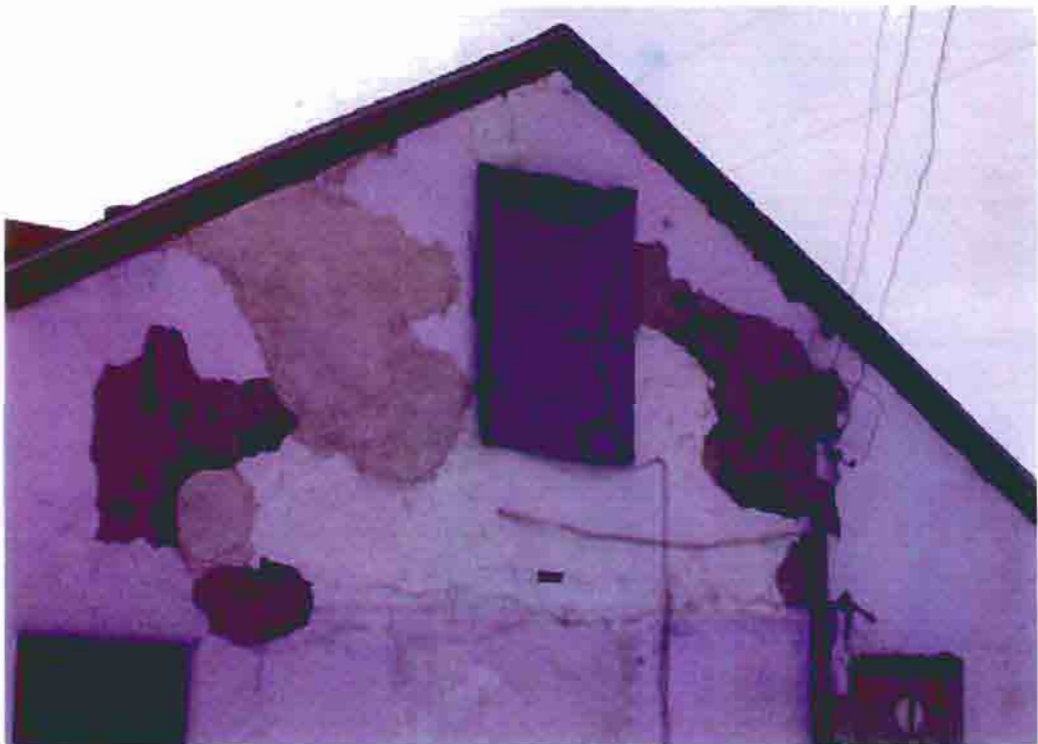
Photo F-14. The Fletcher-Switzer House, failed stucco on the east elevation, February 2001. Photo by Wiss, Janney, Elstner Associates, Northbrook, Illinois.
