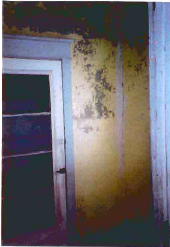
Photo S-25. The District No. 1 School, interior of the entry hall showing failing paint, cracked plaster, and the door to the kitchen, February 2001. Photo by Bahr Vermeer Haecker Architects, Lincoln, Nebraska.
