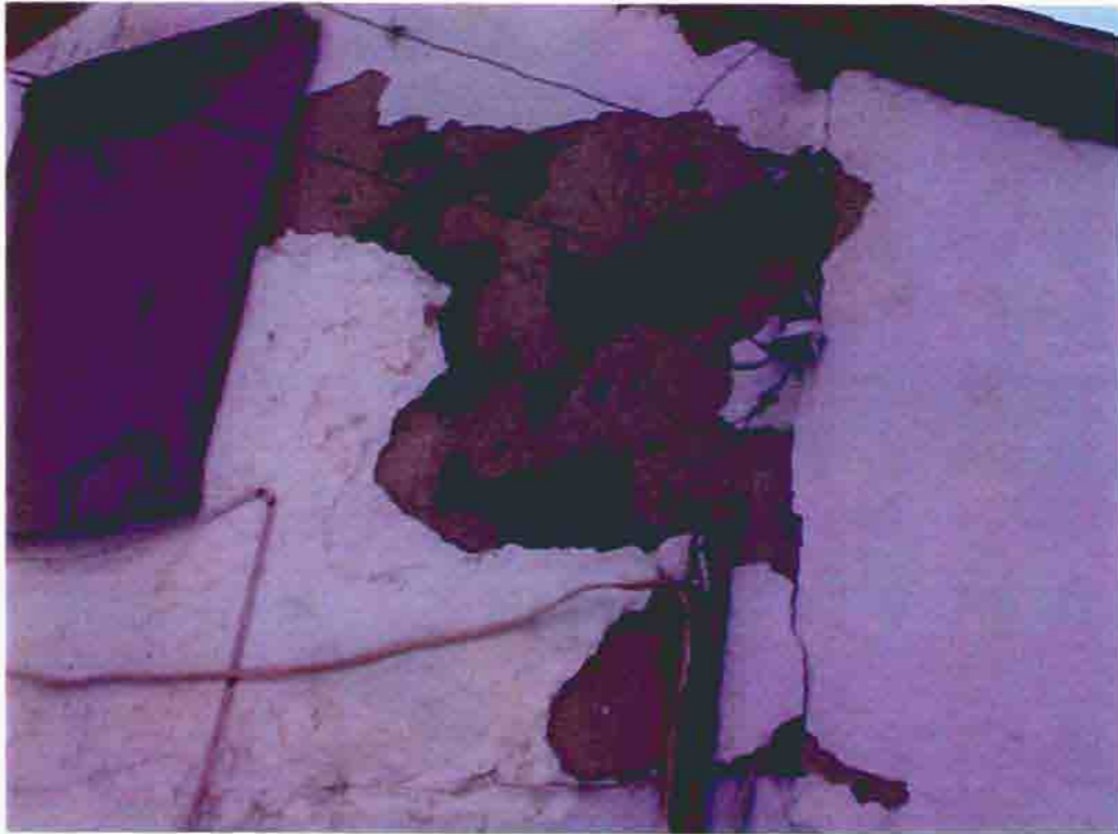
Photo F-15. The Fletcher-Switzer House, detail of failed stucco on the east elevation, February 2001. Photo by Wiss, Janney, Elstner Associates, Northbrook, Illinois.
