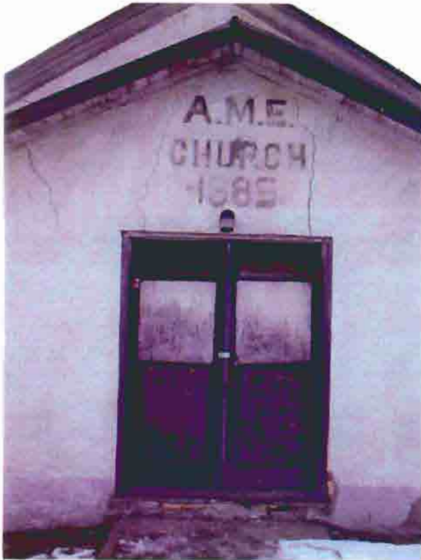
Photo A-19. The A.M.E. Church, east entrance, February 2001. Photo by Wiss, Janney, Elstner Associates, Northbrook, Illinois.
