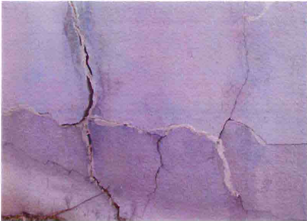
Photo F-17. The Fletcher-Switzer House, failing stucco, February 2001. Photo by Wiss, Janney, Elstner Associates, Northbrook, Illinois.
