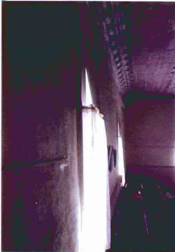
Photo B-21. The First Baptist Church, east wall out of plumb, February 2001. Photo by Wiss, Janney, Elstner Associates, Northbrook, Illinois.
