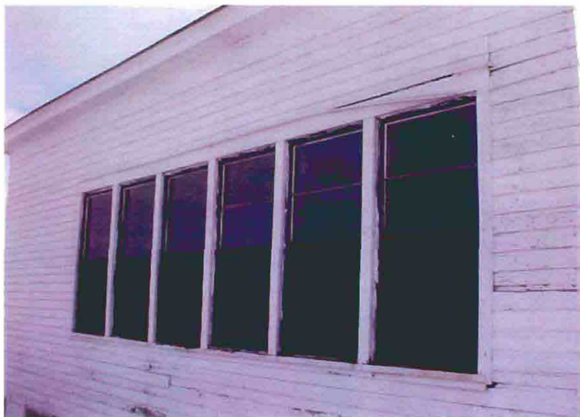
Photo S-12. The District No. 1 School, windows on the north elevation. February 2001. Photo by Wiss, Janney, Elstner Associates, Northbrook, Illinois.
