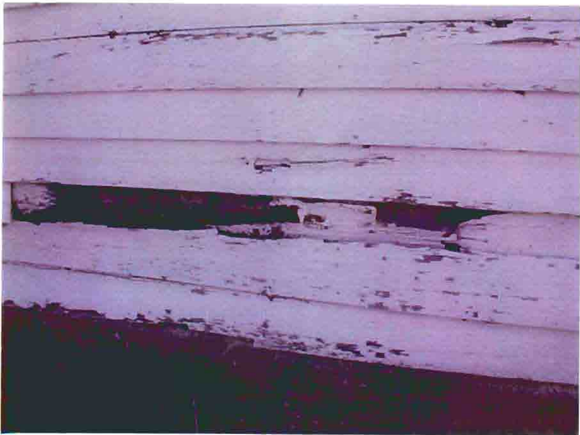
Photo S-18. The District No. 1 School, deteriorated wood siding, February 2001. Photo by Wiss, Janney, Elstner Associates, Northbrook, Illinois.
