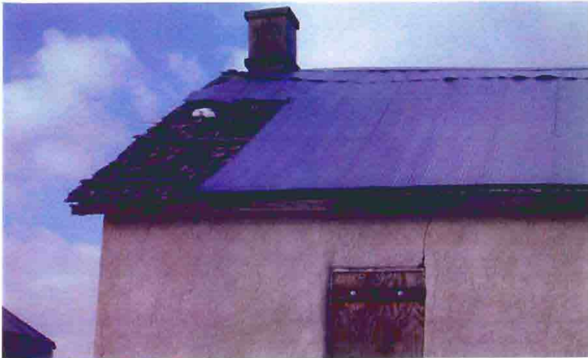
Photo A-17. The A.M.E. Church, missing metal at the west end of the roof, February 2001. Photo by Wiss, Janney, Elstner Associates, Northbrook, Illinois.
