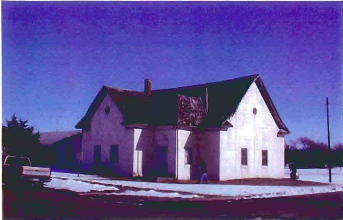
Photo B-13. The Old First Baptist Church, view from the southwest, February 2001. Photo by Wiss, Janney, Elstner Associates, Northbrook, Illinois.
