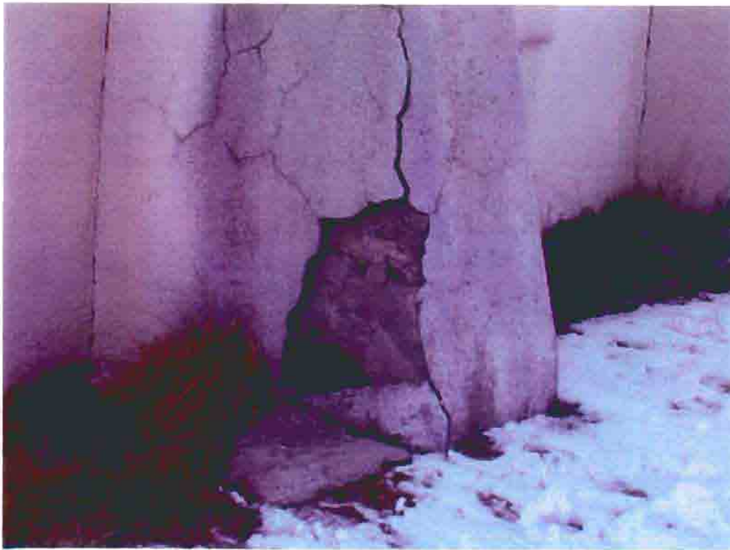
Photo B-18. The Old First Baptist Church, failed stucco on buttress, February 2001. Photo by Wiss, Janney, Elstner Associates, Northbrook, Illinois.
