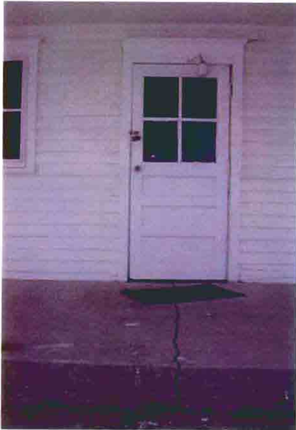
Photo S-13. The District No. 1 School, entrance door and cracked porch slab, February 2001. Photo by Wiss, Janney, Elstner Associates, Northbrook, Illinois.
