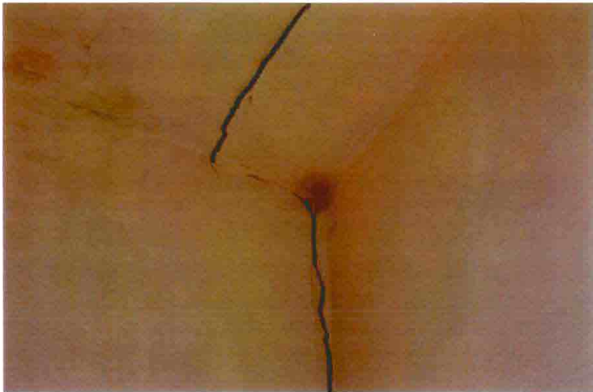
Photo S-24. The District No. 1 School, cracked plaster at wall/ceiling intersection, February 2001. Photo by Wiss, Janney, Elstner Associates, Northbrook, Illinois.
