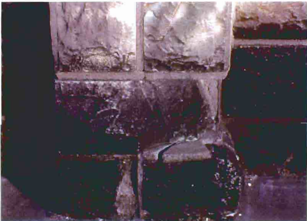
Photo T-16. The Township Hall, failed stone at the base of a butters, February 2001. Photo by Wiss, Janney, Elstner Associates, Northbrook, Illinois.
