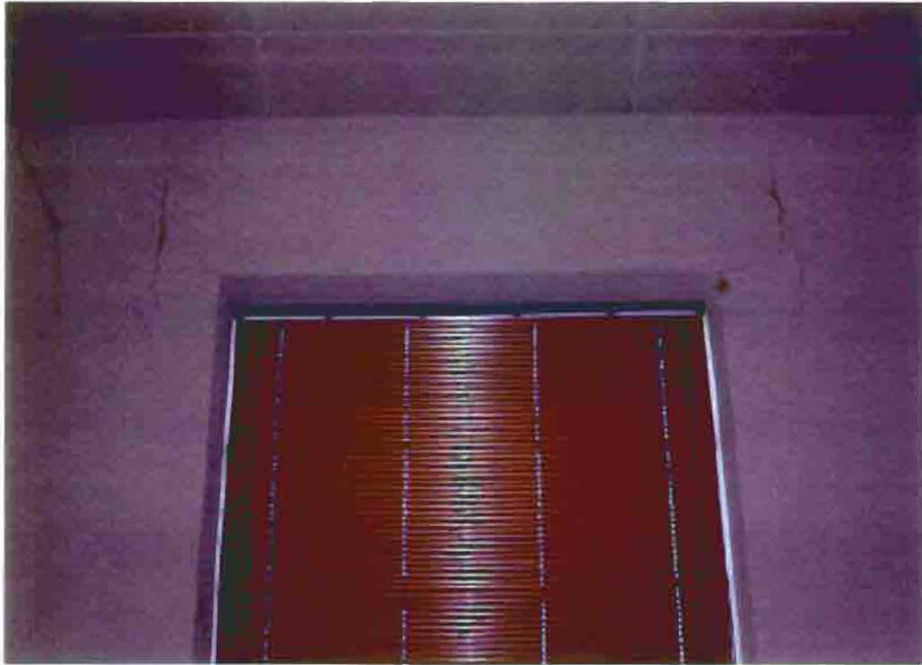
Photo T-19. The Township Hall, cracks in interior plaster around windows, February 2001. Photo by Wiss, Janney, Elstner Associates, Northbrook, Illinois.
