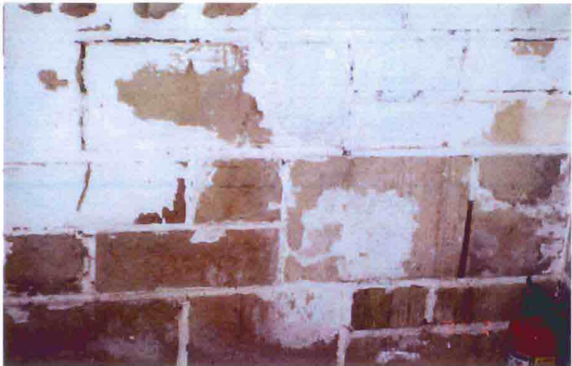
Photo T-25. Township Hall, detail of stonework in basement with failed paint, February 2001. Photo by Bahr Vermeer Haecker Architects, Lincoln, Nebraska.
