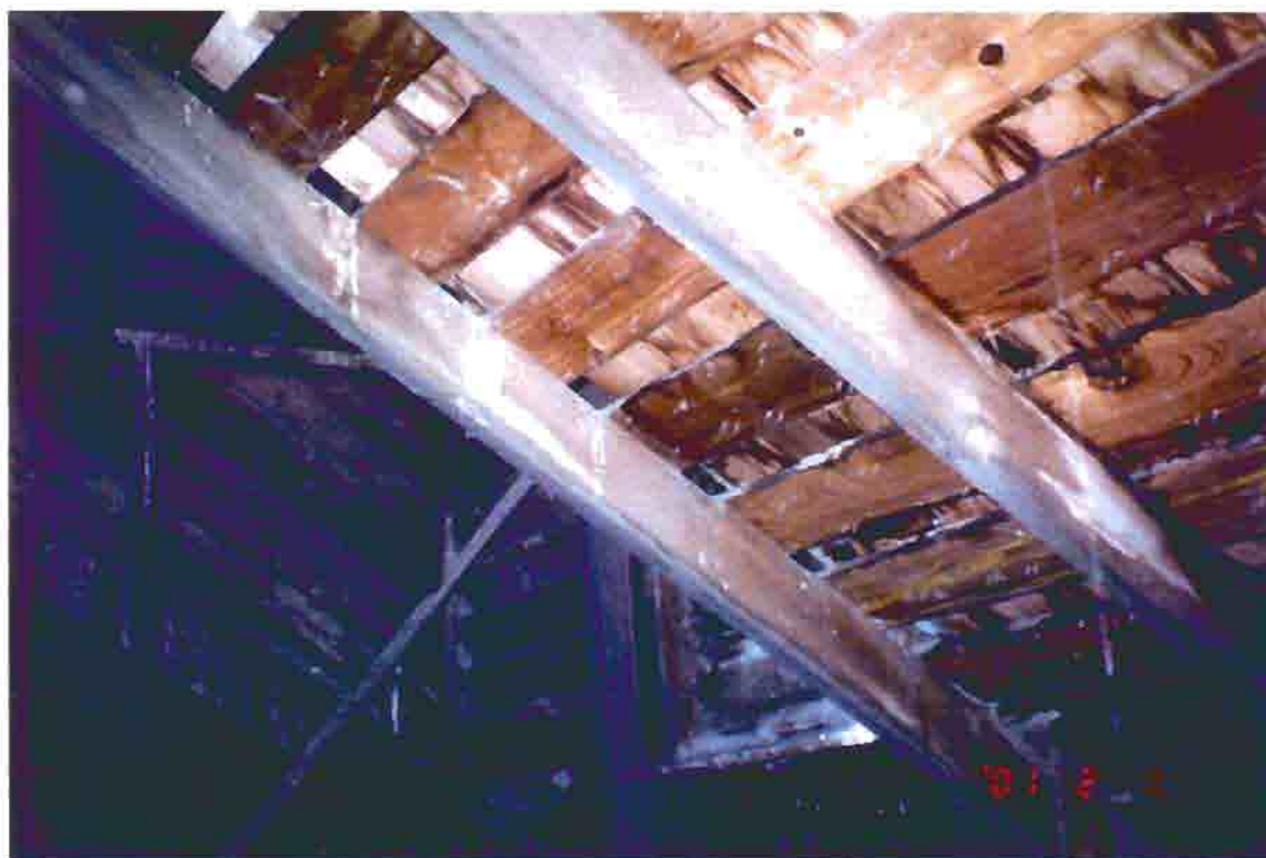
Photo S-28. The District No. 1 School, attic framing near the dormer, February 2001. Photo by Bahr Vermeer Haecker Architects, Lincoln, Nebraska.
