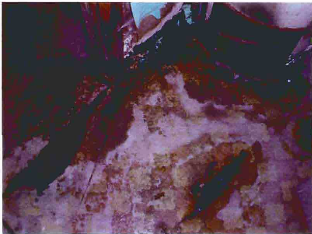
Photo F-24. The Fletcher-Switzer House, water damage in bathroom, February 2001. Photo by Wiss, Janney, Elstner Associates, Northbrook, Illinois.
