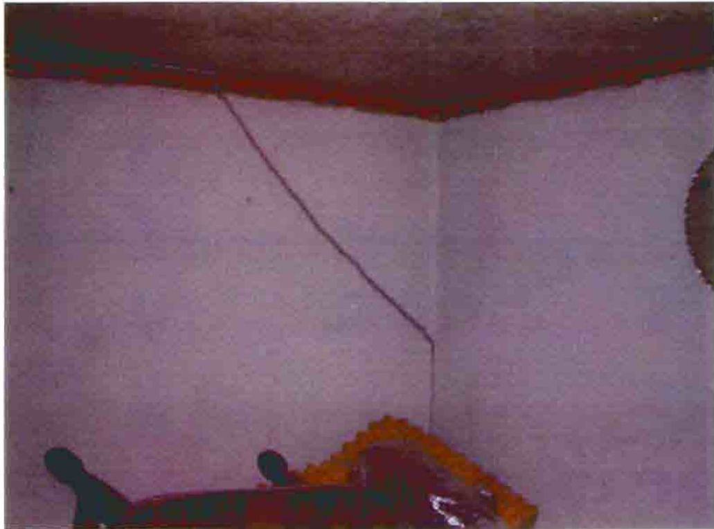
Photo F-27. The Fletcher-Switzer House, crack in interior wall, February 2001. Photo by Wiss, Janney, Elstner Associates, Northbrook, Illinois.
