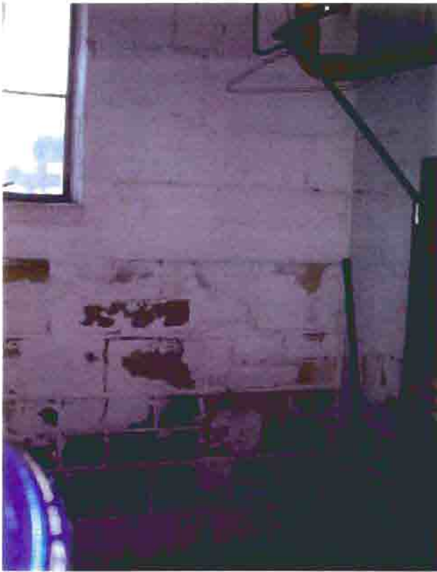
Photo T-21. The Township Hall, limestone foundation wall in basement, February 2001. Photo by Wiss, Janney, Elstner Associates, Northbrook, Illinois.
