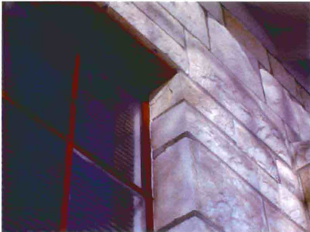
Photo T-20. The Township Hall, spalls in limestone at upper window jamb, February 2001. Photo by Wiss, Janney, Elstner Associates, Northbrook, Illinois.
