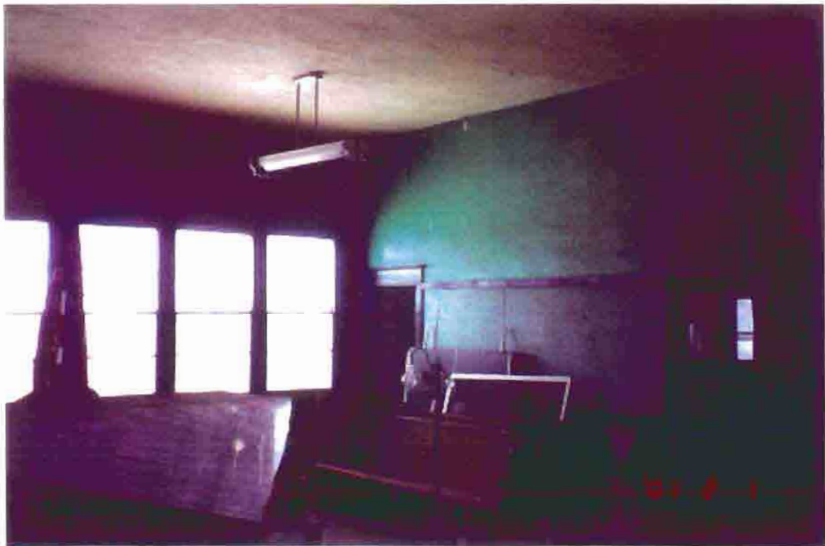
Photo S-22. The District No. 1 School, classroom interior, view to northeast, February 2001. Photo by Bahr Vermeer Haecker Architects, Lincoln, Nebraska.
