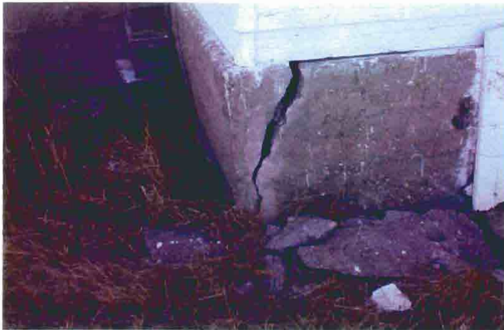
Photo S-19. The District No. 1 School, crack in foundation wall at northeast corner, February 2001. Photo by Wiss, Janney, Elstner Associates, Northbrook, Illinois.
