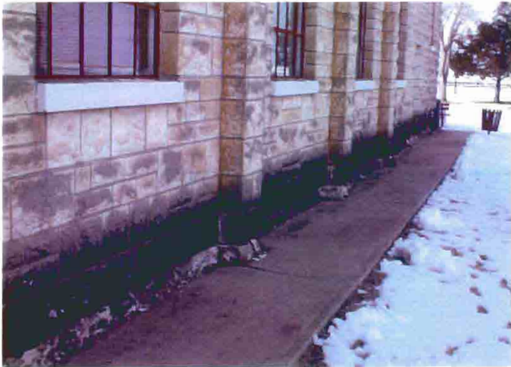
Photo T-15. The Township Hall, staining along the base of the limestone walls, February 2001. Photo by Wiss, Janney, Elstner Associates, Northbrook, Illinois.
