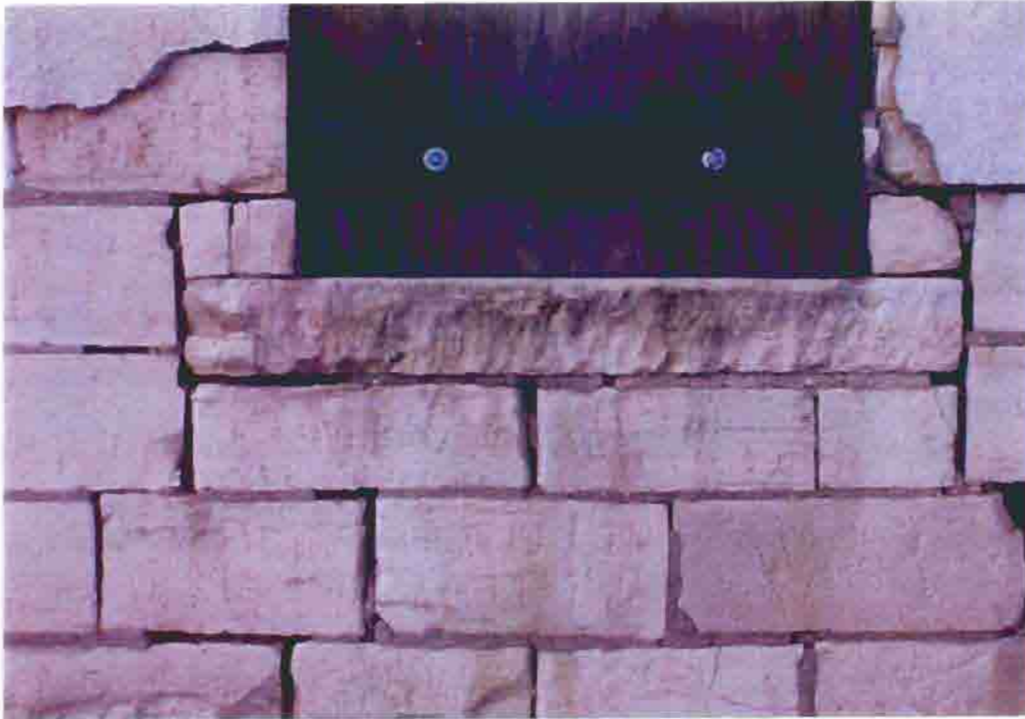
Photo A-21. The A.M.E. Church, limestone window sill, February 2001. Photo by Wiss, Janney, Elstner Associates, Northbrook, Illinois.
