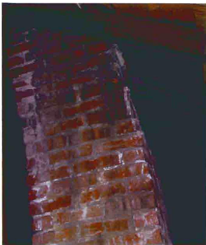
Photo S-27. The District No. 1 School, oblique brick chimney, February 2001. Photo by Wiss, Janney, Elstner Associates, Northbrook, Illinois.
