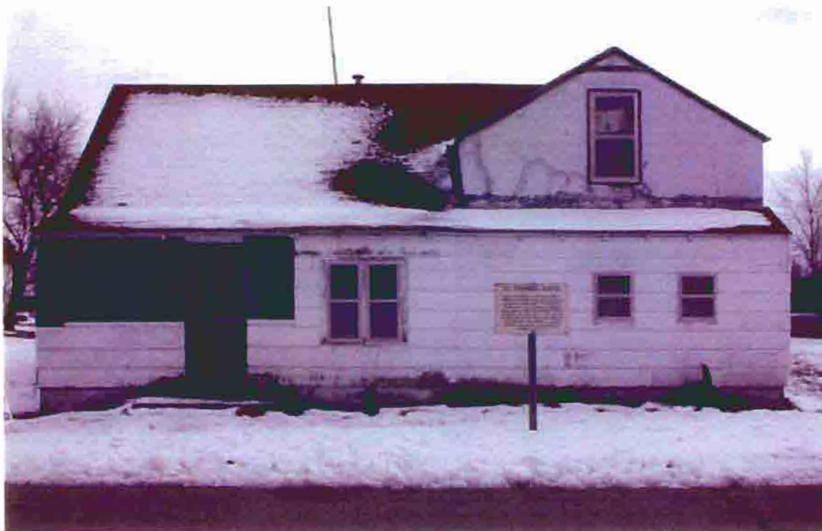
Photo F-11. The Fletcher-Switzer House, north elevation, February 2001. Photo by Wiss, Janney, Elstner Associates, Northbrook, Illinois.
