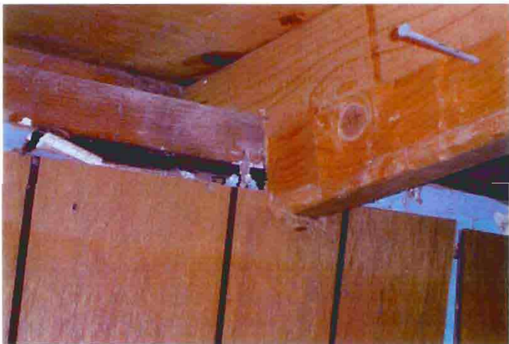
Photo F-28. The Fletcher-Switzer House, new rafters of porch roof, February 2001. Photo by Wiss, Janney, Elstner Associates, Northbrook, Illinois.
