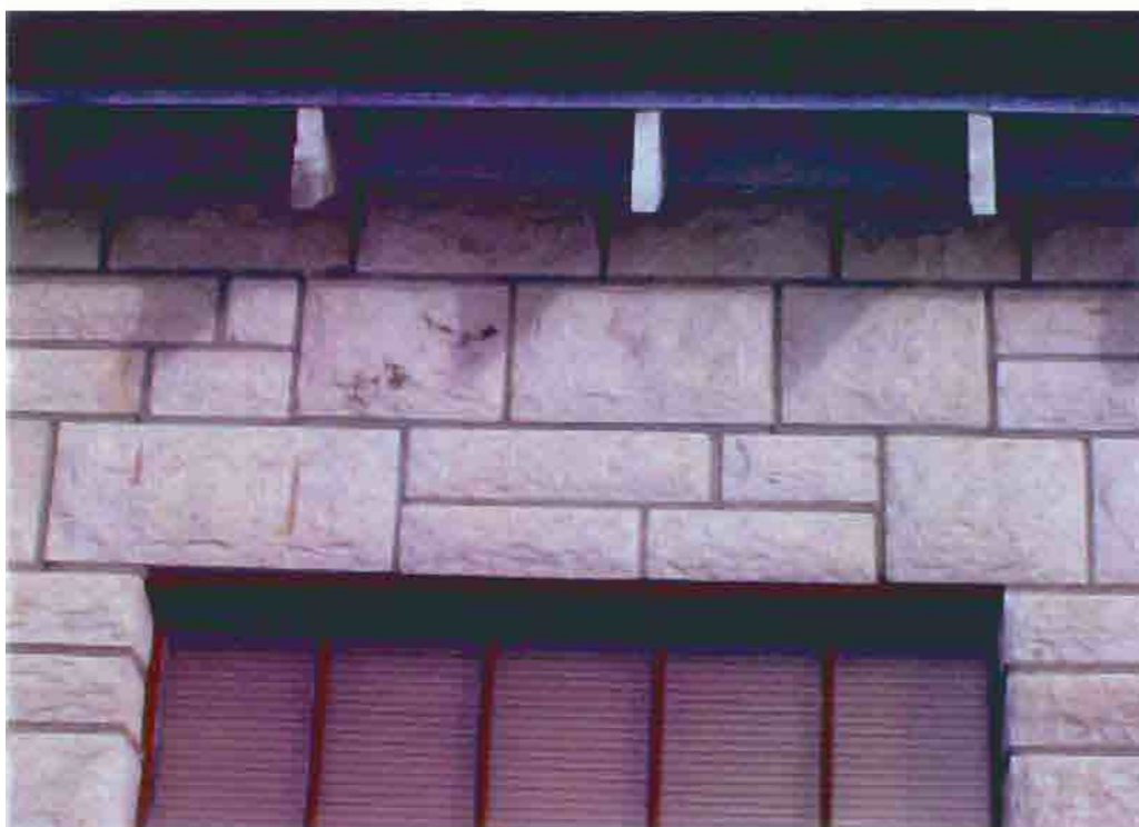
Photo T-17. The Township Hall, cracks above the window head, February 2001. Photo by Wiss, Janney, Elstner Associates, Northbrook, Illinois.
