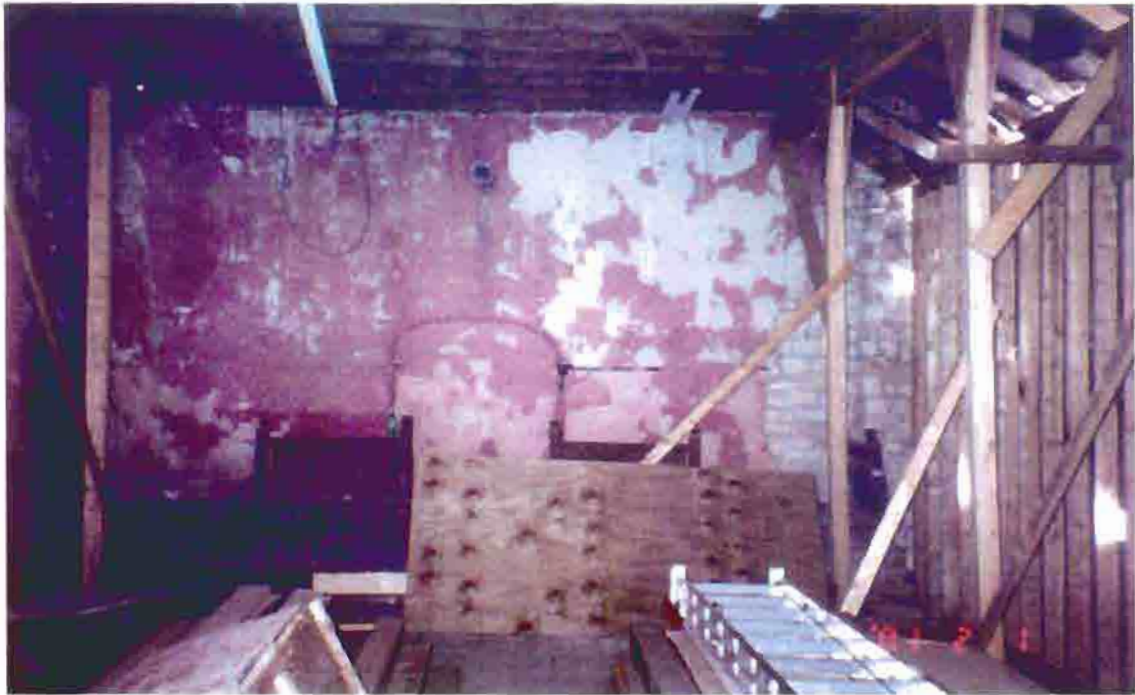
Photo A-23. Interior view of the sanctuary of the A.M.E. church, facing west, February 2001. The posts and beams that were installed to support the roof load are visible at right; beyond is the wood stud wall that replaced the north stone masonry wall. Above the niche in the west wall is a round pipe, where a heating stove was connected to the brick chimney. Photo by Bahr Vermeer Haecker Architects, Lincoln, Nebraska.
