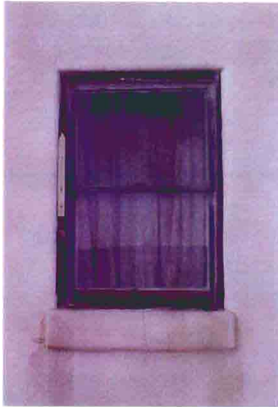
Photo B-17. The Old First Baptist Church, typical window, February 2001. Photo by Wiss, Janney, Elstner Associates, Northbrook, Illinois.
