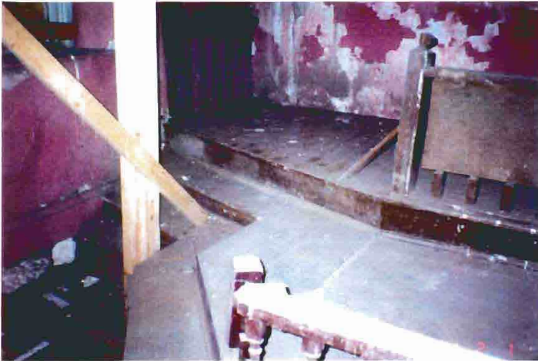
Photo A-25. The altar rail and platform at the west end of the A.M.E. church, February 2001. Photo by Bahr Vermeer Haecker Architects, Lincoln, Nebraska.
