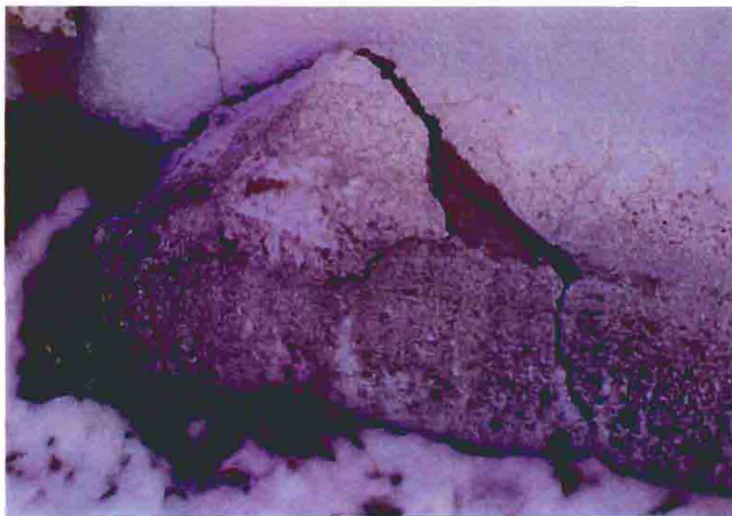
Photo F-20. The Fletcher-Switzer House, failing stucco at the foundation, February 2001. Photo by Wiss, Janney, Elstner Associates, Northbrook, Illinois.
