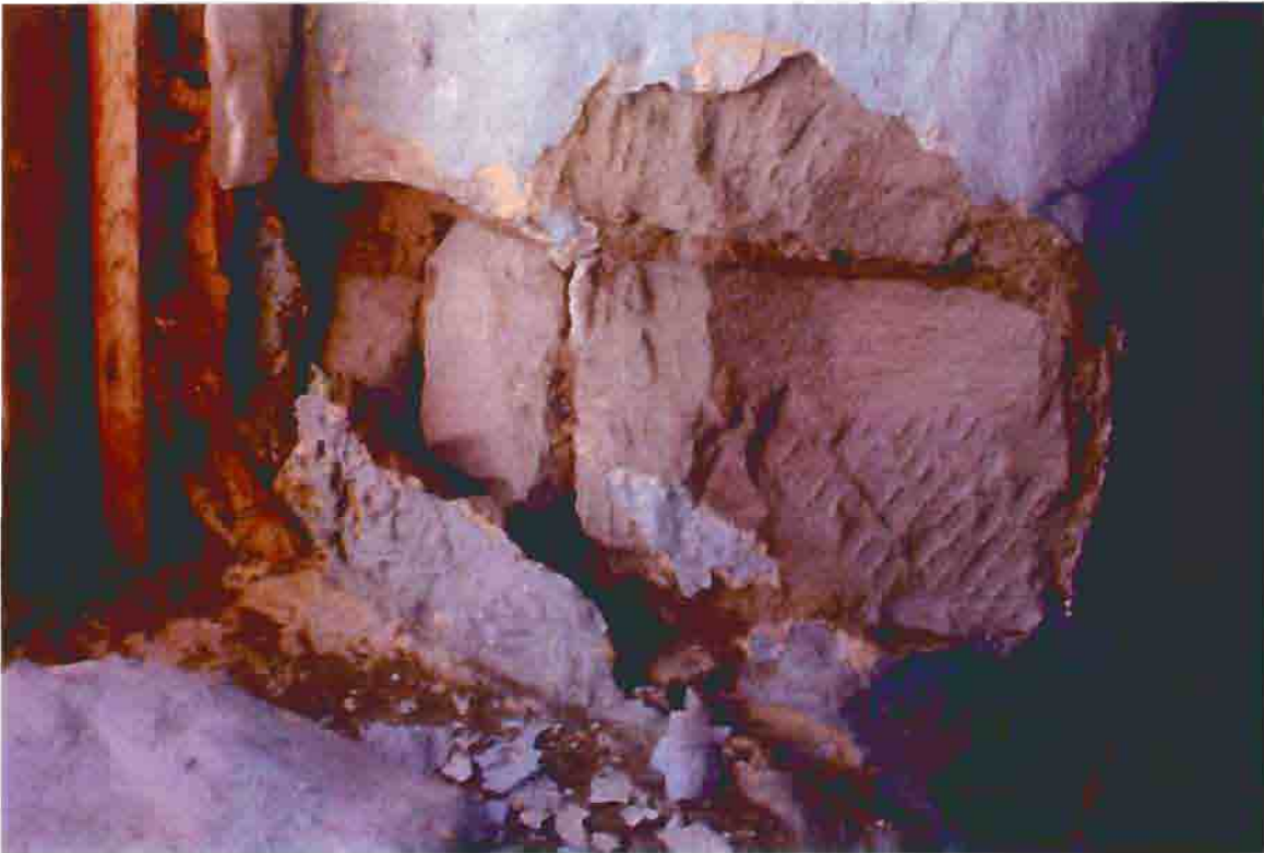
Photo F-30. The Fletcher-Switzer House, failed plaster at upstairs South Bedroom window jamb, February 2001. Photo by Wiss, Janney, Elstner Associates, Northbrook, Illinois.
