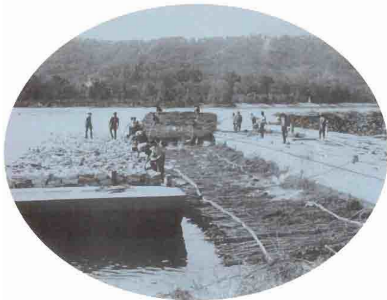
FIGURE 9. Wing-dam construction. Photo by Henry P. Bass, St. Paul District, Corps of Engineers.
