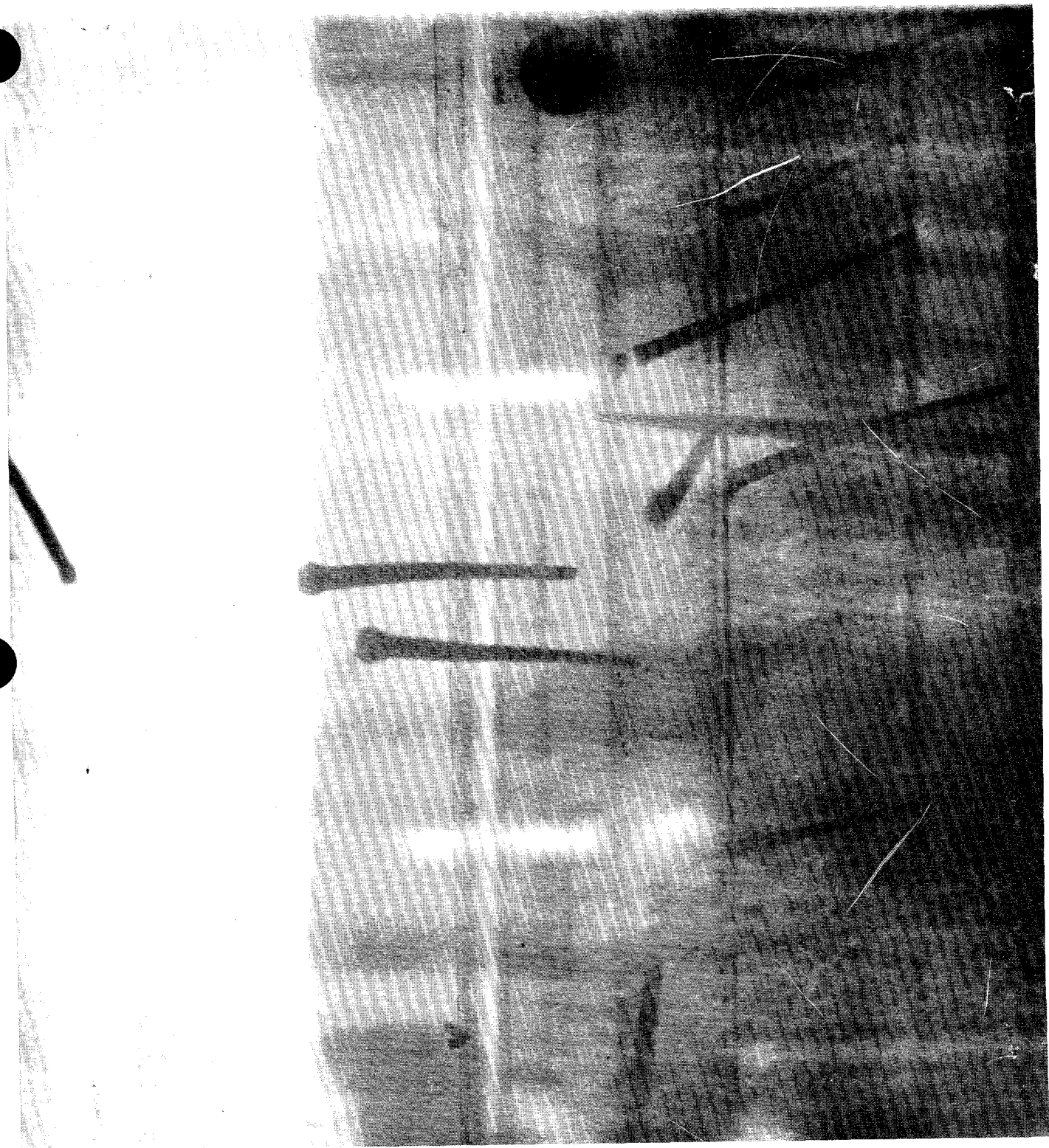
MAVA 01 X001 Room 105, south wall, east jamb of door 130, looking south 36" above the floor.
