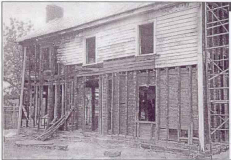
The WPTC photographs #9 & #31 above show the porch from the west (before removal, top) and the north elevation after removing the porch (bottom).
