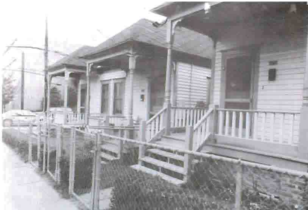
Fig. 35. Existing condition of double shotguns at intersection of Boulevard and Auburn Avenue, 1995.
