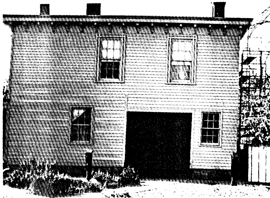
Photo showing back side (east) with primer and one top coat of paint applied.
