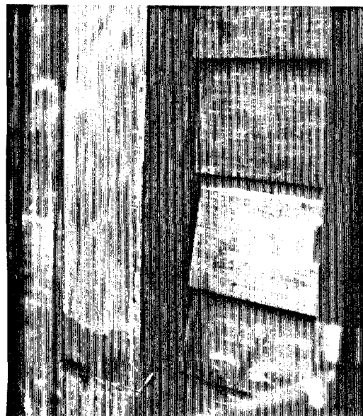
Photo showing large space in between board siding and trim at corner, front (west). Arrow showing this.
