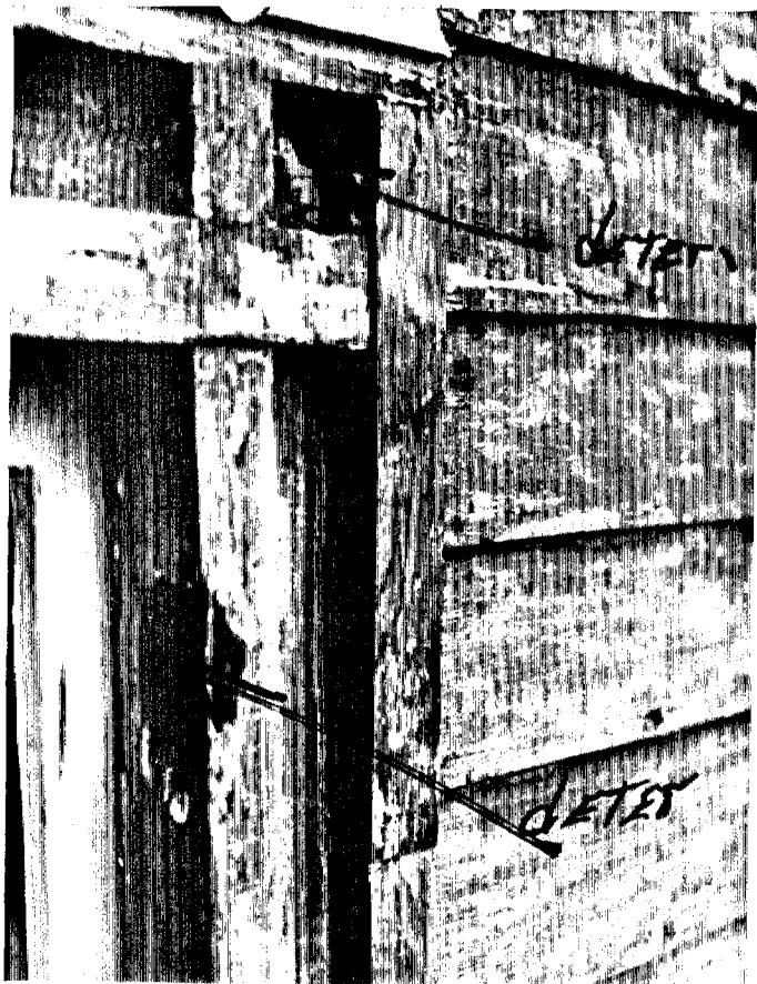
Photo showing deterioration in trim and siding. Arrow showing this.
