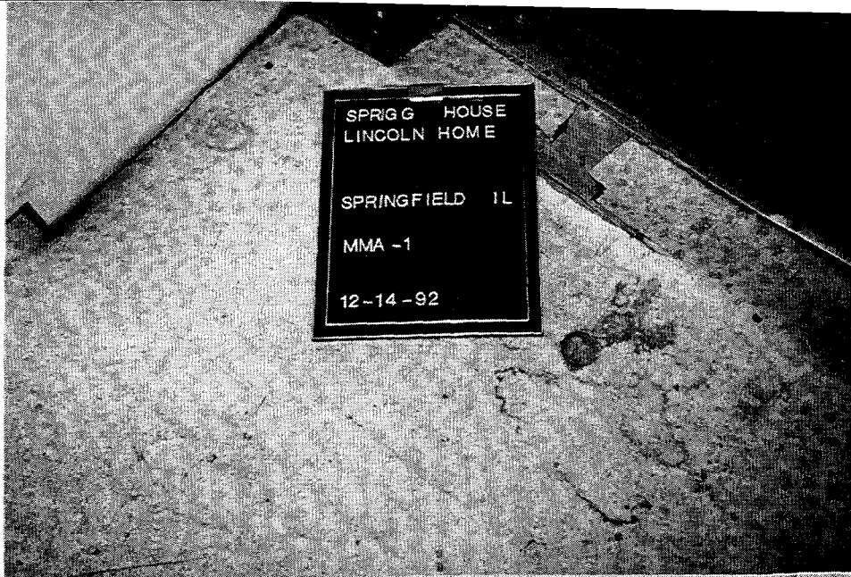
Photo MMA-1 Mastic Under Sheet Flooring Room 208
