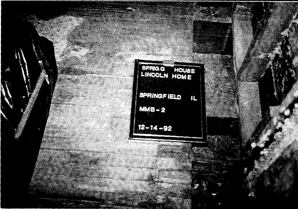
Photo MMB-2 Felt Paper Under Wood Floor Room 208
