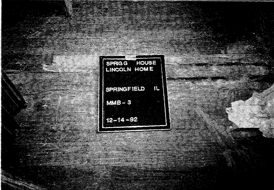
Photo MMB-3 Felt Paper Under Wood Floor Room 202
