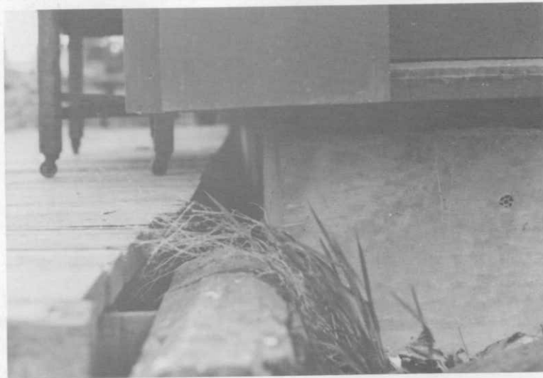
Photograph 22. 1981. Southwest corner. Building offset from foundation.
