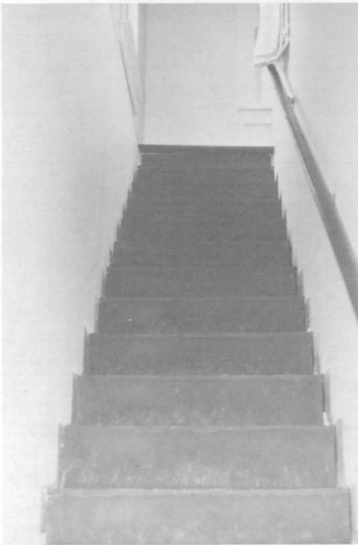
Photograph 22. North stairs. Remove and relocate.
