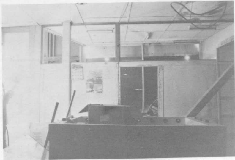
Photograph 26. 1978. As found conditions.
