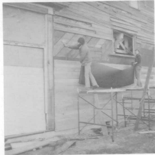
Photograph 21. April 1980. Note typical 1 x 12 diagonal sheathing with horizontal boards at historic window location.
