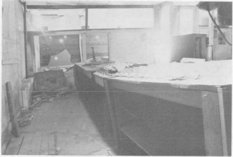
Photograph 29. 1978. As found conditions.
