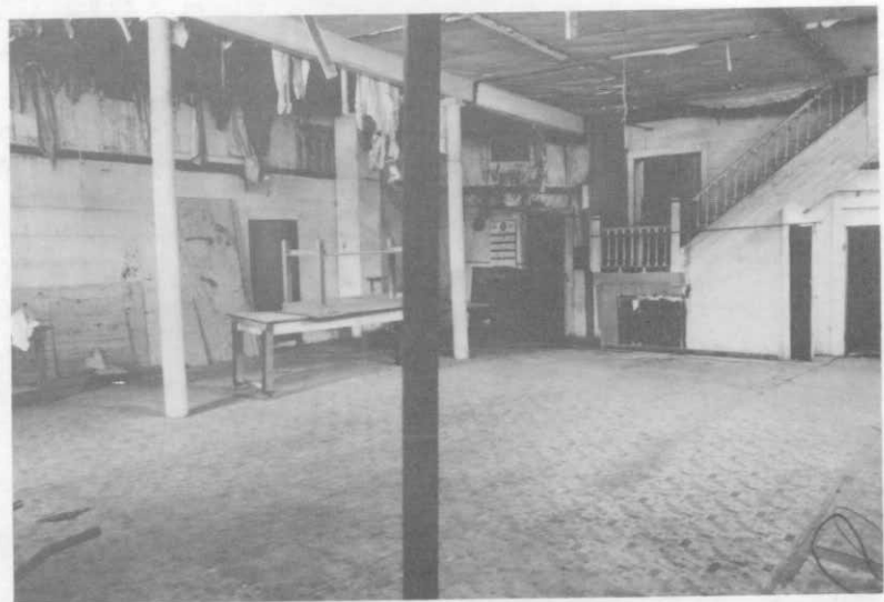
Photograph 39. 1978. After debris removal.
