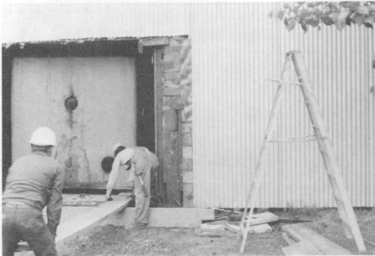
Photograph 27. South elevation during removal of bakery oven. Note haphazard construction of wall sheathing.
