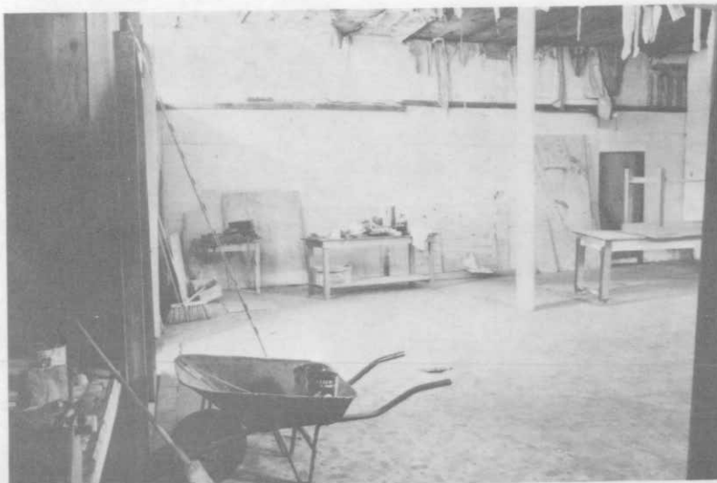
Photograph 40. 1978. After debris removal.
