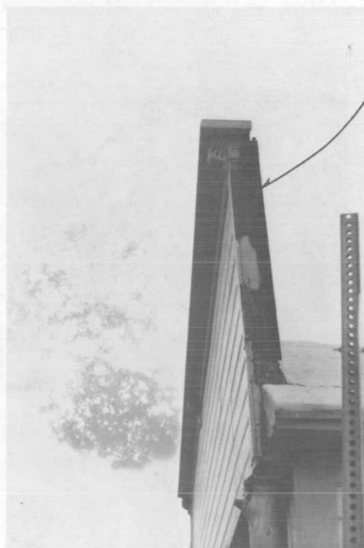
Photograph 24. False front detail.
