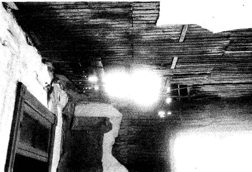
40. Ceiling at southeast corner of room 105, Unger House. February 1984. NPS photograph.
