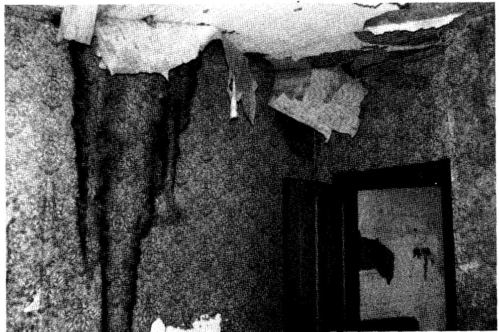
34. Water stain on east wall of room 101, Unger House. Early 1980s, NPS photograph.
