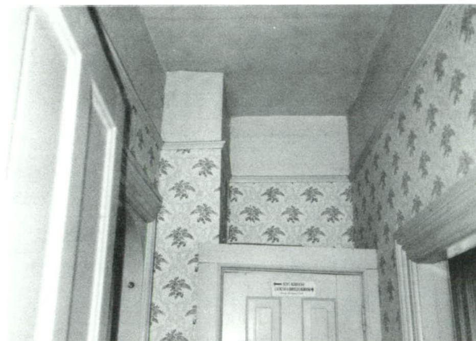
SP-12, Wall displacement, room 209.
