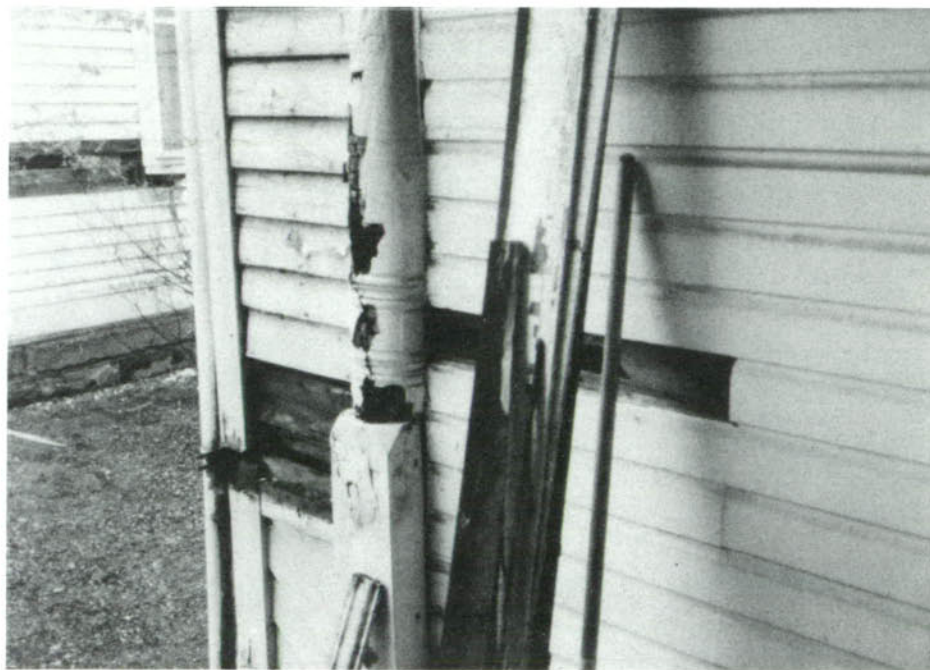
SP-8, Wall deterioration adjacent to the porch.
