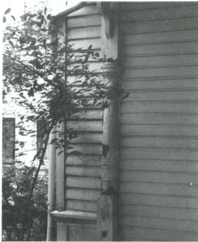
CP-35, Roof and flashing problems have caused severe deterioration at the exterior of the parlor stair and west porch. Engaged porch column, siding, trim are rotted. Porch rail is missing entirely.
