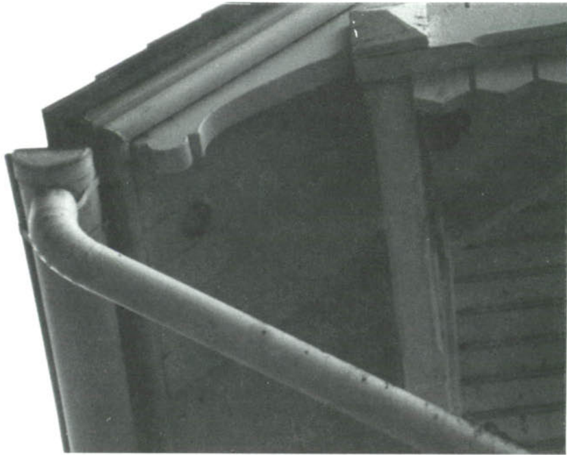
CP-15, Eave detail at the downspout. The hole through the roof sheathing at the right is from the original downspout. Half-round gutter at the left has replaced the original trough gutter system. Pigeons on the bracket soil the building with waste.
