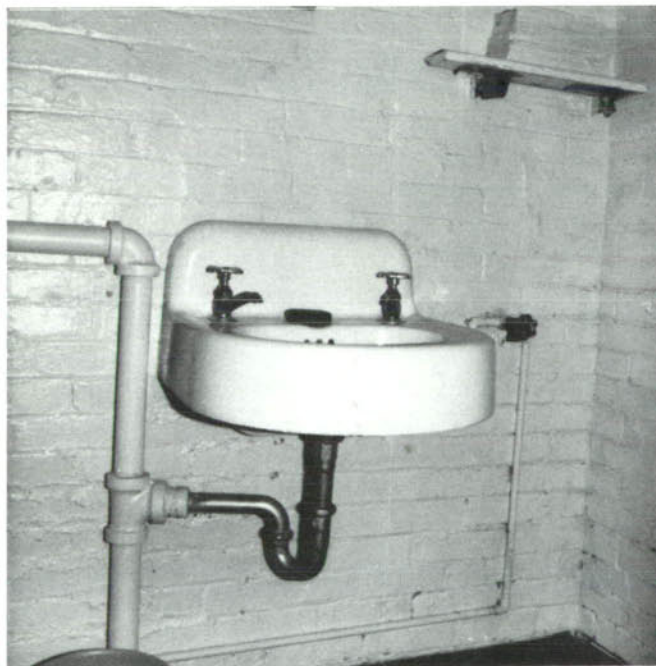
CP-58, Rest room itself is minimally accessible. The installation of grab bars will be required at the toilet.
