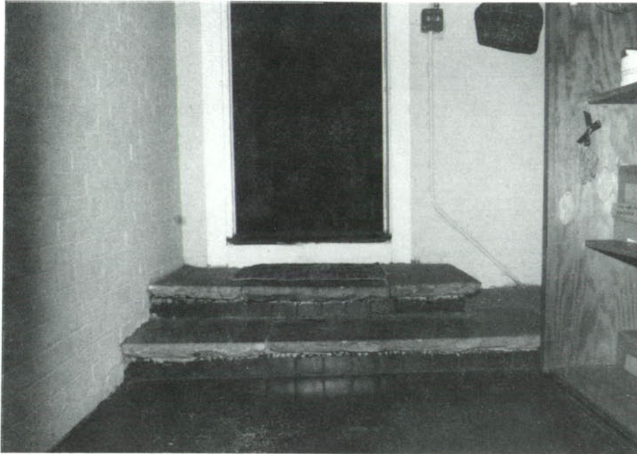
CP-59, A three-riser stair from the gift shop to the first-floor of the house is a barrier for wheelchair bound visitors.
