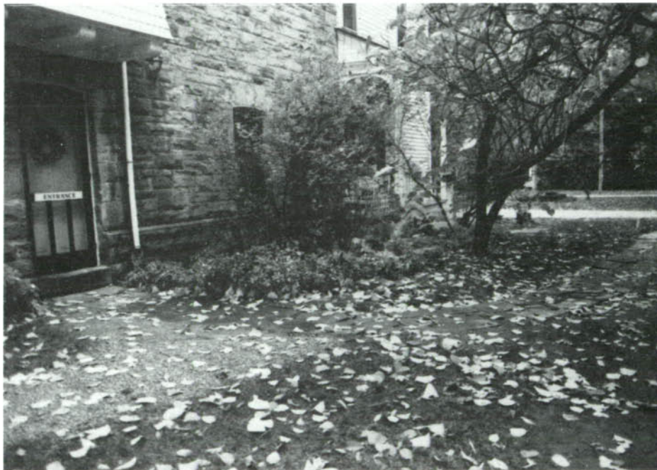
CP-56, Use of flagstone walks have historic precedent, but uneven and irregular open joints are an impediment to wheelchairs.
