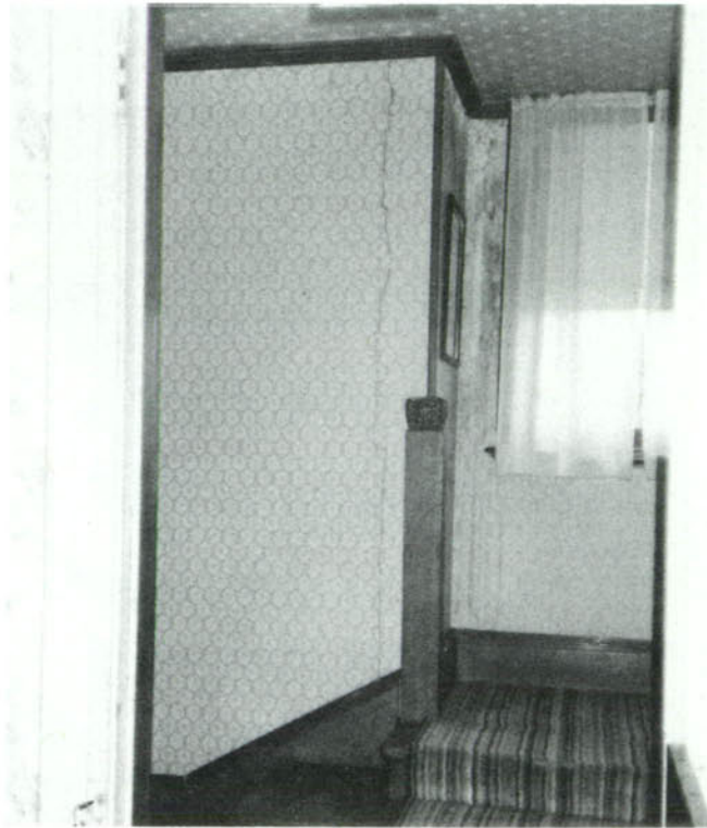
SP-28, Second-floor wall crack at the main stair.
