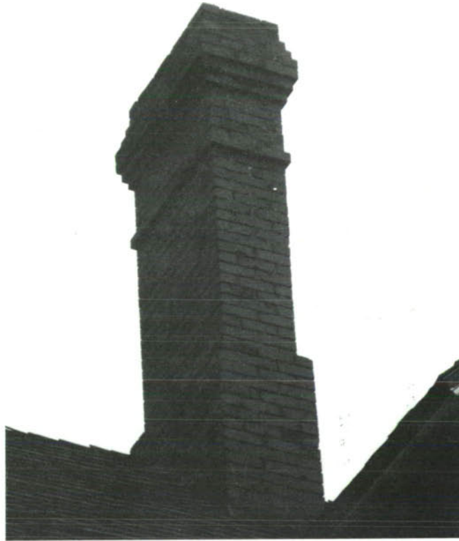
CP-9, Typical tall chimney unsupported above the roof. All chimneys need repainting.
