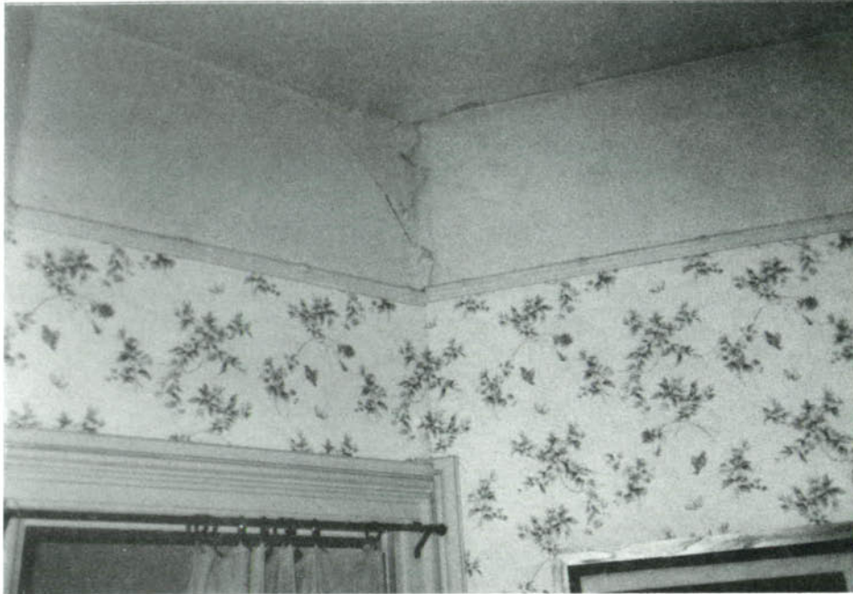
SP-15, Wall displacement, rooms 201-202.
