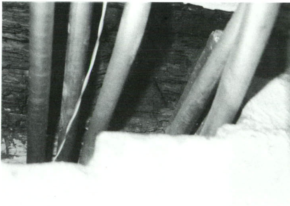
SP-24, Sill plate rot.
