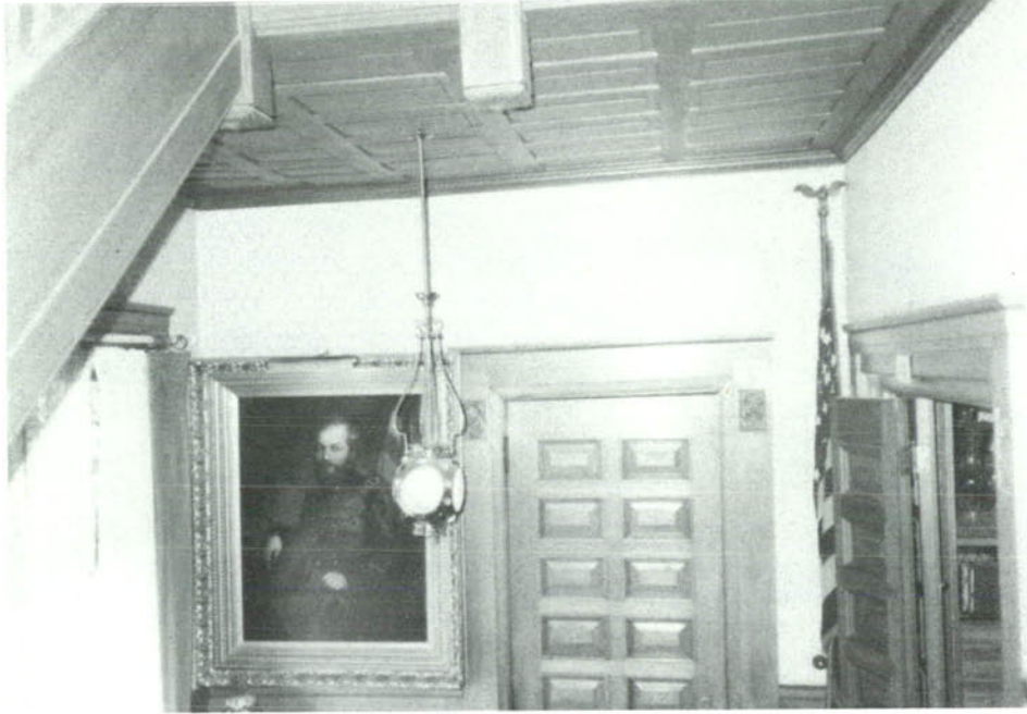
SP-25, Exterior wall displacement outside the library.
