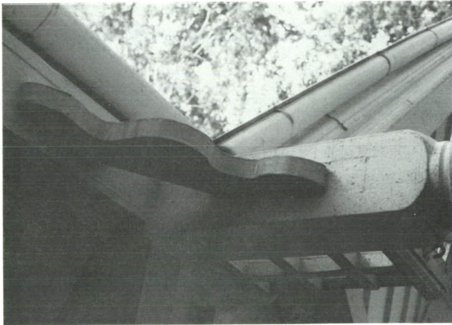
CP-34, West porch, shadow of original porch brackets is visible below the replacement.
