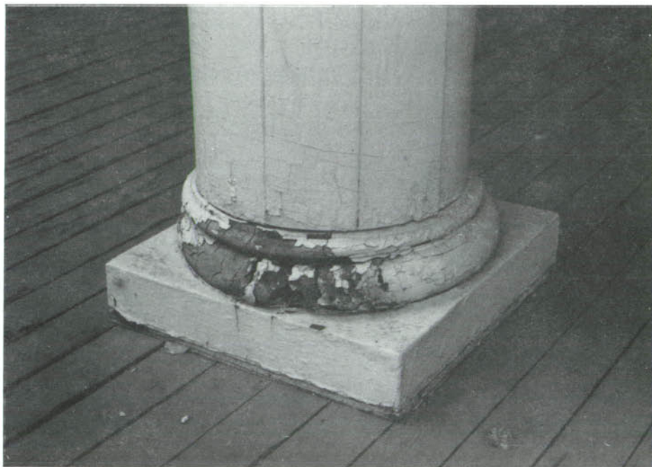
CP-20, Several of the column bases exhibit rot at the bases.
