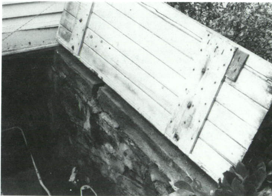
CP-48, Wood doors and stone walls of the cellar entrance are in poor condition, allowing moisture to enter and providing little security.
