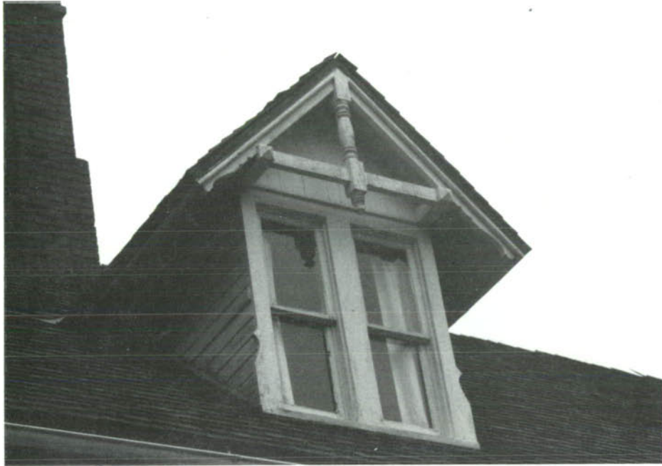
CP-13, Typical dormer on the 1880 portion of the house. Finial above the roof is missing.
