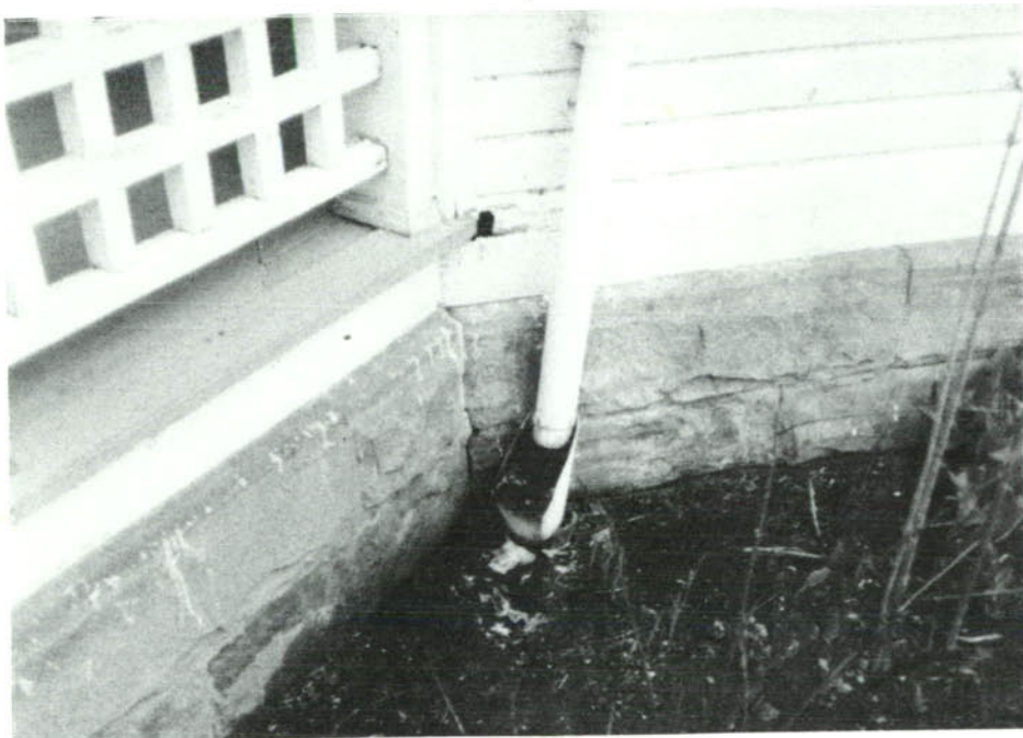
SP-42, Downspout drain overflowing.
