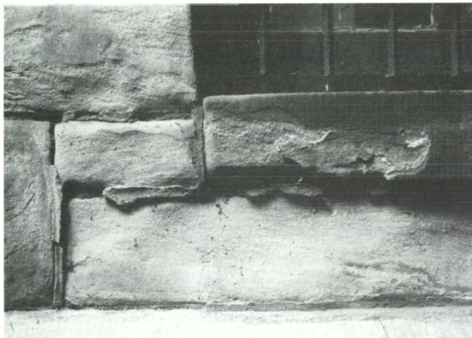
CP-38, All ground level memorial library stone window openings have stone problems, although not as severe as the above window.
