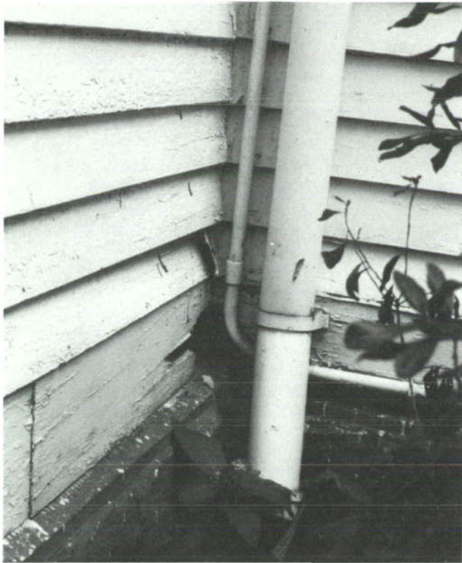
CP-41, Inside corner at 1885 kitchen. Water intrusion in the wall from the gutter above has caused severe deterioration from roof to foundation.
