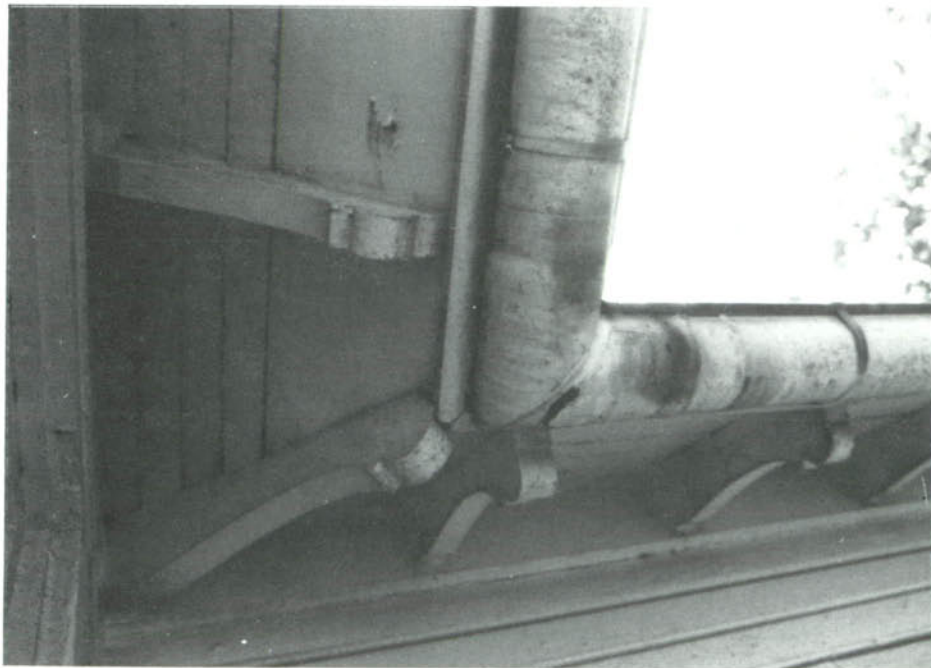
CP-16, Original narrow exposed eave sheathing boards replaced with wide board, probably at the time of gutter replacement. Note the rafter tip splice repairs.
