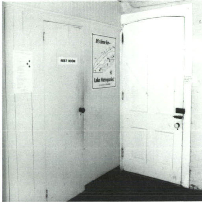
CP-57, Entrance to the rest room is too narrow for handicapped accessibility.
