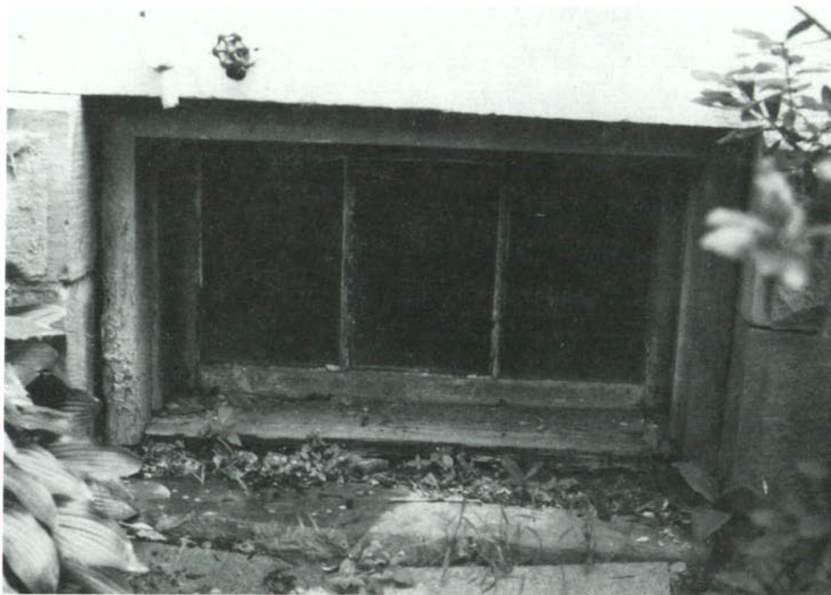
CP-47, Typical deteriorated basement window. The grade is too high and the foliage is too close to the wood frames, keeping them continuously damp.
