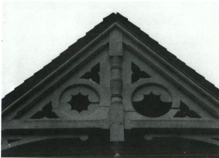
CP-12, Fret detailing of the large gable on the south side. Finial above the roof is missing as well as the lower half of the right hand circle.
