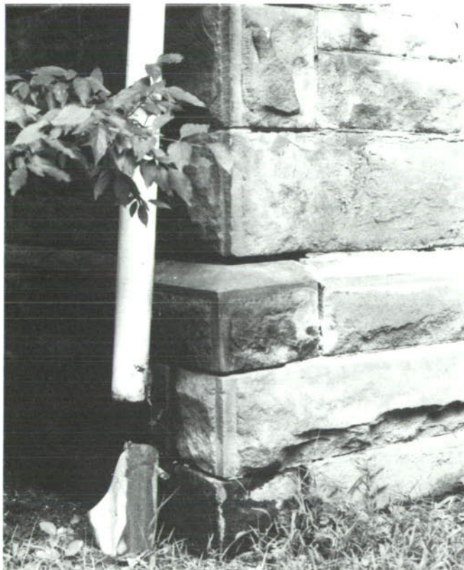
CP-42, Downspout is not connected to the drain and the back side seam is open allowing water to wash over the stone, leaching mortar from the joints.
