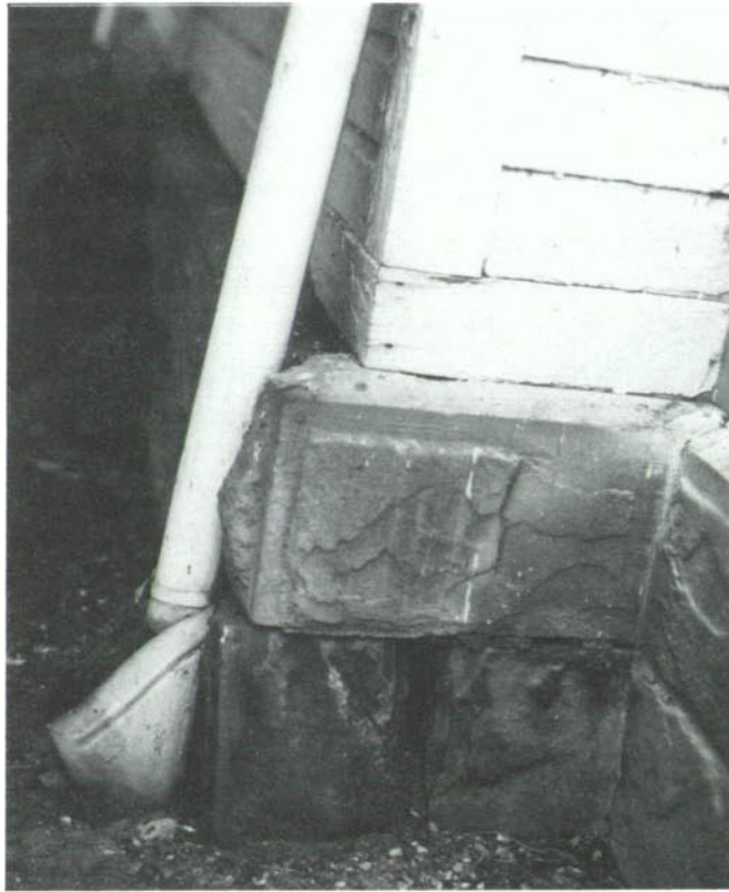
CP-39, An often blocked drain and separated stone veneer channeling into the foundation wall have caused deterioration of the brick masonry.
