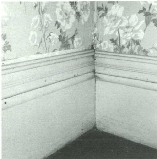
SP-18, Floor trim displacement, northeast corner, room 216.
