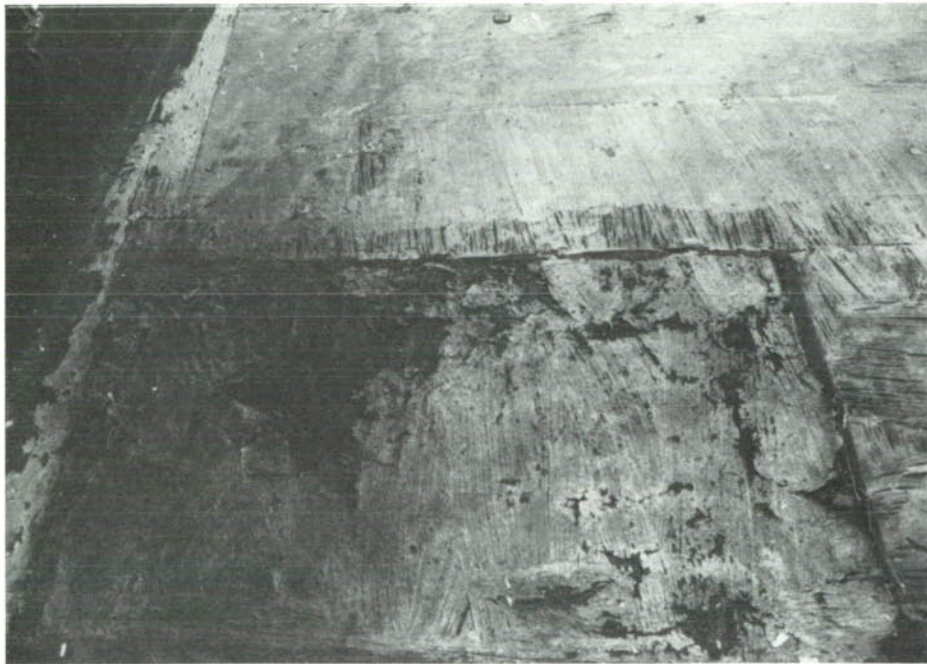
CP-18, Deteriorated roofing of the east porch.
