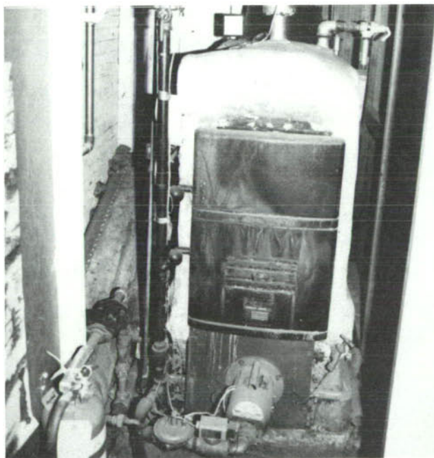
CP-62, Steam boiler has friable asbestos insulation which needs to be removed.
