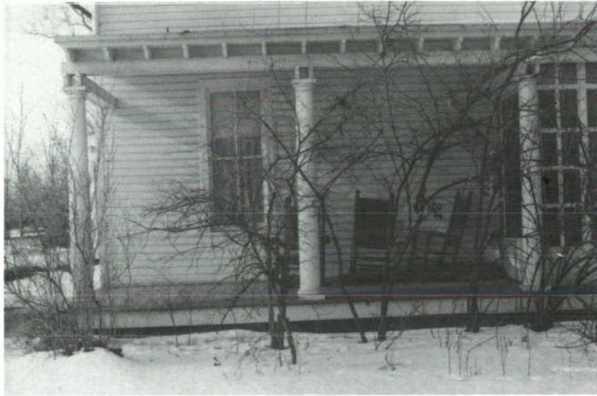
CP-25, East porch exhibits the same problems as the south porch.
