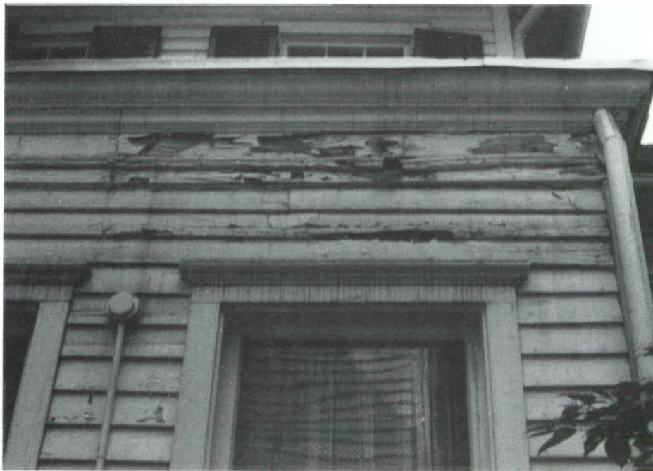
CP-36, Another view of the rotted siding at the parlor stair. There is most likely structural damage within the wall as well.
