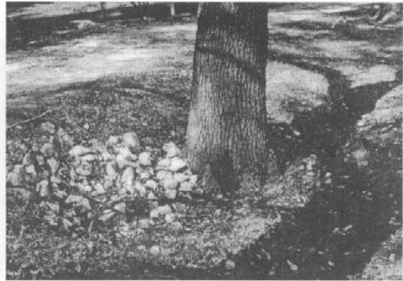
Figure III-35: Erosion and culvert at #48, north side of road, 8/11/98.
