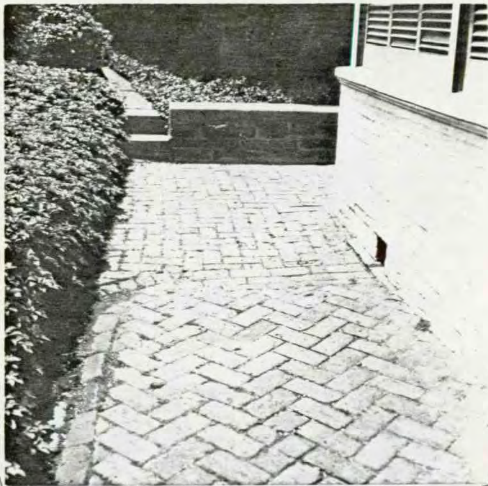
ILLUSTRATION 63 1880 Section Brick paving outside Room 115, looking west. Note opening through wall for hydrant.
