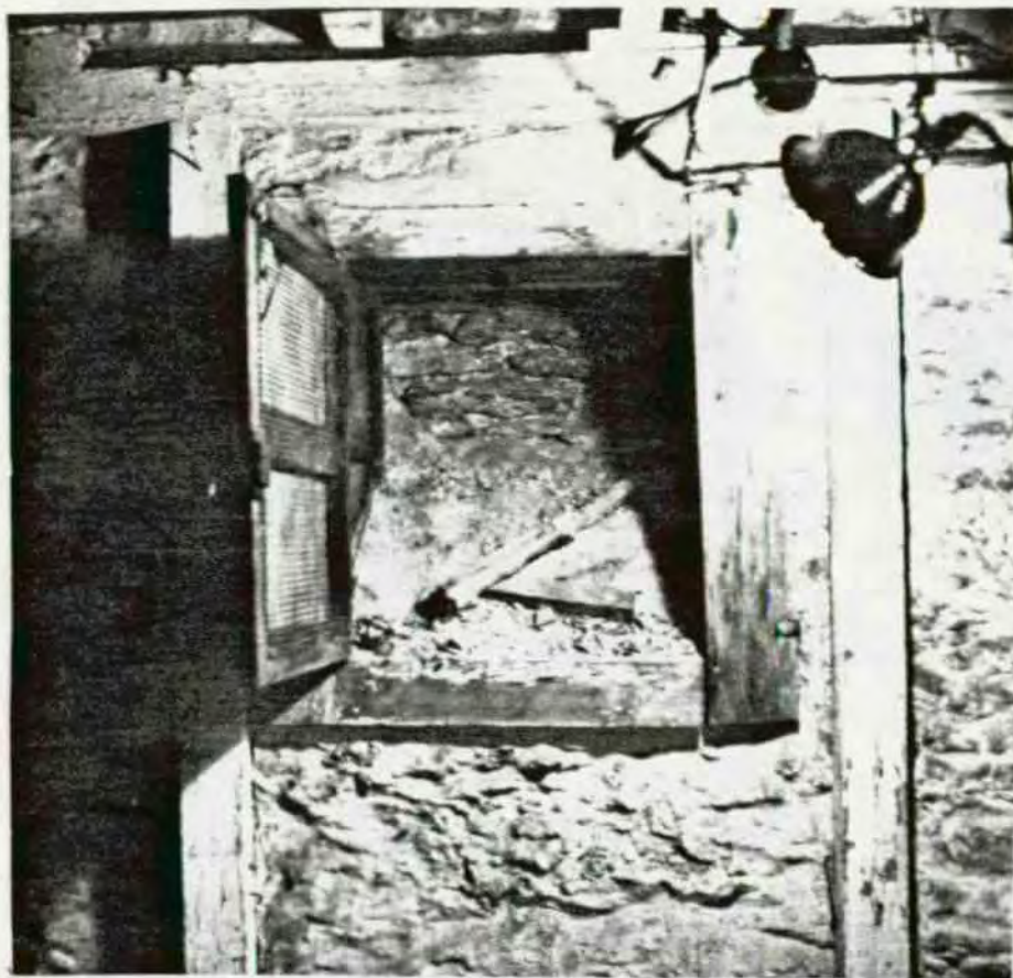
ILLUSTRATION 18 - PHOTOGRAPHED BY NPS. 1750 Section Cellar - south wall, looking south. Opening under porch utilized for dumping materials into cellar before 1772.
