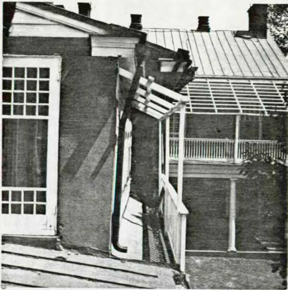
ILLUSTRATION 15 - PHOTOGRAPHED BY NPS. 1850s Section Original roof cornice - imitation of 1750s roof cornice in background. Note clapboards above the second floor on the west elevation, looking east.
