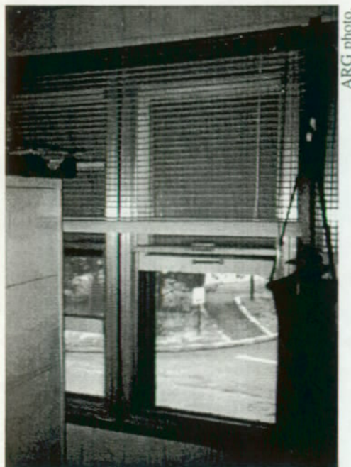
Figure 27: Double-hung wood sash window at Room 201. Note underside of awning outside window.
