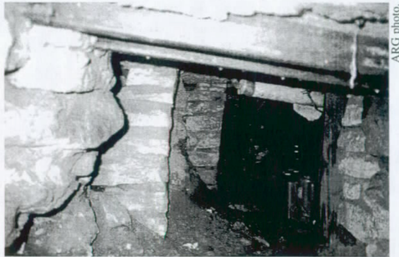
Figure 29: Utility tunnel. Standing ground water was measured to a depth of 24" in May, 2000.
