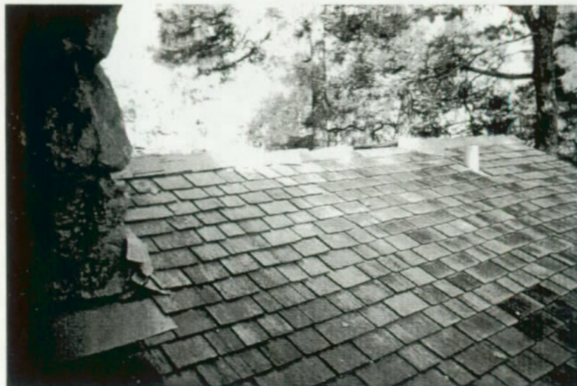
Figure 28: Roofing over toilet room addition. Some wood shingles are slipping at ridge line.
