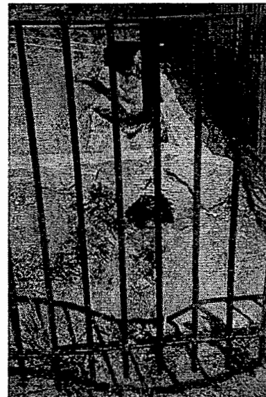
Photograph 127. Concrete-lined swale with decorative cut stone arch, viewed through iron fence at Depot. (JMA, 2001)
