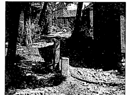
Exposed utility boxes
