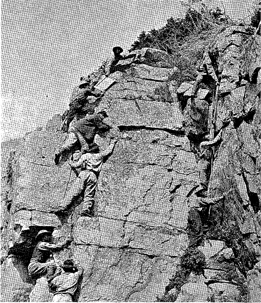
Mormon surveyors at work on the construction of the Union Pacific Railroad in the Wasatch Mountains. This photograph was taken by Charles R. Savage and is a gift of the Union Pacific Railroad Company.
