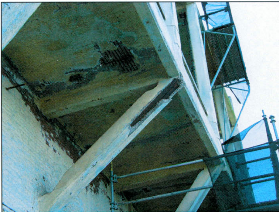
Top: View of underside of concrete balcony under repair, 2003. Photo Credit: John Martini.
