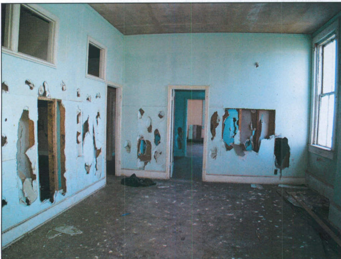
Above: Typical apartment interior with 1/4" gypsum board partition walls, 2003. Photo Credit: John Martini.
