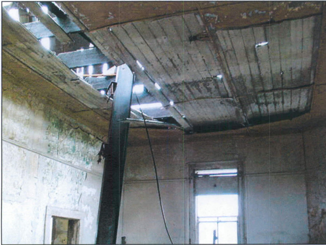
View of extensive ceiling damage at south end of third floor, 2003. Photo Credit: Jane Lehman.
