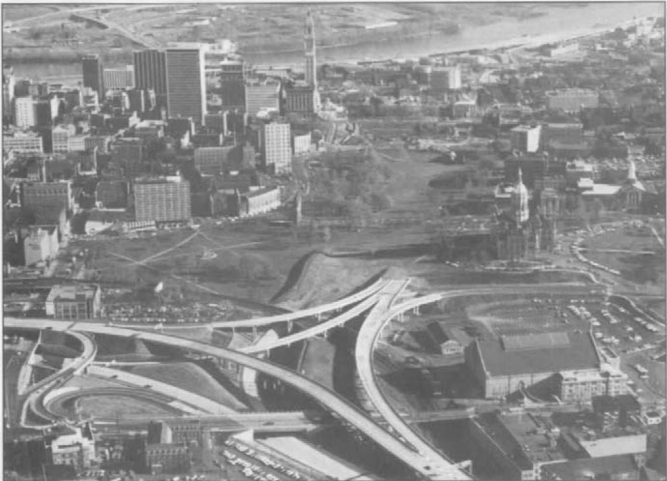
Construction of an interstate highway interchange in Hartford, Connecticut, circa late 1960s. Courtesy, National Register Branch, National Park Service Washington Office (WASO).
