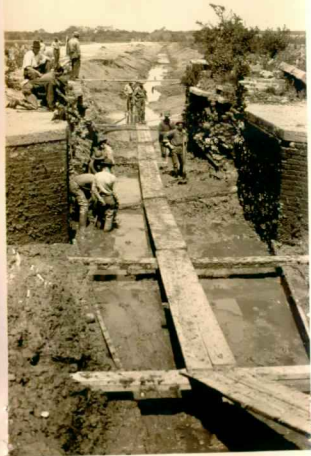
Beginning to lay wooden footing in main ditch, April 5, 1935. Much of the early work in the reclamation of Cockspar Island was done knee-deep to waist-deep in soft mud.
