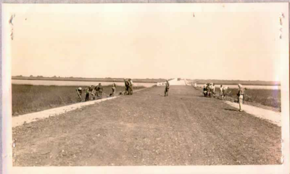
Much attention was given by CCC forces in 1938-40 to the final preparation of the causeways to receive surface treatment and serve as the entrance road and administration area road. Above, at work on south bridge approach, October, 1938, placing mud on slopes preparatory to laying riprap which is necessary to protect the fill from tidal action.
