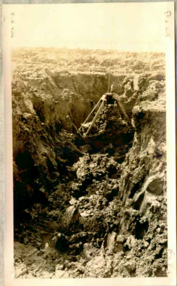
Cutting diversion ditch around tide gate, Ditch No. 5, showing type of soil when no water present. Much of the work of the enrollees was done in this type of soil during the first years.
