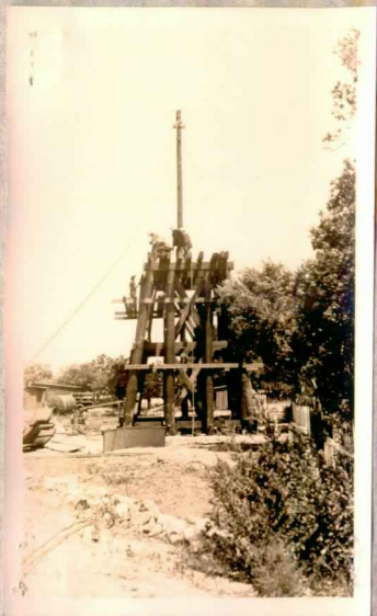
Among the numerous small jobs not listed in this summary is the erection of a temporary overhead water tank in the CCC shop yard. Enrollees are shown at work on this structure.
