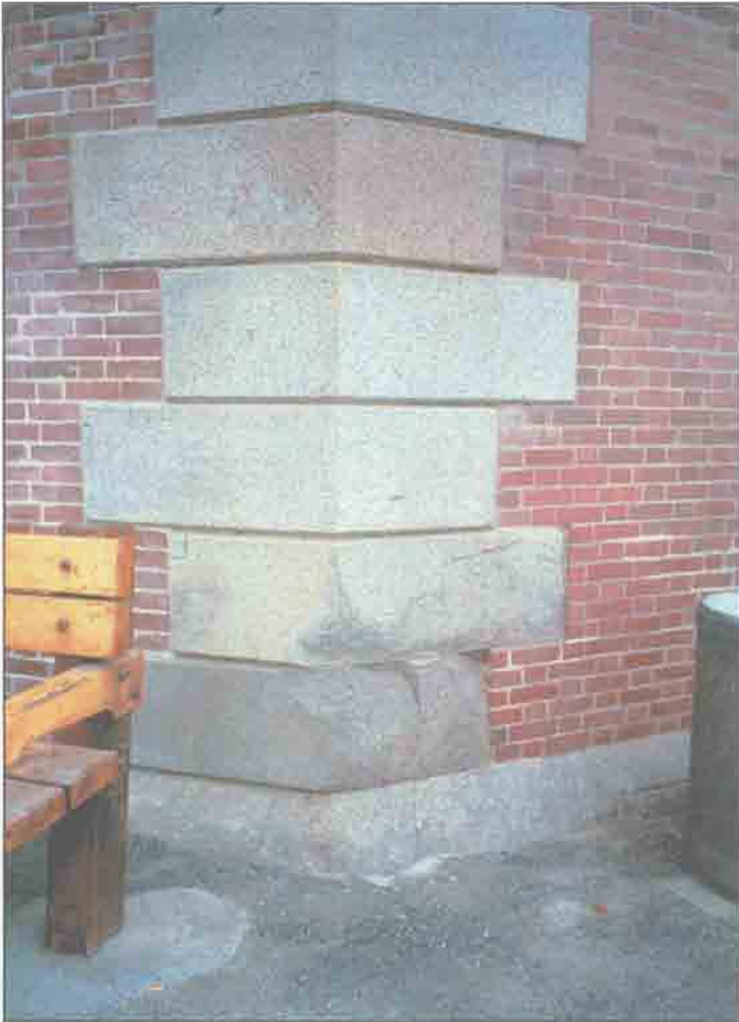
Condition Photo 2: East Bastion—East Flank, impact damage at granite quoins and base. (Courtesy of ARG, 2003)
