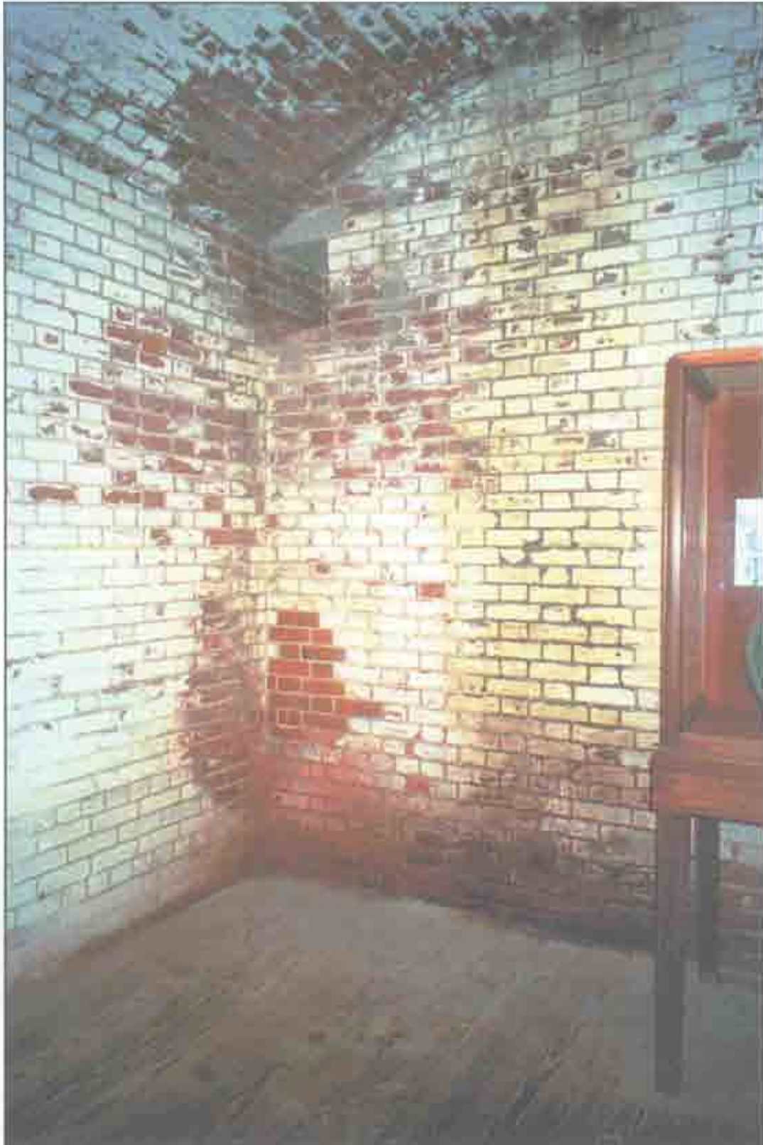
Condition Photo 16: Casemate 11; Open joints at the brick masonry and heavy water infiltration. Biological growth on the interior brick. (Courtesy of ARG, 2003).
