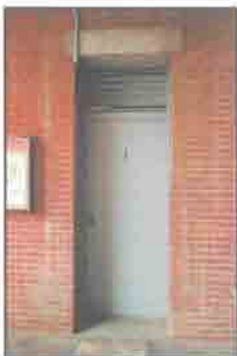
The transom windows above the 3rd tier gallery doors were replaced with wood louvers. These louvers need to be replaced because they are all installed backwards. (John Martini, 2005)
