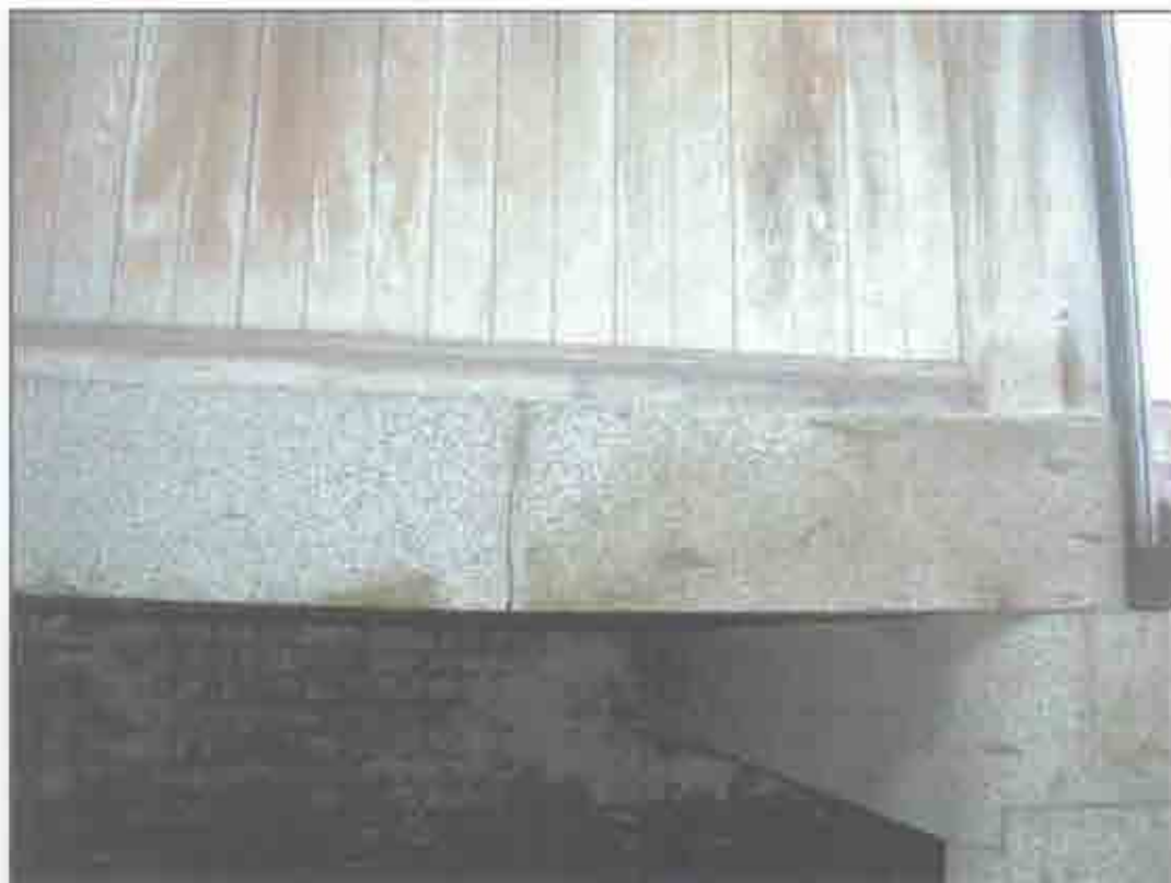
Condition Photo 6: Top Landing at Barbetta Tier; Crack in granite. (Courtesy of ARG, 2003)
