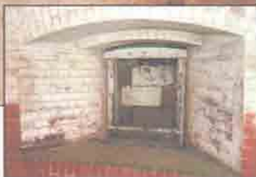
Most of the iron embrasures have deteriorated over the years and the openings have been infilled with brick and block for security purposes. (John Martini, 2005)
