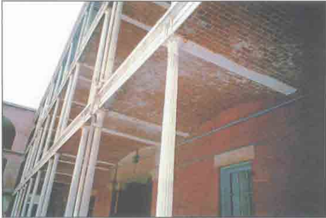
Condition Photo 10: Southeast Face Courtyard; Corroding metal columns and walkway supports. Missing metal railings in this photo have been reinstalled. (Courtesy of ARG, 2003)
