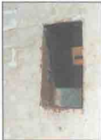
Seven original 6" x 12" rifle slit openings remain in the sallyport. (John Martini, 2005)
