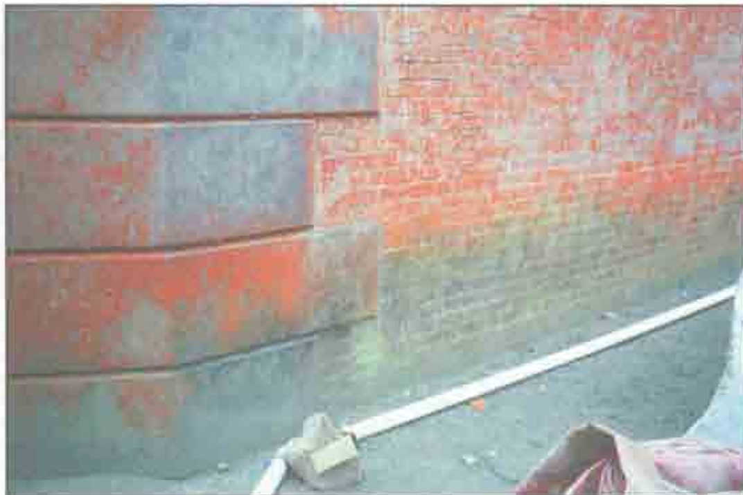
Condition Photo 1: Northwest Face Elevation; Biological growth located on brick wall and granite quoin surfaces. Exfoliation on granite quoin is due to the growth. (Courtesy of ARG, 2003)
