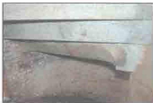
Stair #2 - Extra headroom was created between the 1st and 2nd tiers by carving into the granite tread. (John Martini, 2005)
