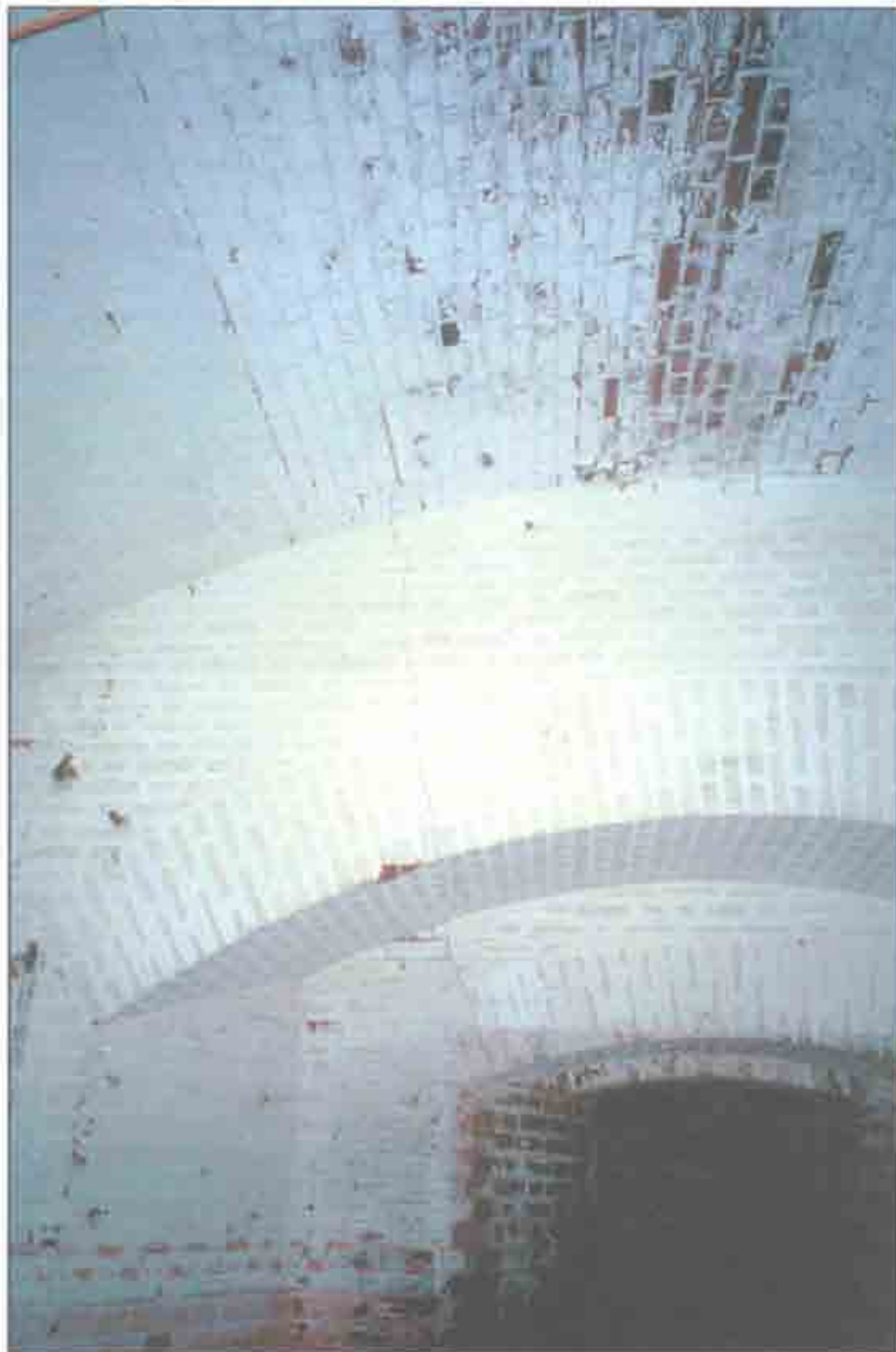
Condition Photo 15: Casemate 19; Cracks in brick masonry and joints have failed. The heavily flaking paint is typical in casemats. (Courtesy of ARG, 2003)
