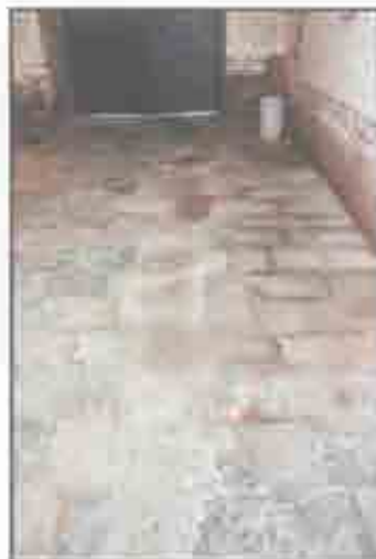
The original granite floors remain in good condition although a large concrete patch exists where a previous water line was installed. (John Martini, 2005)
