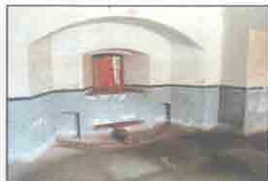
Typical cannon embrasure. This embrasure in casemate 2 still retains part of its original front pintle carriages. (John Martini, 2005)
