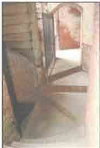
Each landing in the circular staircase is composed of slightly different shaped pieces of granite depending on the floor-to-floor heights. (John Martini, 2005)
