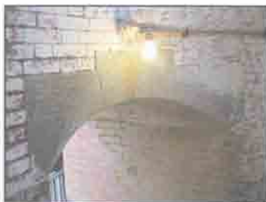
Stair #3 - The header over the openings on the 3rd tier consist of a 3-part segmental granite arch. (Jane Lehman, 2005)
