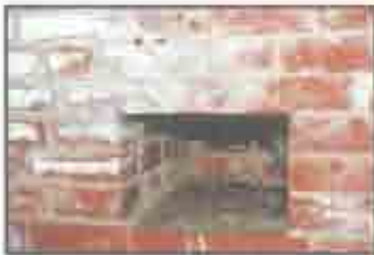
This small kitchen vent has a keystone brick on the top part of the opening. (John Martini, 2005)
