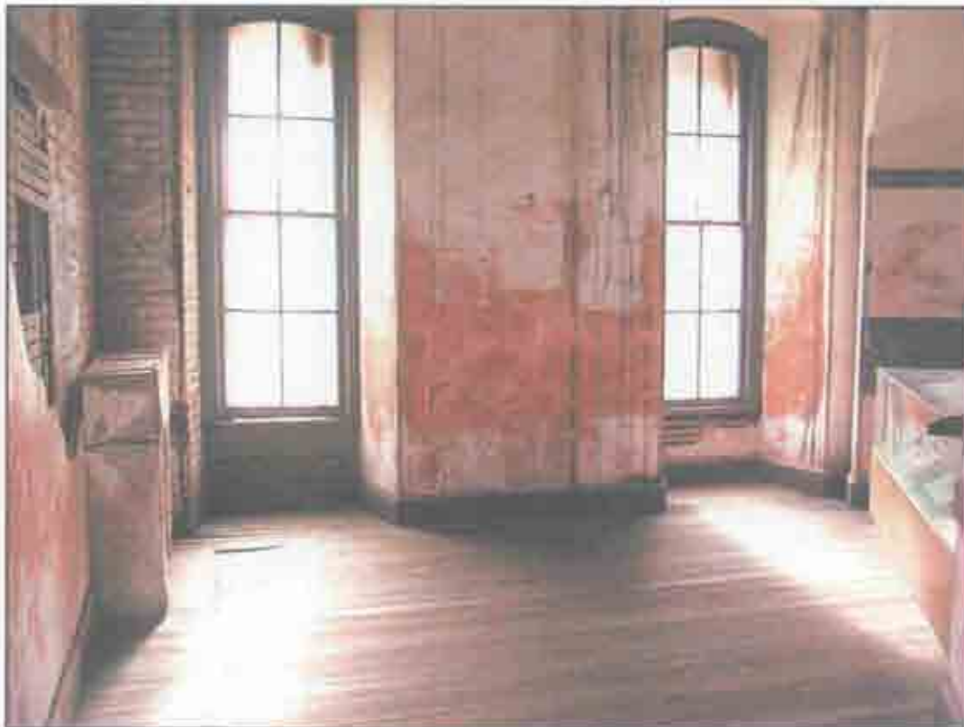
Condition Photo 23: Stained plaster at Casemate 81. (Courtesy of ARG, 2003)
