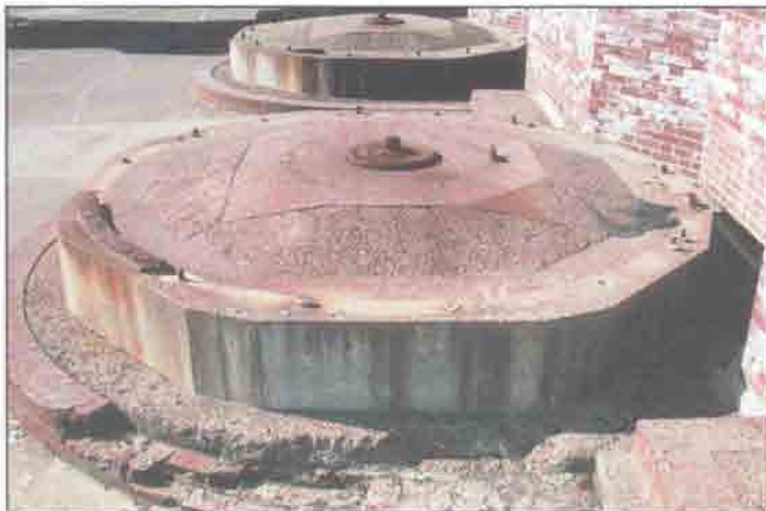
Condition Photo 8: Gun Emplacement No. 104; Open joints, spalled and missing bricks at the gun emplacements. Metal attachments are improperly sealed and are corroding and staining the concrete and granite materials. (Courtesy of ARG, 2003)
