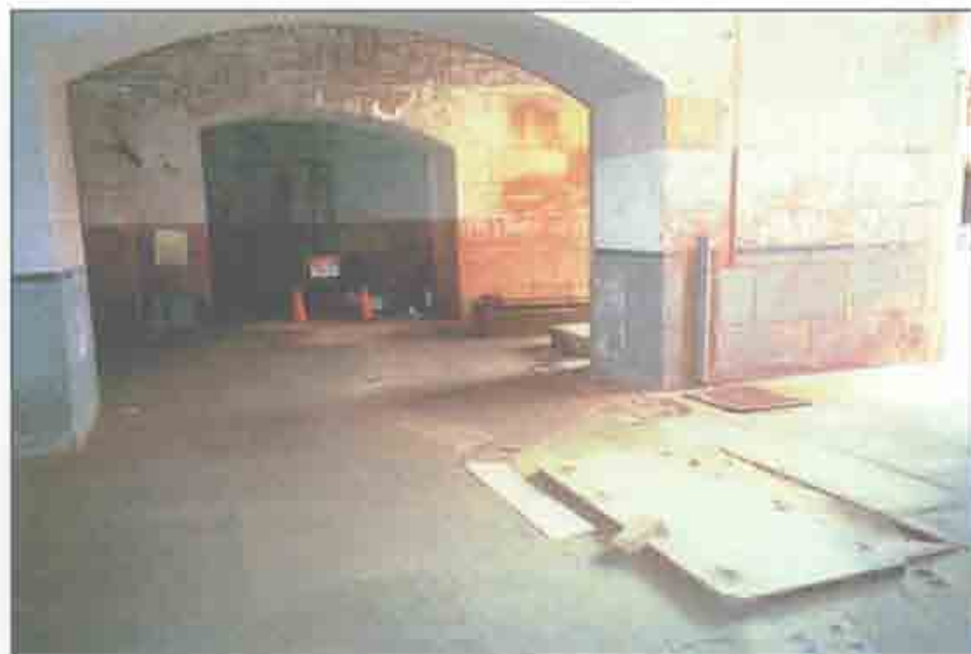
Condition Photo 19: Casemate 34: Uneven surfaces, open holes and potential tripping hazards. (Courtesy of ARG, 2003)
