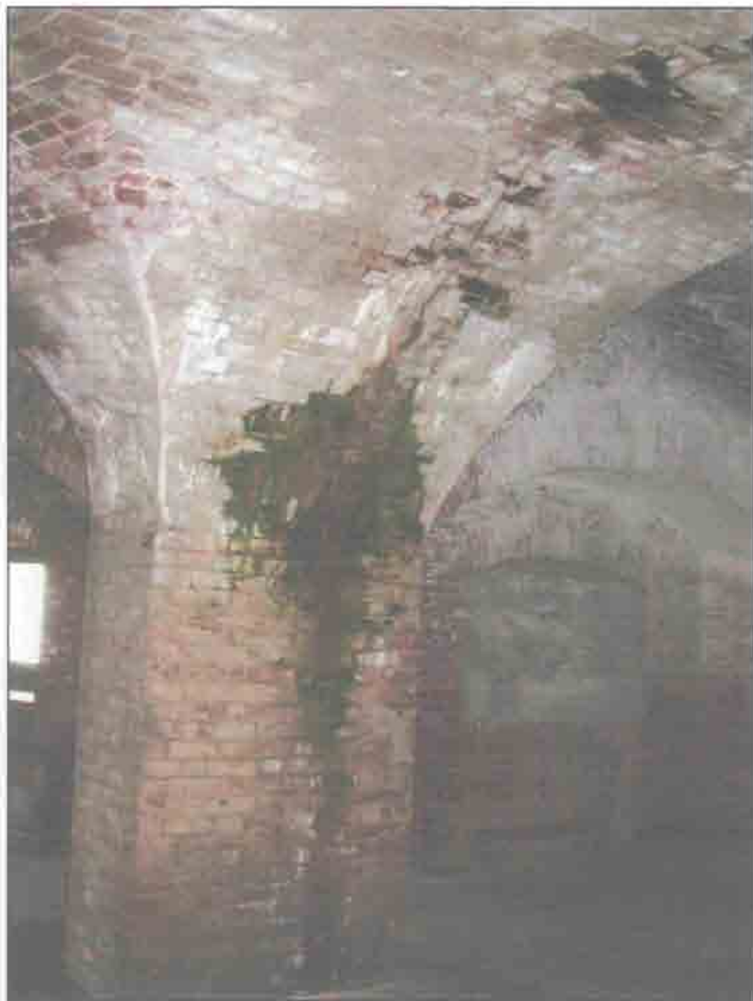
Condition Photo 17: Casemate 68A- Third Tier; Crack spanning the arch of a casemate, typical at the intersection of the east bastion and arch of the adjacent walkway. Extensive water damage, biological growth and efflorescence of masonry. (Courtesy of ARG, 2003)
