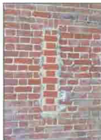
Former rifle slit on south flank filled in with brick. (Jane Lehman, 2005)
