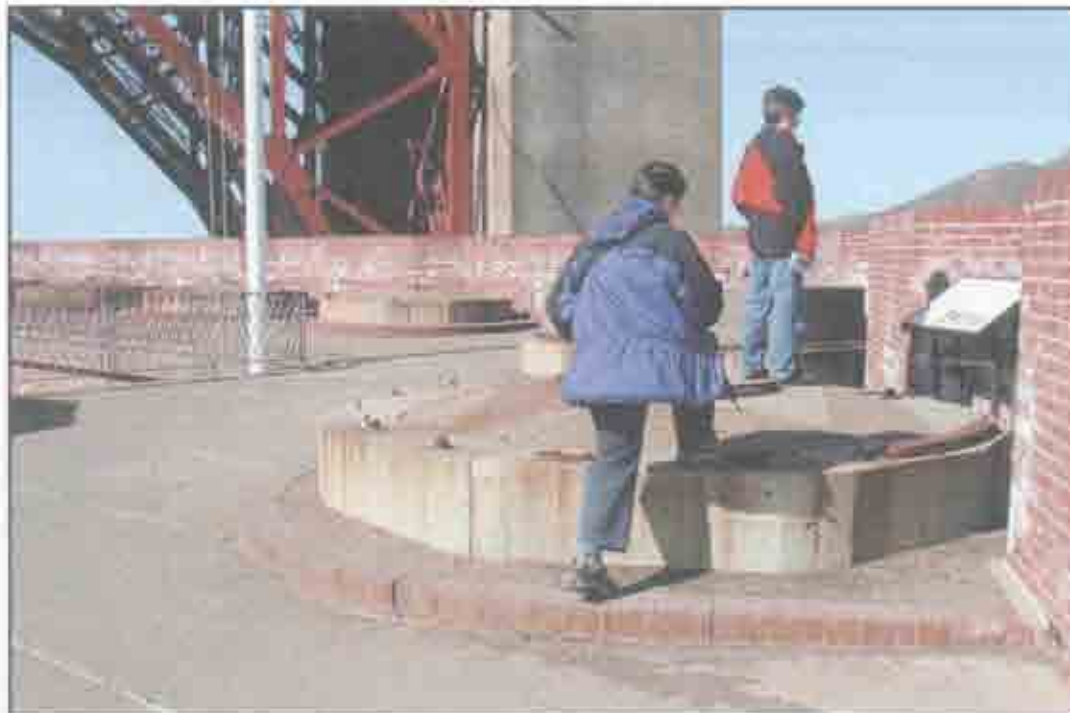
Condition Photo 5: Gun Emplacement 97; Efflorescence occurring on the brick parapet wall surface. (Courtesy of ARG, 2003)
