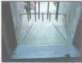
The outline of the former rifle slit is visible in all the window sills along the southwest gorge elevation. (Jane Lehman, 2005)
