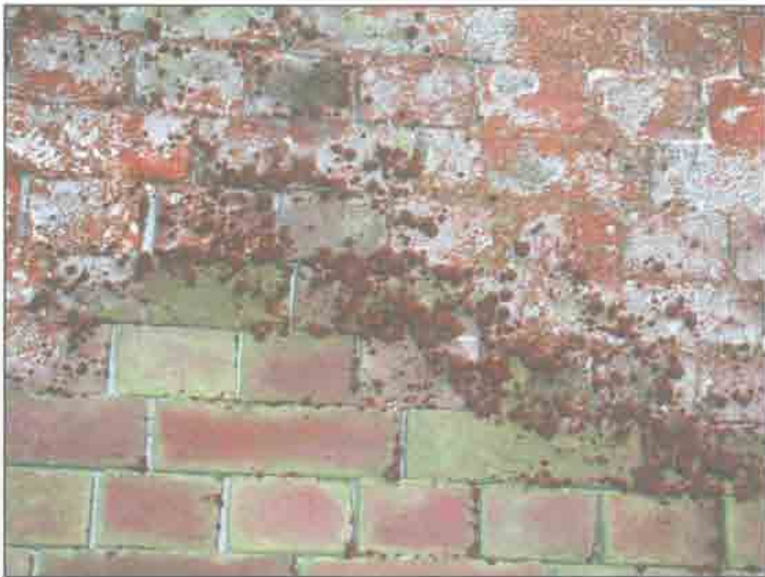
Condition Photo 4: Casemate 100; Biological growth and salts on masonry surface. (Courtesy of ARG, 2003)
