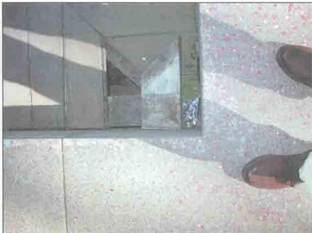
Condition Photo 14: Wood Walkway – Barrette Tier by Stair 1; Components are not properly fastened at wood walkway. (Courtesy of ARG, 2003)
