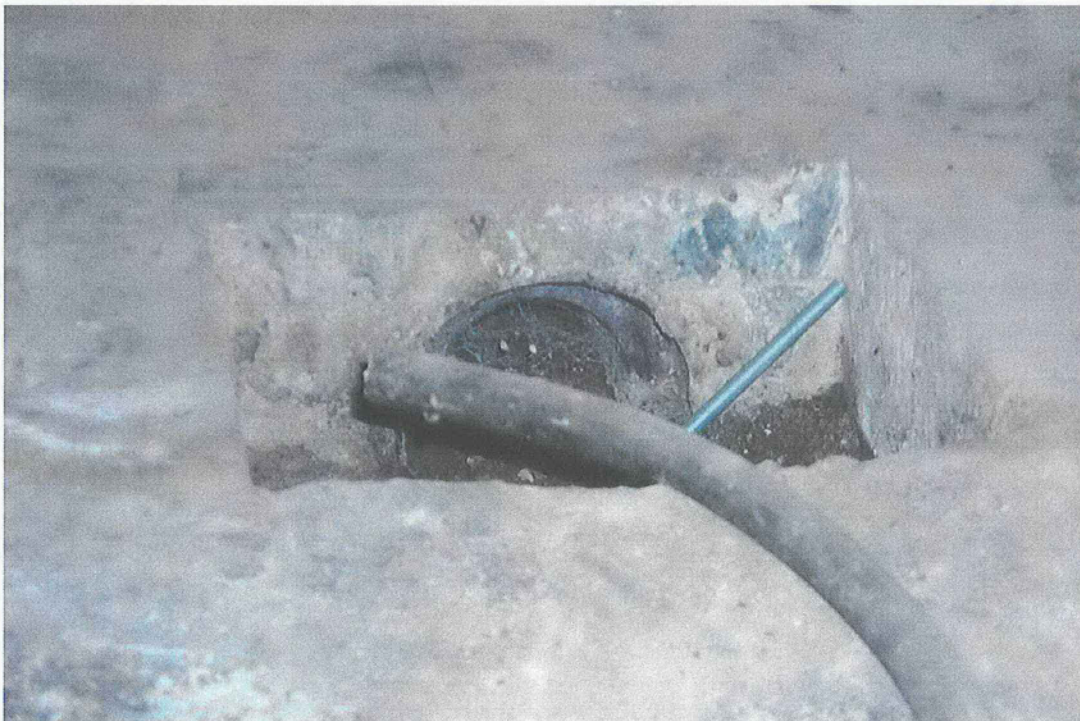
Wright Hall south plenum, drain (QE\A 2000)
