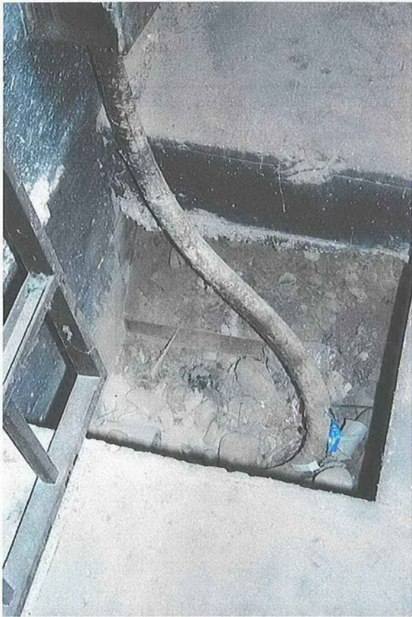
Wright Hall north plenum (QE\A 2000)
