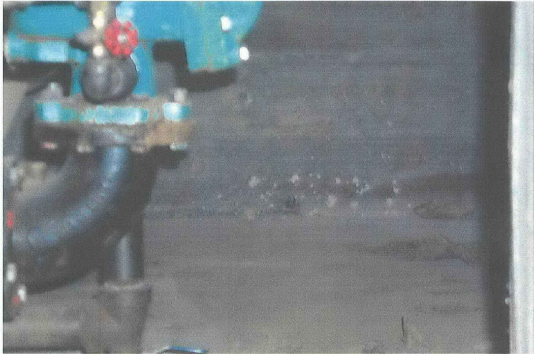
Wright Hall east plenum, south end (QE\A 2000)
