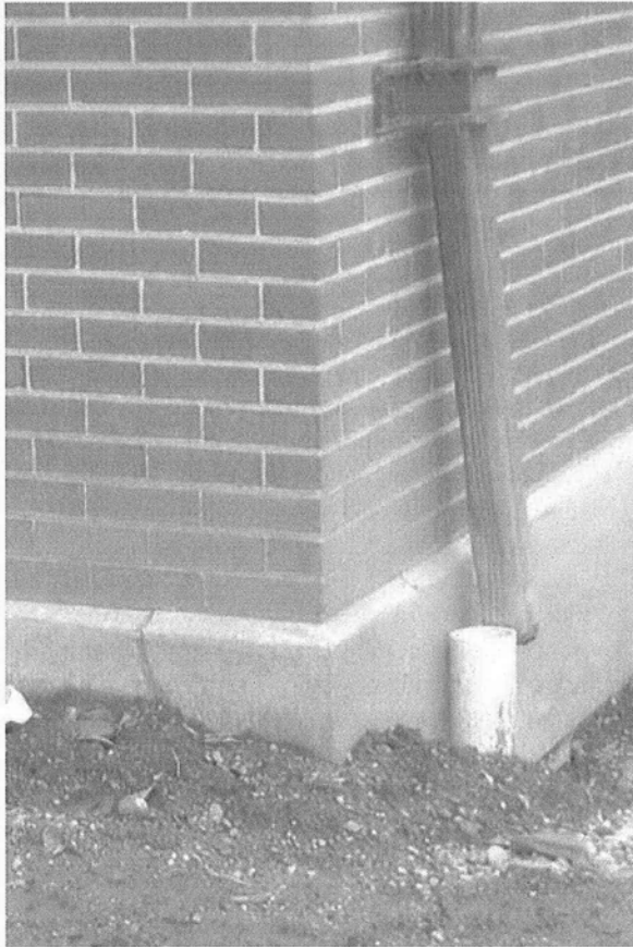
Figure 30: Evidence of cracking at floor on exterior
