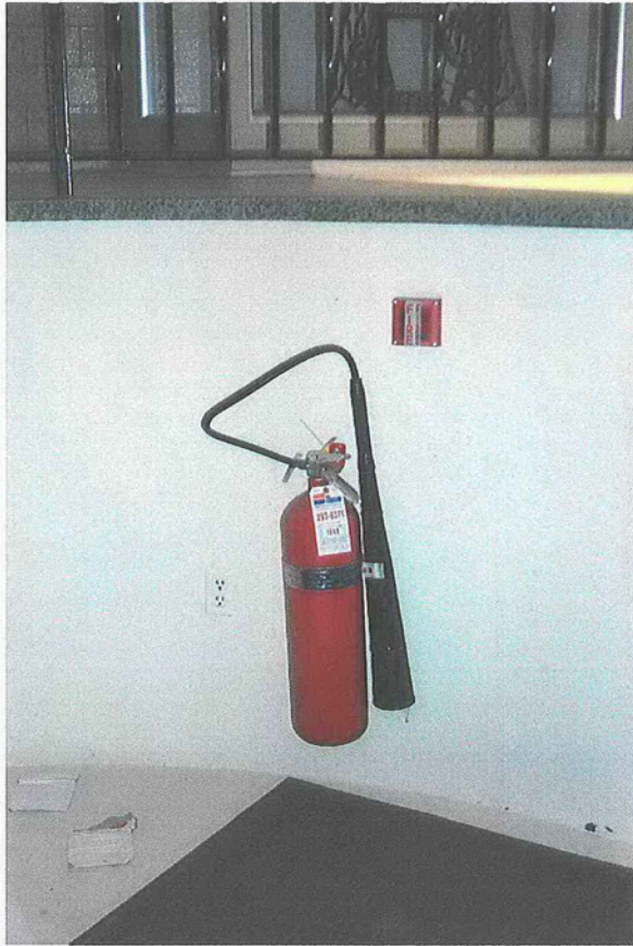
Wright Hall interior, "pit" fire extinguisher (QE|A 2000)
