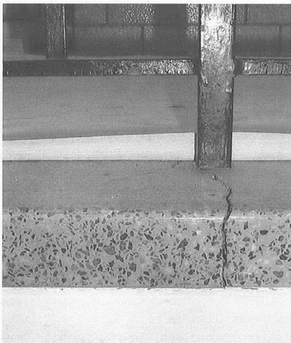
Figure 29: Crack in terrazzo floor.
