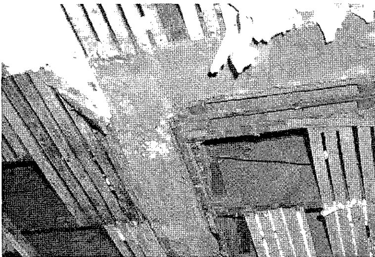
Figure 18 Apparent concrete infill at west side of third floor structure; note that concrete cuts across joist spans with no obvious support (photo 3:16, Fitzpatrick Structural Engineering, P.C., October, 1996)
