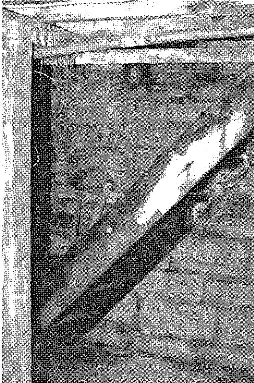
Figure 7 Stair remnant at middle basement south wall (photo 2:19, Fitzpatrick Structural Engineering, P.C., October, 1996)
