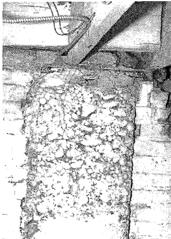
Figure 3 West interior basement wall, first concrete column from the north supporting steel column above; note extensive honeycombing (photo 2:27, Fitzpatrick Structural Engineering, P.C., October, 1996)
