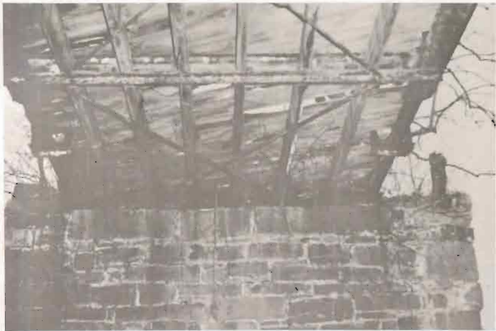
XVI. Iron Bridge at White's Ferry, built in 1876. Photograph from files C&O Canal National Monument.
